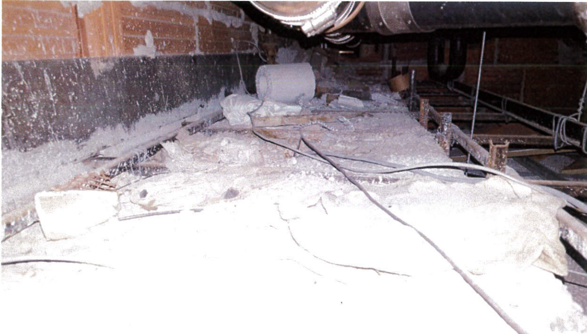
Photo 5: Asbestos containing pipe insulation debris above the solid ceiling in Room 128 at the M-59 Building
