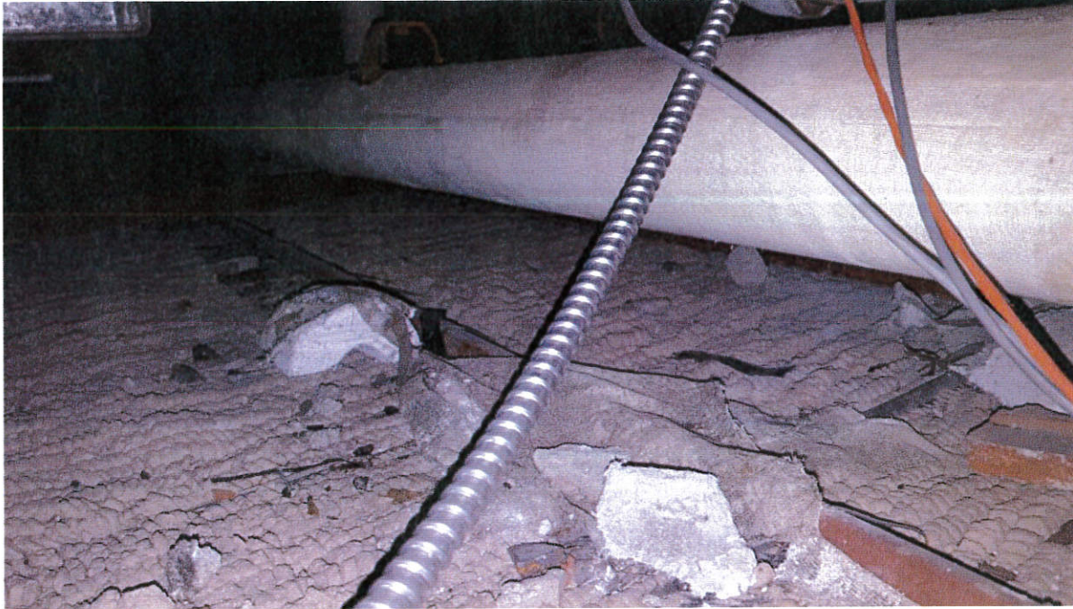
Photo 3: Asbestos containing pipe insulation debris above the solid ceiling in Room 115 at the M-59 Building
