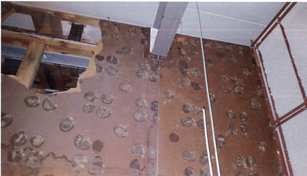
Photo 2: Suspected asbestos containing remnant mastic pucks above Room 271 solid ceiling at the M-2 Building
