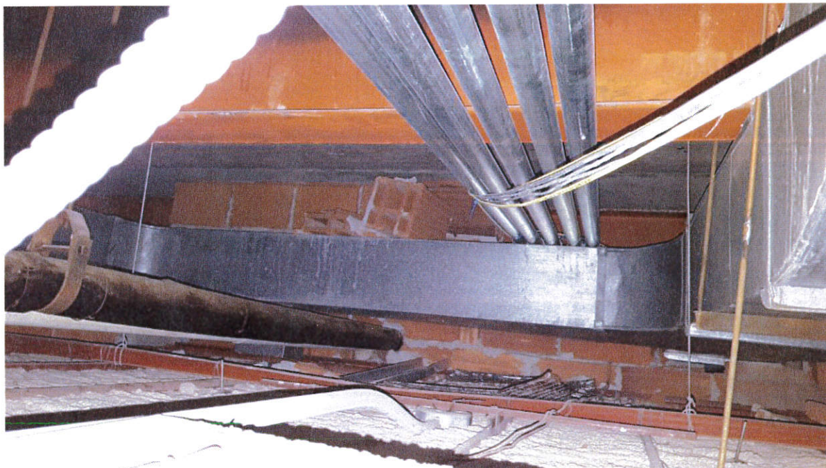
Photo 4: Loose terracotta bricks on top of duct work pose a risk to potential workers removing the duct work.
