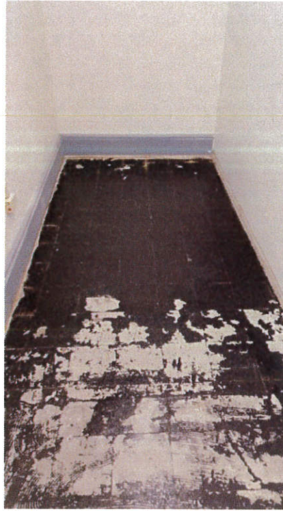
Photo 1: Asbestos-containing remnant mastic and floor levelling compound in Room 133 at the M-2 Building.
