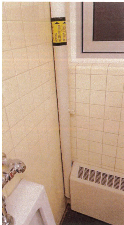
Photo 6: Good condition Mag-block pipe insulation feeding a radiant heater.
