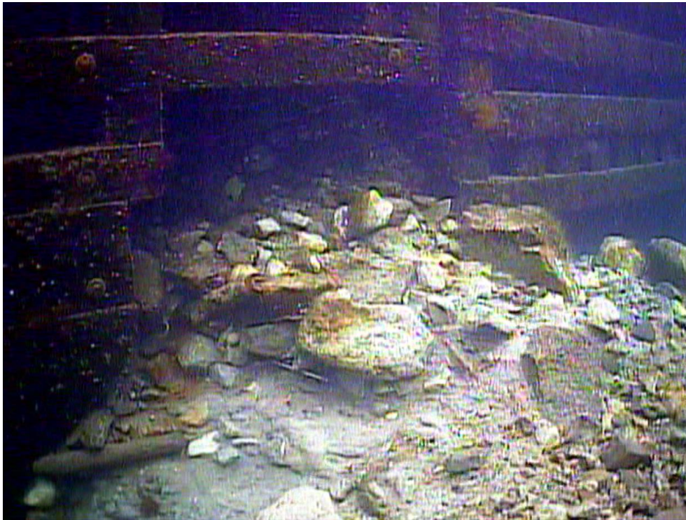
Photo #4 – a area where the crib was stepped up appears to have ballast spilled
