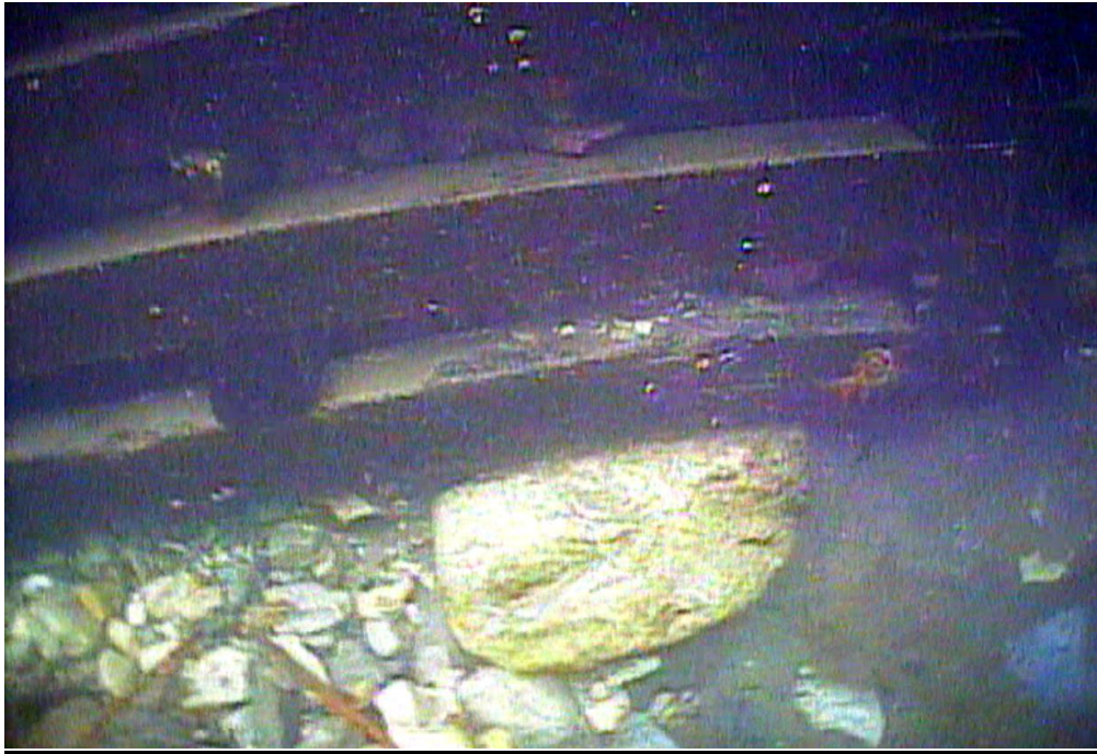
Photo #9 – Crib sitting on wharf, cracked timber.
