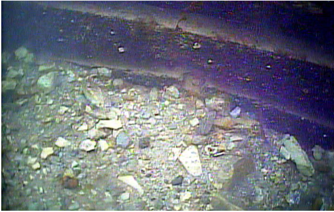
Photo #7 – Cracked bottom timber of crib
