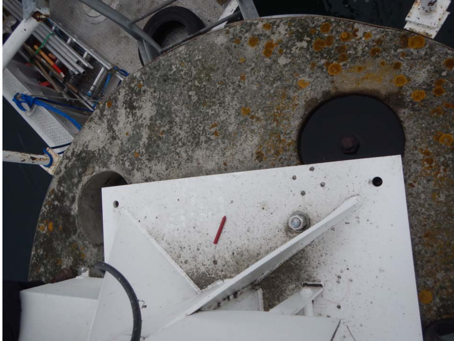
Existing pier top and soil anchors. Removals must preserve integrity of anchors
