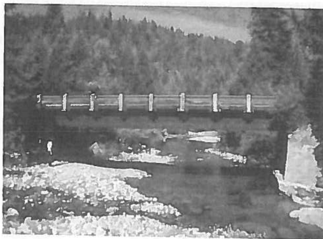
Figure 4.2 Oilborne preservatives are often used for treatment of glulam beams, such as in this bridge (Lebow and Tippie, 2001).
