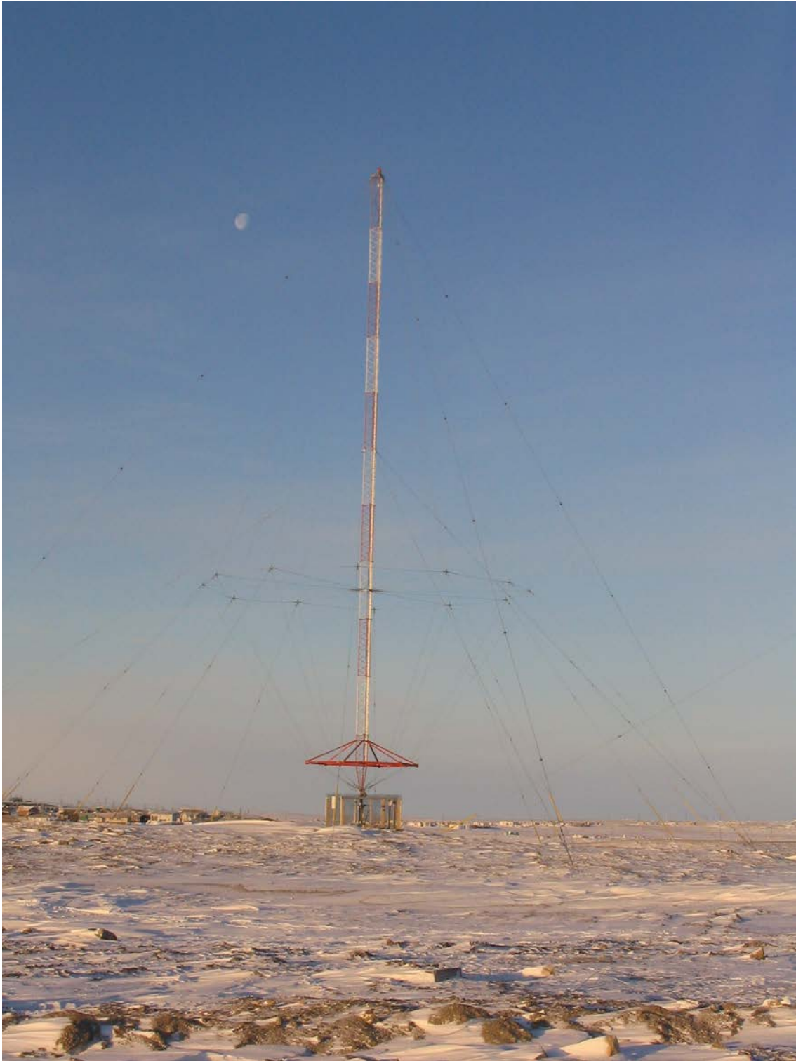
Figure 8: M19 Tower Paint touch up required
