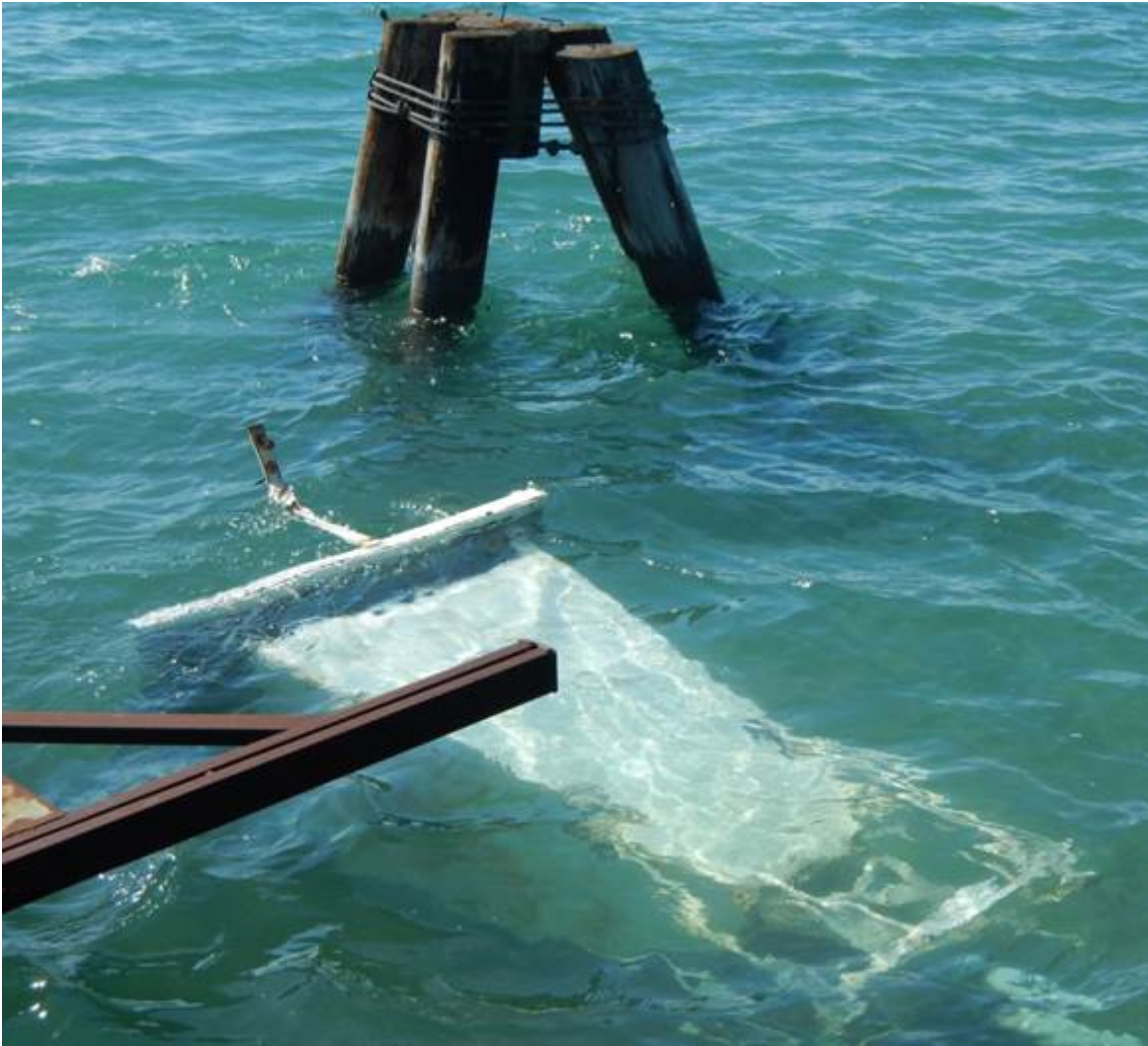
Figure 3: Detached and Sunken naavid (has been removed by CCG)
