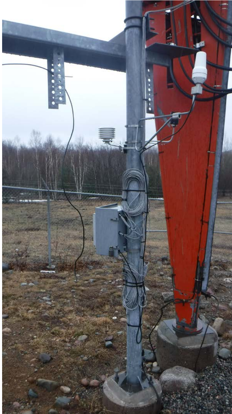
Figure 19: Waveguide bridge post adjacent to the tower with mounted equipment (not to be demolished).
