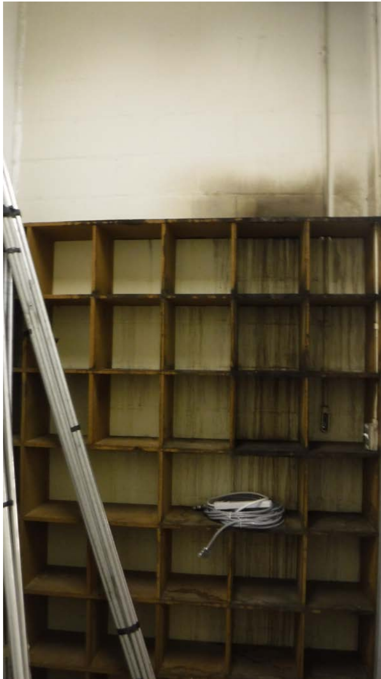
Figure 9: Mould on shelves (to be demolished). See Hazardous Materials Survey in Appendix B4 for removal procedure.
