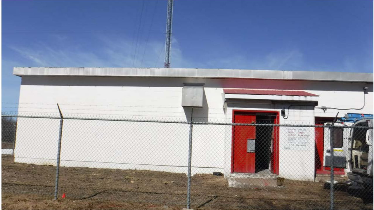
Figure 3: Old radio equipment building facing [East] and entrance porch (to be demolished)
