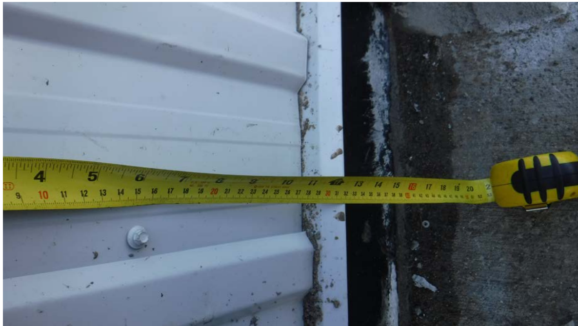
Figure 22: Approximate measurement from concrete pad to floor level in door opening. To be confirmed by contractor.
