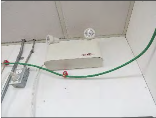
Photo 11: Emergency light, location 1.
