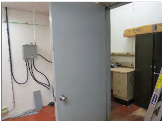
Photo 10: Grey paint on wood door, lead containing.
