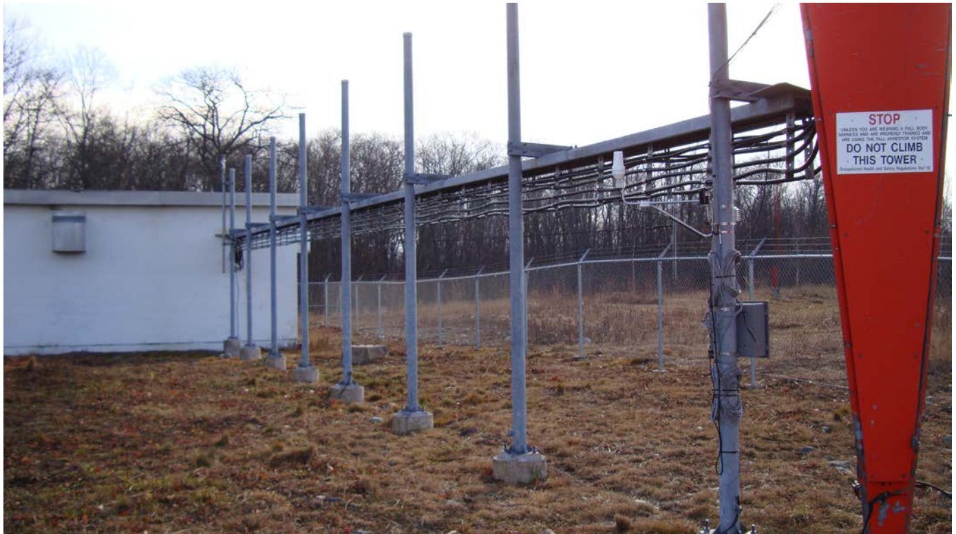
Figure 18: Waveguide bridge to be demolished. The post adjacent to the tower containing equipment is not to be demolished.
