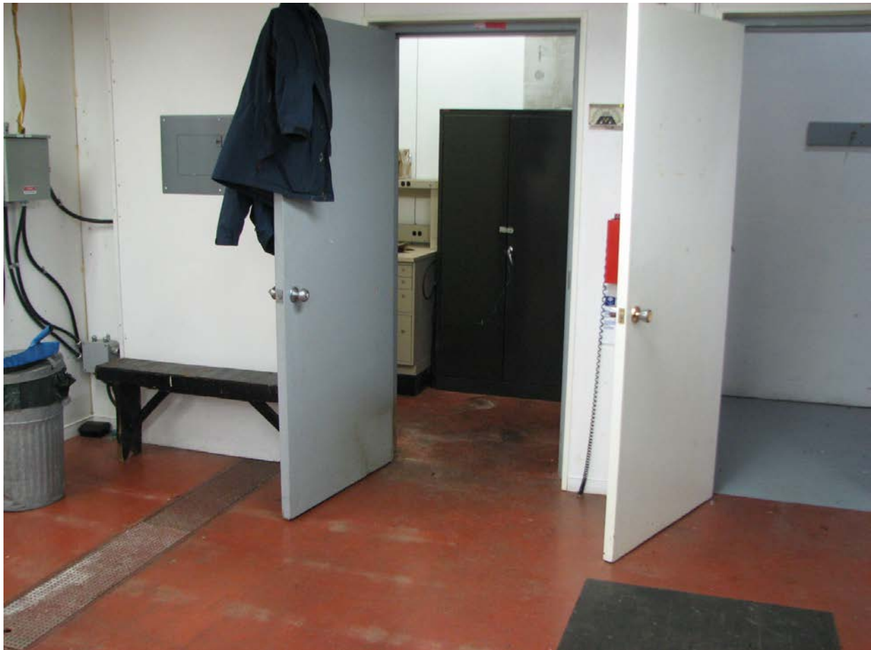
Figure 15: grey door contains lead paint.
