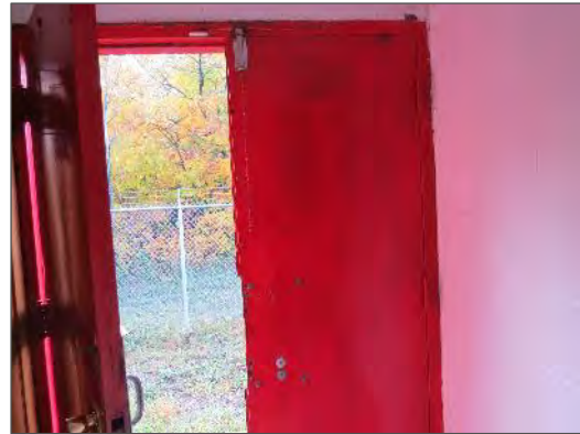
Photo 7: Red paint on metal door, lead-containing.
