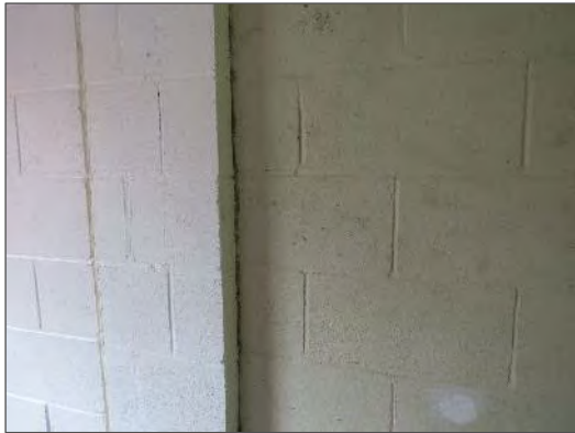
Photo 6: Beige on concrete block, insignificant lead concentration.
