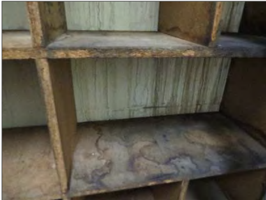
Photo 14: Water staining and mould growth on the OSB shelving in Location 3.
