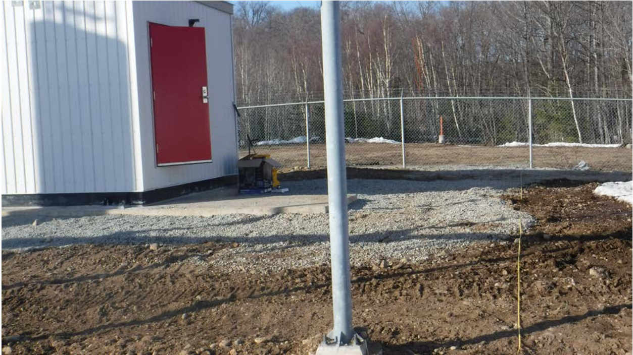
Figure 21: One of two doors of new building. Notice concrete pad extending in front of door.
