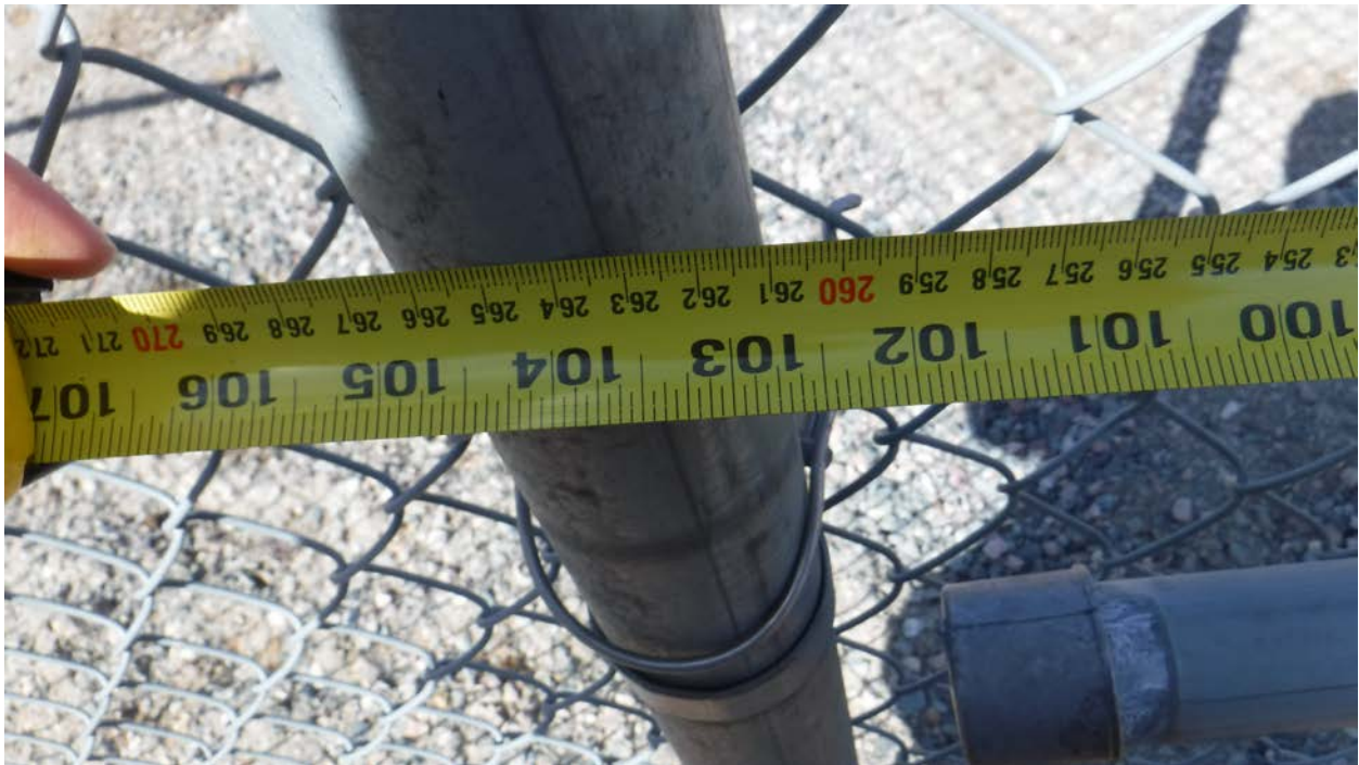
Figure 16: Broken brace. To be repaired.
