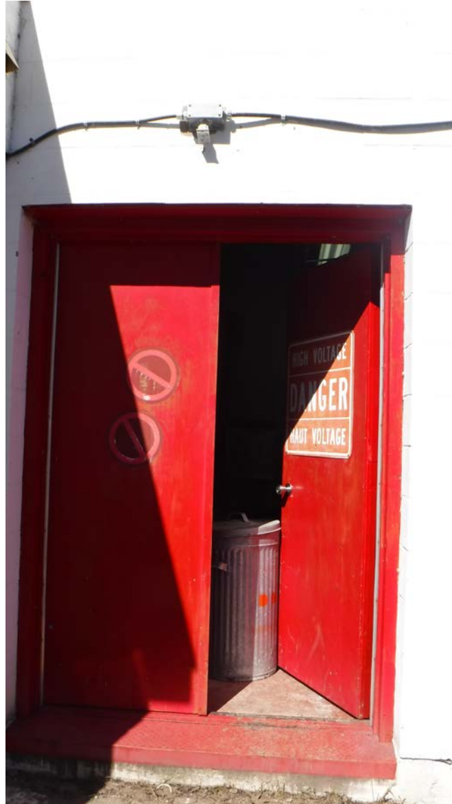
Figure 14: One of the three lead paint containing exterior doors of the building (to be demolished).
