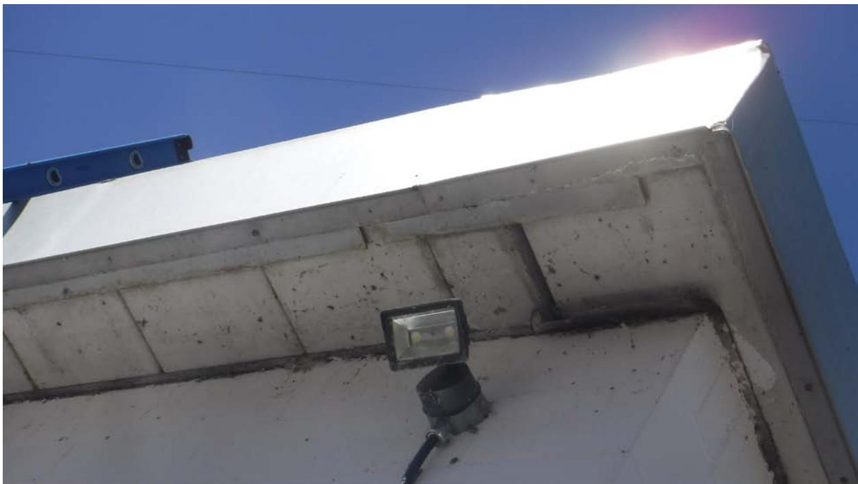
Figure 11: Precast concrete panels on the roof of the building (to be demolished)
