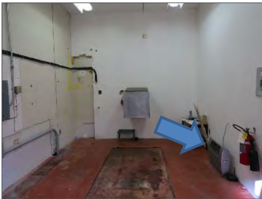
Photo1: Electric baseboard radiators, uninsulated.
