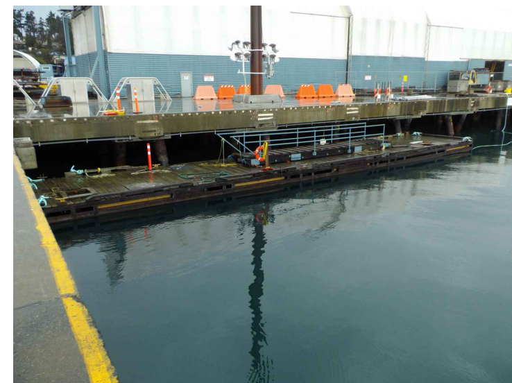
PHOTO C47-09 TUG BOAT WHARF AND SOUTH FACE OF PILED DECK - NOTE REINSTATED HIGH MAST LIGHT
