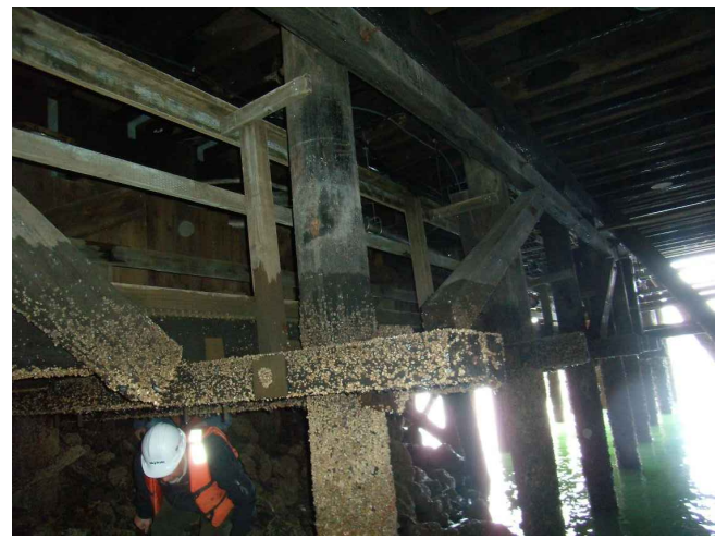
PHOTO C15-05 TIMBER PILED JETTY – VIEW AT EAST END FIRE STOP WALL AND CATWALK (BEFORE SHEET PILE PERIMETER WALL WAS INSTALLED)
