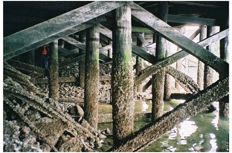
PHOTO C15-04 TIMBER PILED JETTY – TYPICAL VIEW LOOKING EAST (BEFORE SHEET PILE PERIMETER WALL WAS INSTALLED)
