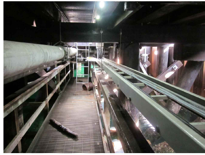
PHOTO C16-02 SOUTH JETTY CATWALK WITH MECHANICAL AND ELECTRICAL SERVICES
