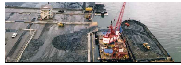
PHOTO 1: EXAMPLE OF OFFLOADING OPERATIONAL CONTROLS
