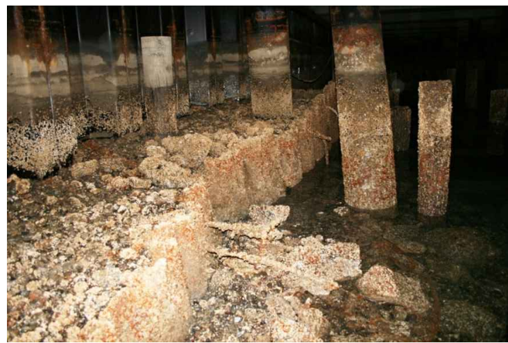
PHOTO C14-07 REMNANTS OF LOWER SHEET PILING - NOTE SHEET PILED BULKHEAD IN BACKGROUND
