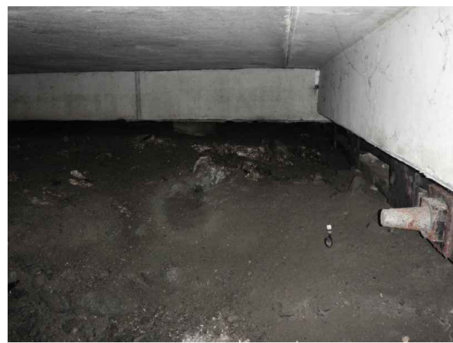
PHOTO C17-08 FORESHORE FILL MOUND UNDER STEEL PILED CONCRETE DECK – NOTE STEEL WALER AT RIGHT AND SEVERELY LIMITED HEADROOM
