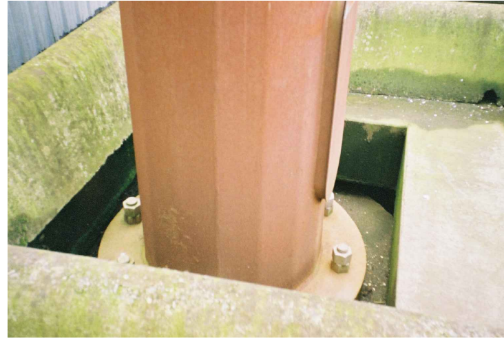
PHOTO C17-02 HIGH MAST LIGHT ABOVE STEEL PILED CONCRETE DECK – NOTE LIMITED SIZE OF DECK OPENING
