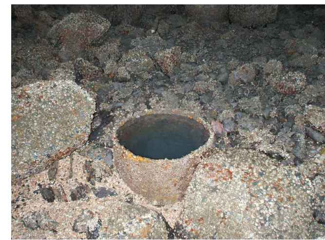
PHOTO C14-09 OPEN STEEL PIPE PILE UNDER STEEL PILED CONCRETE DECK - NOTE SAFETY RISK
