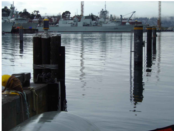
PHOTO C47-04 NAVIGATIONAL DOLPHINS AND CORNER DOLPHIN AT THE NORTHWEST FACE OF THE TIMBER CRIB
