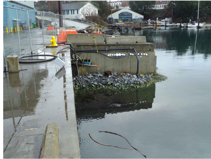
PHOTO C47-02 UTILITIES TERMINATED AND CAPPED AT FACE OF CONCRETE L-WALL - NOTE TEMPORARY ELECTRICAL SERVICE TERMINATED WITH JUNCTION BOX AT DECK LEVEL
