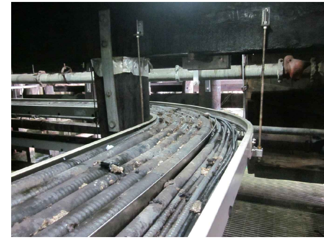
PHOTO C16-03 UNDER-PIER CATWALK - TYPICAL CABLE TRAY
