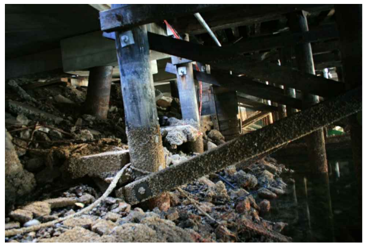
PHOTO C15-06 TIMBER PILED JETTY AT INTERFACE WITH STEEL PILED DECK— NOTE RIPRAP ON FORESHORE AND MISCELLANEOUS CONCRETE FOOTINGS
