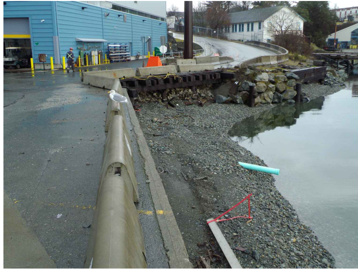
PHOTO C47-01 EAST APPROACH STRUCTURE AND CONCRETE L-WALL - NOTE TIMBER BENT AND PILE CAP
