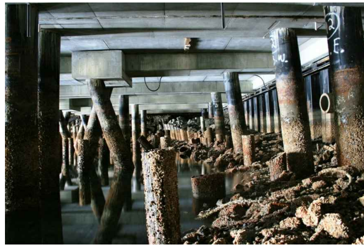
PHOTO C14-04 STEEL PILED CONCRETE DECK LOOKING WEST - NOTE CATHODIC PROTECTION CABLES AT SLAB SOFFIT
