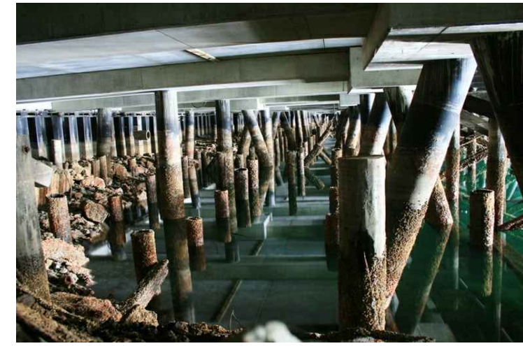
PHOTO C14-03 STEEL PILED CONCRETE DECK LOOKING EAST - NOTE BATTER PILES AND TIMBER PILE REMNANTS
