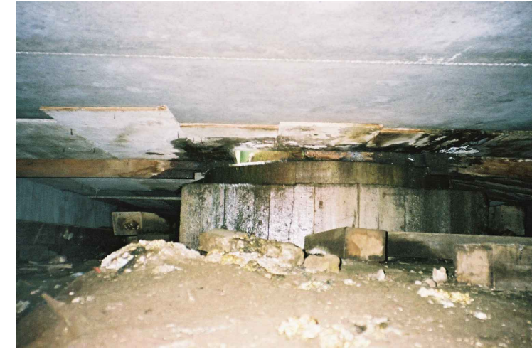
PHOTO C17-03 HIGH MAST LIGHT FOUNDATION UNDER STEEL PILED CONCRETE DECK – NOTE TIMBER FORMS LEFT IN PLACE
