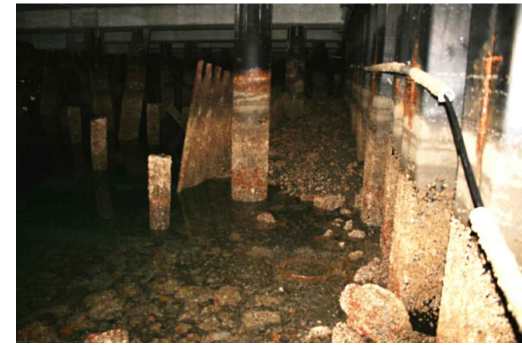
PHOTO C14-06 PAINTED SHEET PILE BULKHEAD - NOTE CATHODIC PROTECTION AND REMNANTS OF LOWER SHEET PILING (TIDE APPROX. EL+1.0M)
