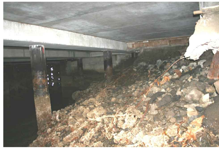
PHOTO C17-05 FORESHORE FILL MOUND UNDER STEEL PILED CRANE PAD – LOOKING NORTHWEST TOWARDS TIMBER CRIB
