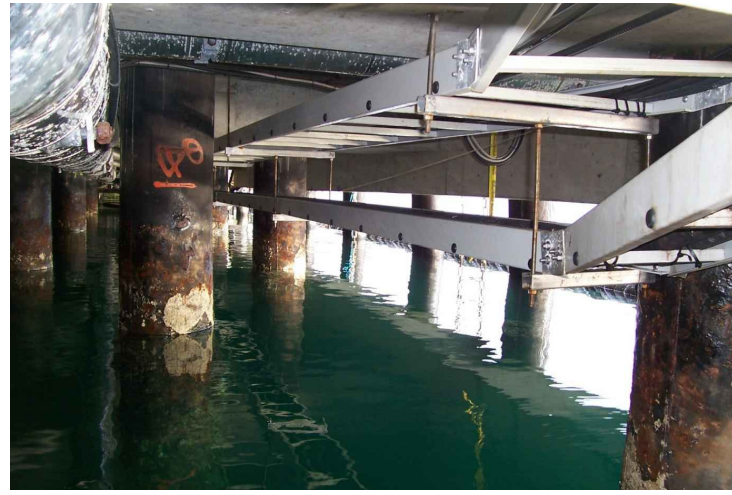
PHOTO C17-01 CABLE TRAY UNDER CONCRETE DECK LOOKING EAST FROM WEST TIMBER PILED JETTY (BEFORE SHEET PILE PERIMETER WALL WAS INSTALLED)
