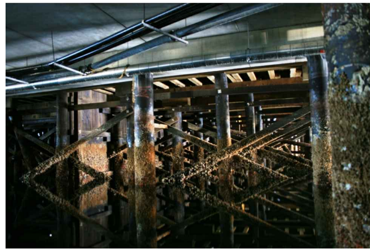
PHOTO C14-05 STEEL PILED CONCRETE DECK NEXT TO TIMBER PILED WEST JETTY - NOTE TIMBER FIRE STOP WALL AND CROSS-BRACING
