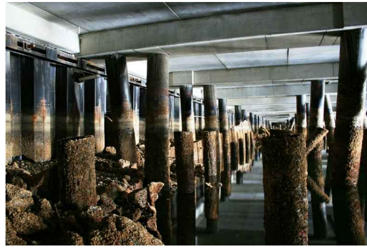
PHOTO C14-02 STEEL PILED CONCRETE DECK LOOKING EAST - NOTE TIMBER PILE REMNANTS AND LOWER SHEET PILING
