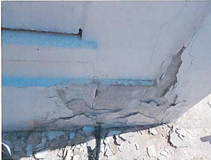
Photo 15 – Southwest Wall – Deteriorated and Cracked Façade and Blocks
