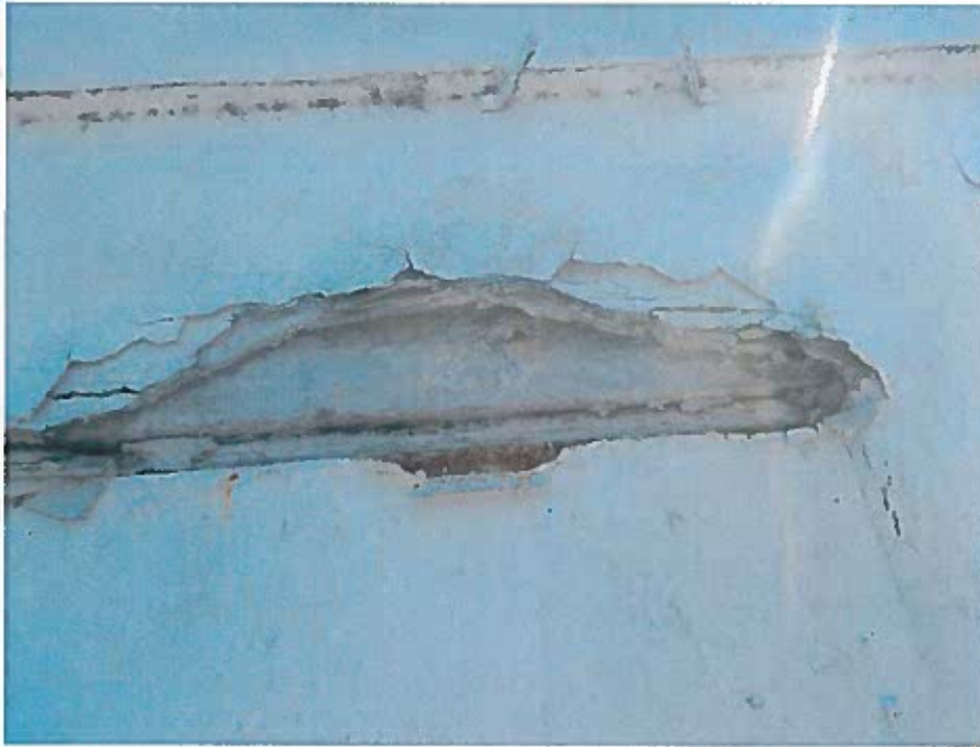
Photo 14 – Southwest Wall – Deterioration at Window Lintel
