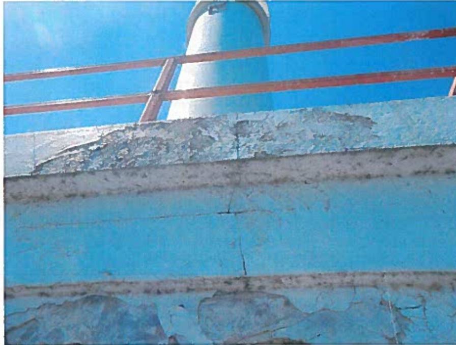
Photo 7 – Northeast Wall – Cracking through Roof Slab and Wall
