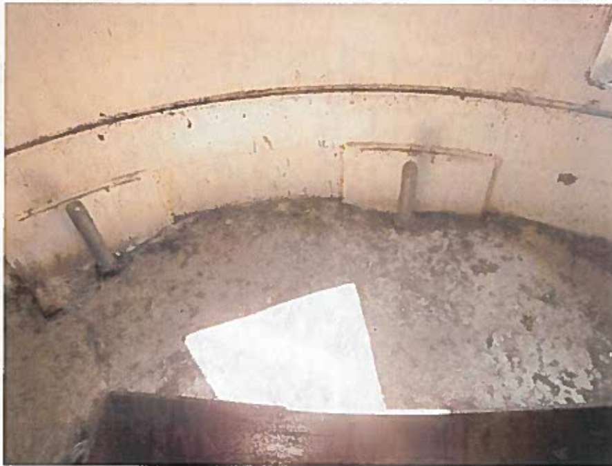
Photo 26 – Typical Tower Connection to Building Roof
