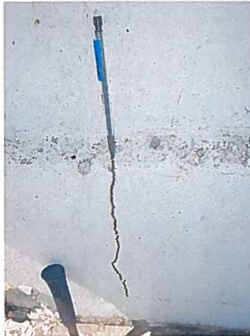
Photo 8 – Northeast Wall – Crack in Wall Down to Foundation
