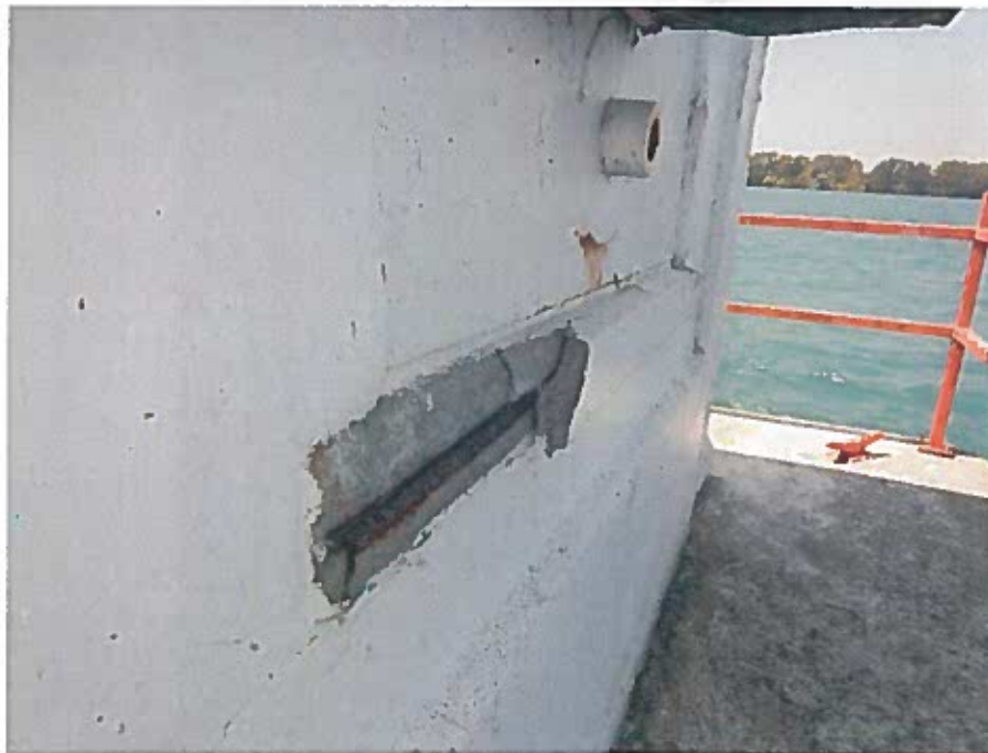
Photo 10 – Northwest Wall – Damaged Window Sill
