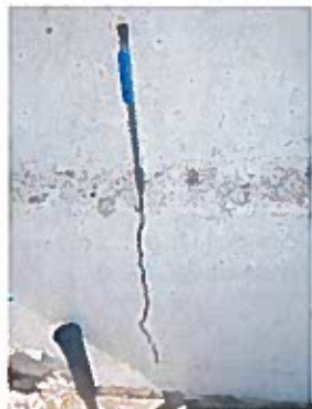
Photo 2.3 – Crack in Building Wall to Foundation
