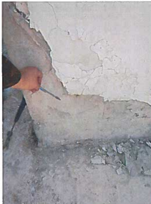
Photo 12 – Southwest Wall – Delaminated Patch
