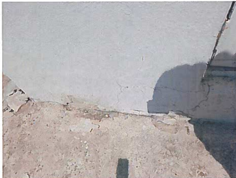
Photo 16 – Southeast Wall – Cracking through Foundation to Crib Cap
