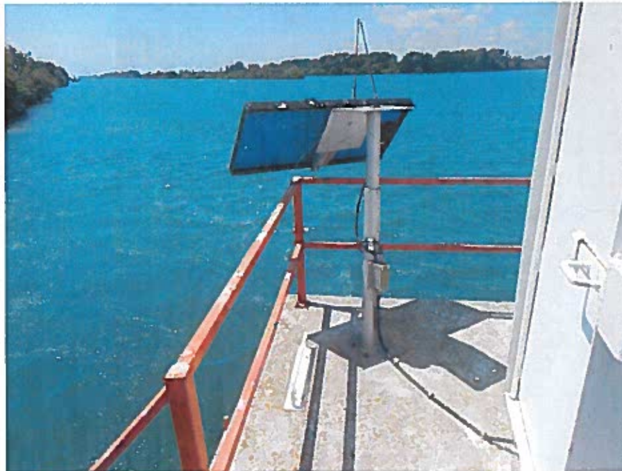
Photo 24 – Solar Panel on South Corner of Building Roof
