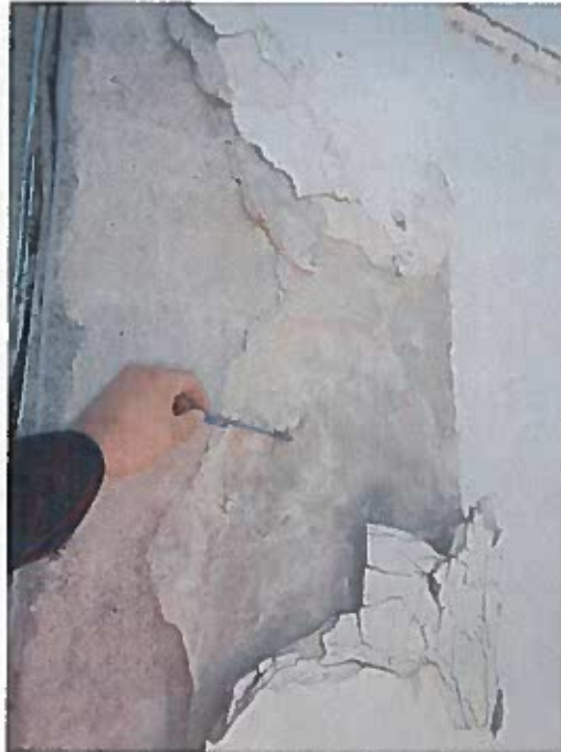
Photo 13 – Southwest Wall – Delaminated Façade
