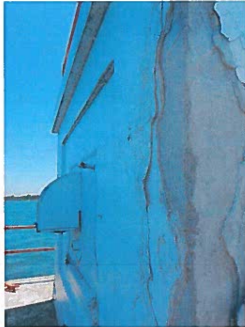
Photo 11 – Northwest/Southwest Wall – Delaminated and Spalling Façade
