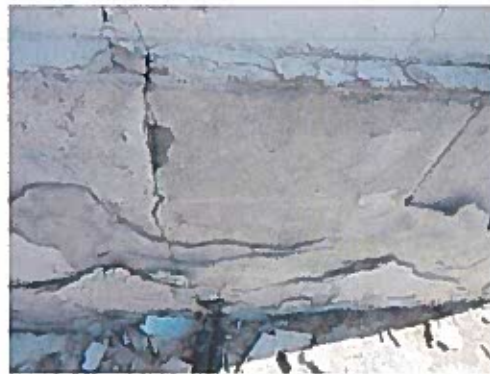
Photo 2.2 – Deteriorated and Cracked Wall
