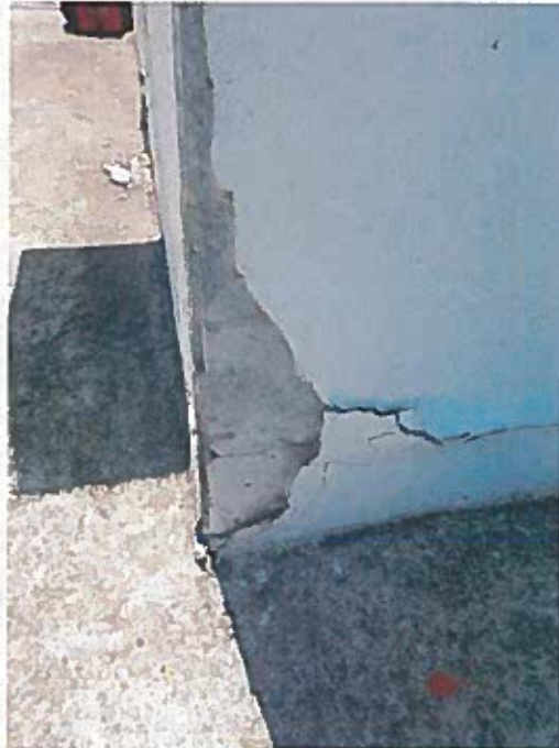
Photo 9 – Northwest Wall – Deteriorated Façade, Cracked and Spalled Blocks
