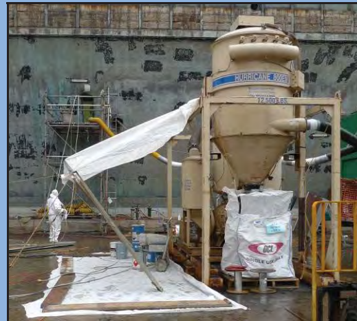
All hazardous materials must be stored in appropriate containment and away from tunnel drain system.
