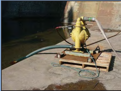
The sill diversion pump removes clean saltwater from the pool at the front of Section 1 (moon pool) and discharges to the tunnel drains through a hard pipe on the dock wall.
