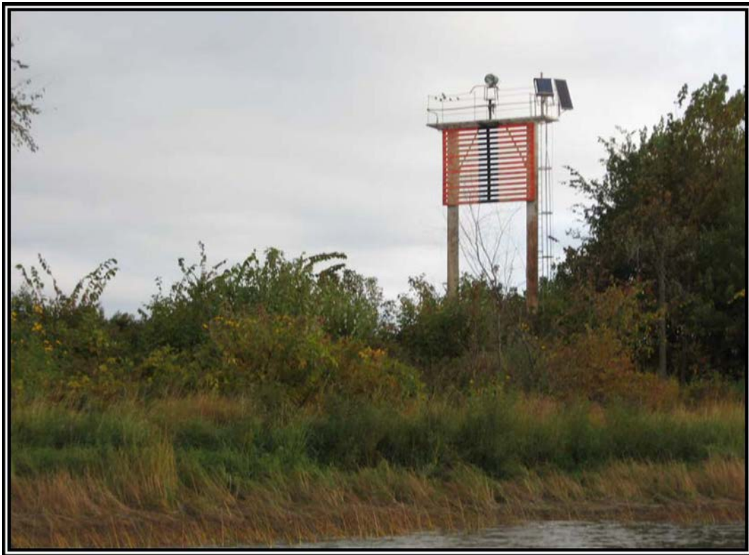
Photograph no. 1: Northbound view of the front range light (FRL) for navigation on Île Bouchard.
