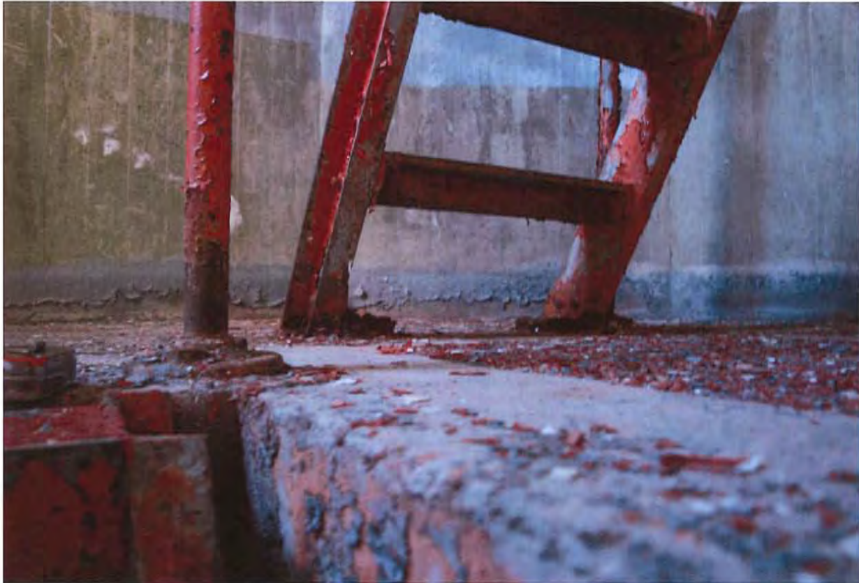
Typical condition of ladders and railings at supports. Peeling paint, local corrosion.
