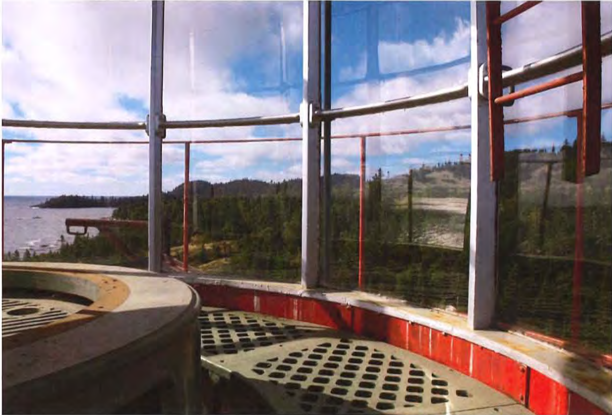
Lantern room: Metal-plate wall, open-grate cast iron upper floor. Condition generally satisfactory.
