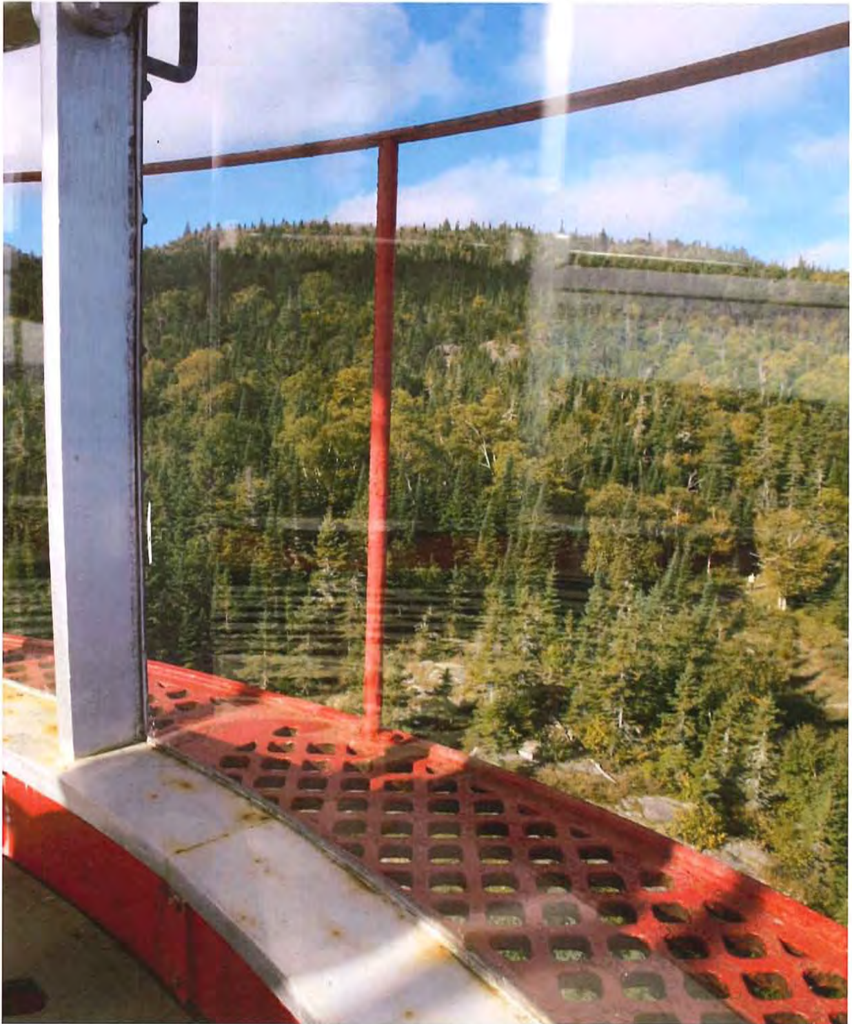
Exterior platform: Open-grate cast-iron with steel pipe railing. Local corrosion.
