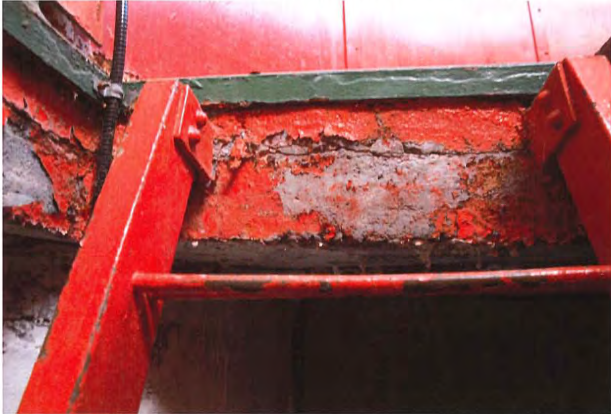
Ladder opening through top floor. Horizontal crack in slab is probably same crack visible at outside edge of exterior concrete platform. See P6.
