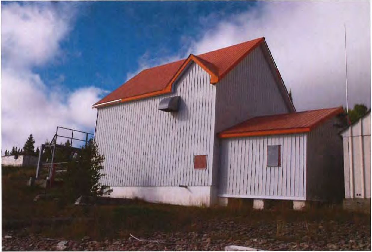
Generator Building & Annex. Metal cladding in good condition, several fascia pieces missing.
