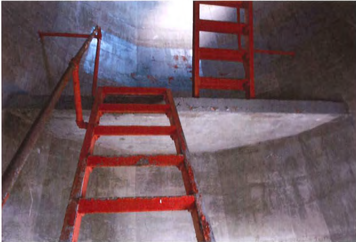
Typical ladders, pipe railings, concrete landing. Note walls generally in good condition.
