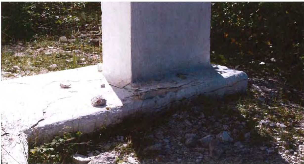
Concrete cracking and spalling at base of buttress.
