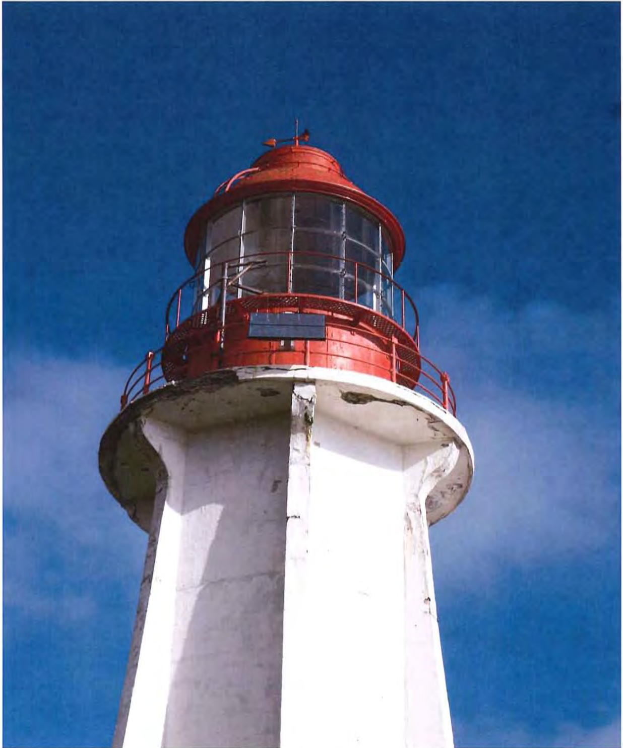
Concrete spalling at exterior concrete platform. Note horizontal crack at edge of slab. See P8.
