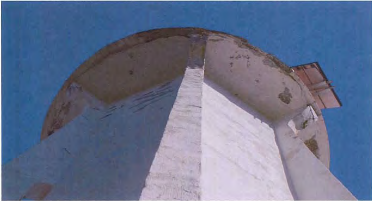
Concrete spalling on wall face and at buttress flares.
