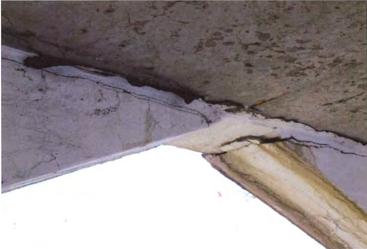
Balcony slab. Cracking at column haunches. Paint fully peeled-off slab underside.
