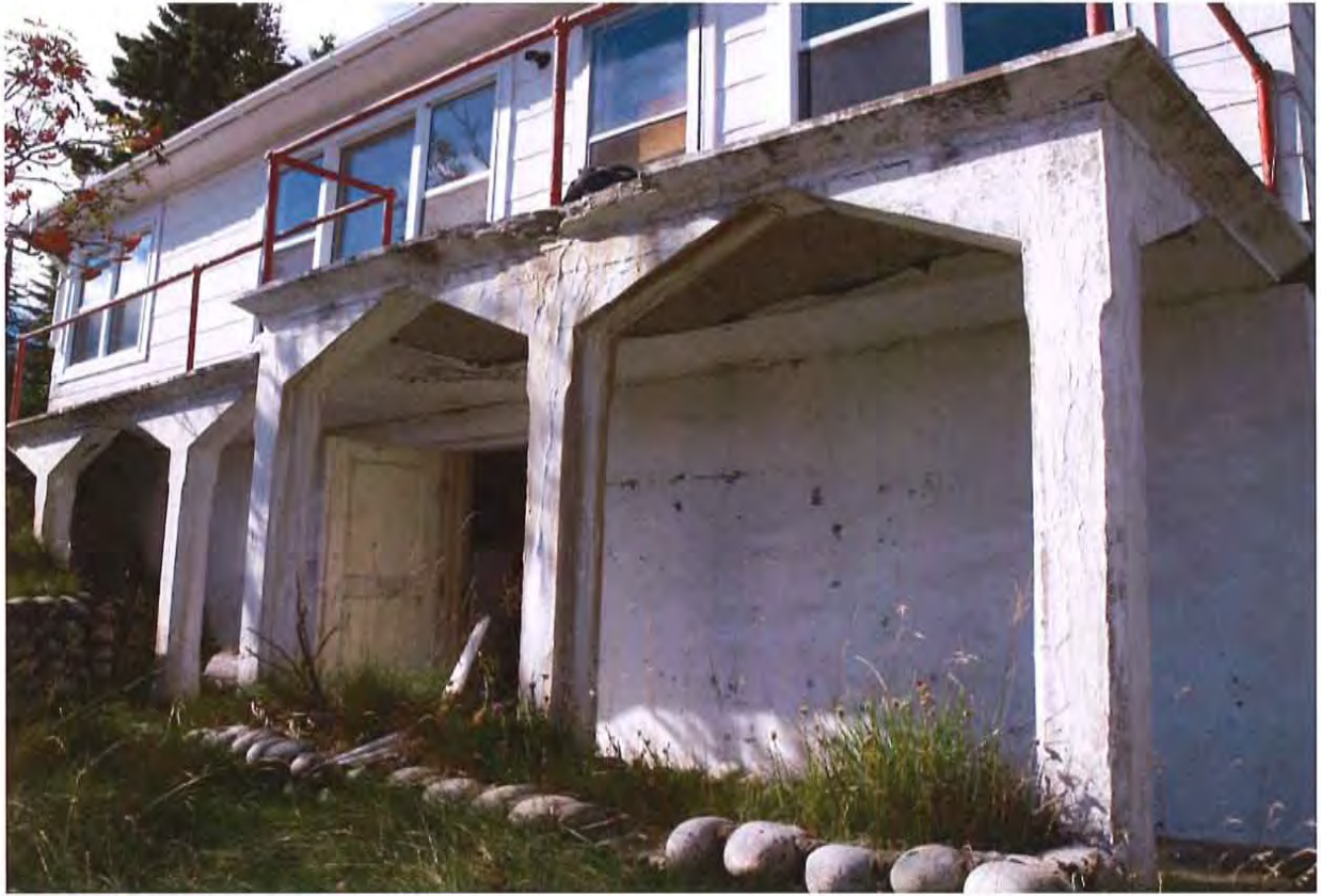
Significant spalling of slab edge. Loss of integrity at base of railing post. Peeling paint on slab soffit.
