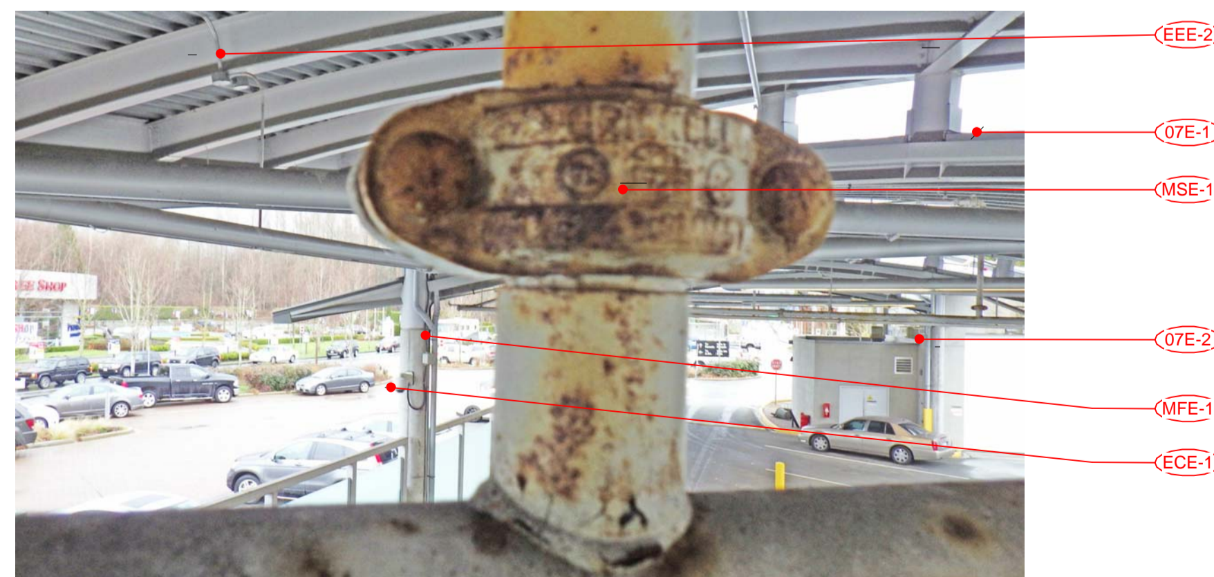
3 SIA CANOPY FIRE PROTECTION A305 TYPICAL EXTG CONDITION OF FIRE PROTECTION PIPING
