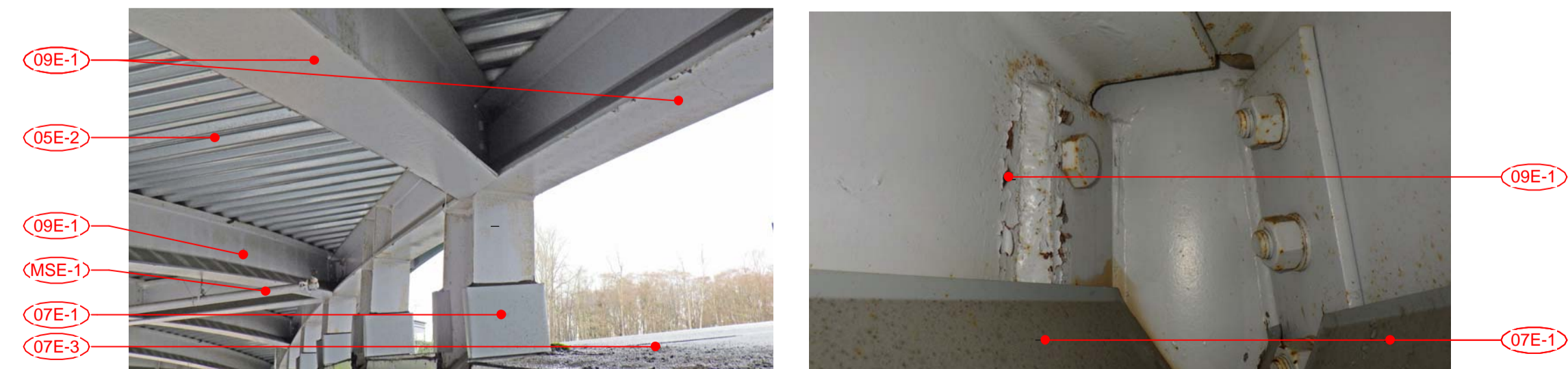
6 SIA CANOPY STEEL STRUCTURE & CONNECTIONS A305 TYPICAL EXTG CONDITION OF STEEL BEAMS, CONNECTIONS, FLASHING AND ROOF MEMBRANE
