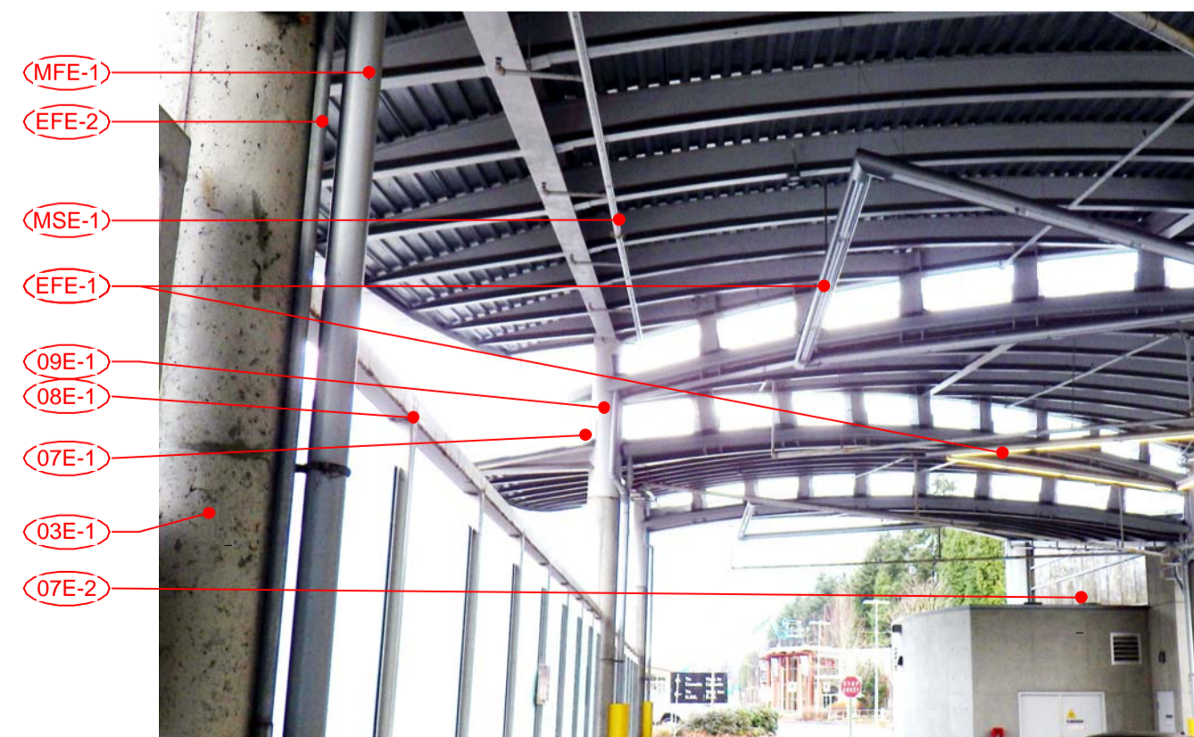
8 TIA - SOUTH ELEVATION A306 TYPICAL EXTG CONDITION OF STRUCTURAL STEEL AND PEDESTRIAN SCREEN
