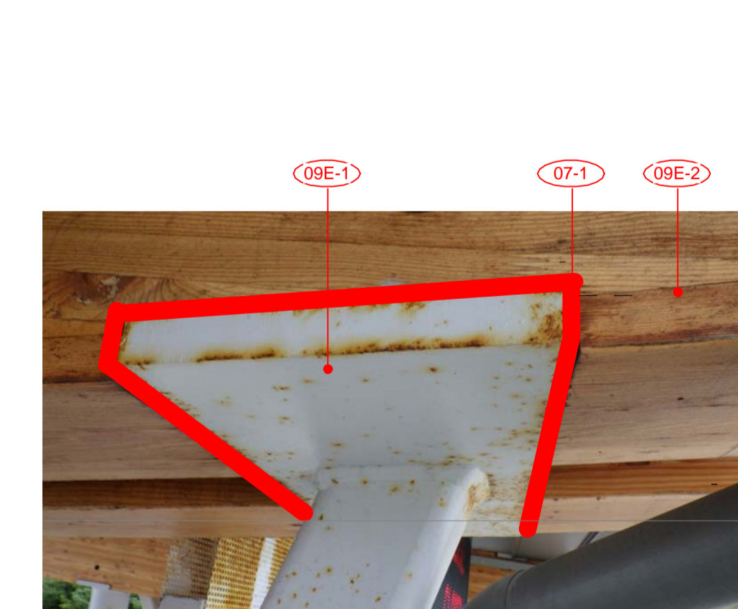
6 STEEL COLUMN TO GLULAM BEAM A300 TYPICAL EXTG CONDITION OF STEEL AND NEW SEALANT APPLICATION TO STEEL BRACE AT GLULAM BEAM
