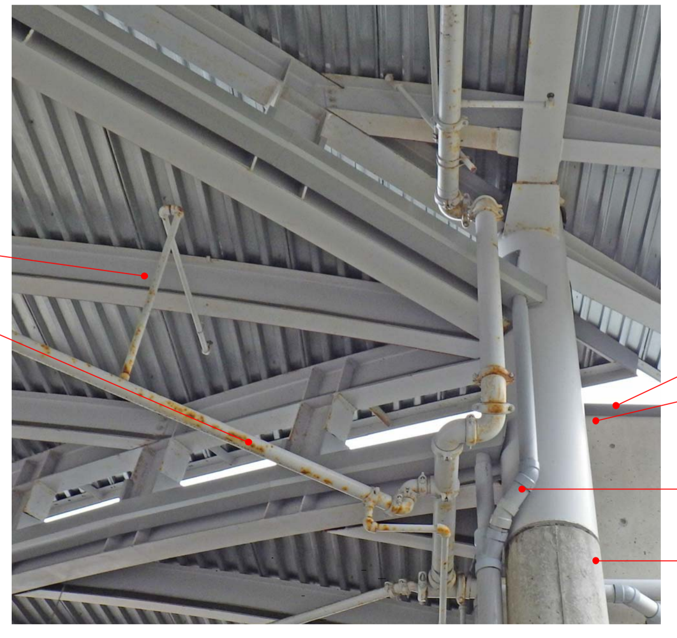
5 TIA CANOPY INTERFACE A303 TYPICAL EXTG CONDITION OF STRUCTURAL STEEL AND FIRE PROTECTION PIPING AT SIA CANOPY/TIA CANOPY INTERFACE
