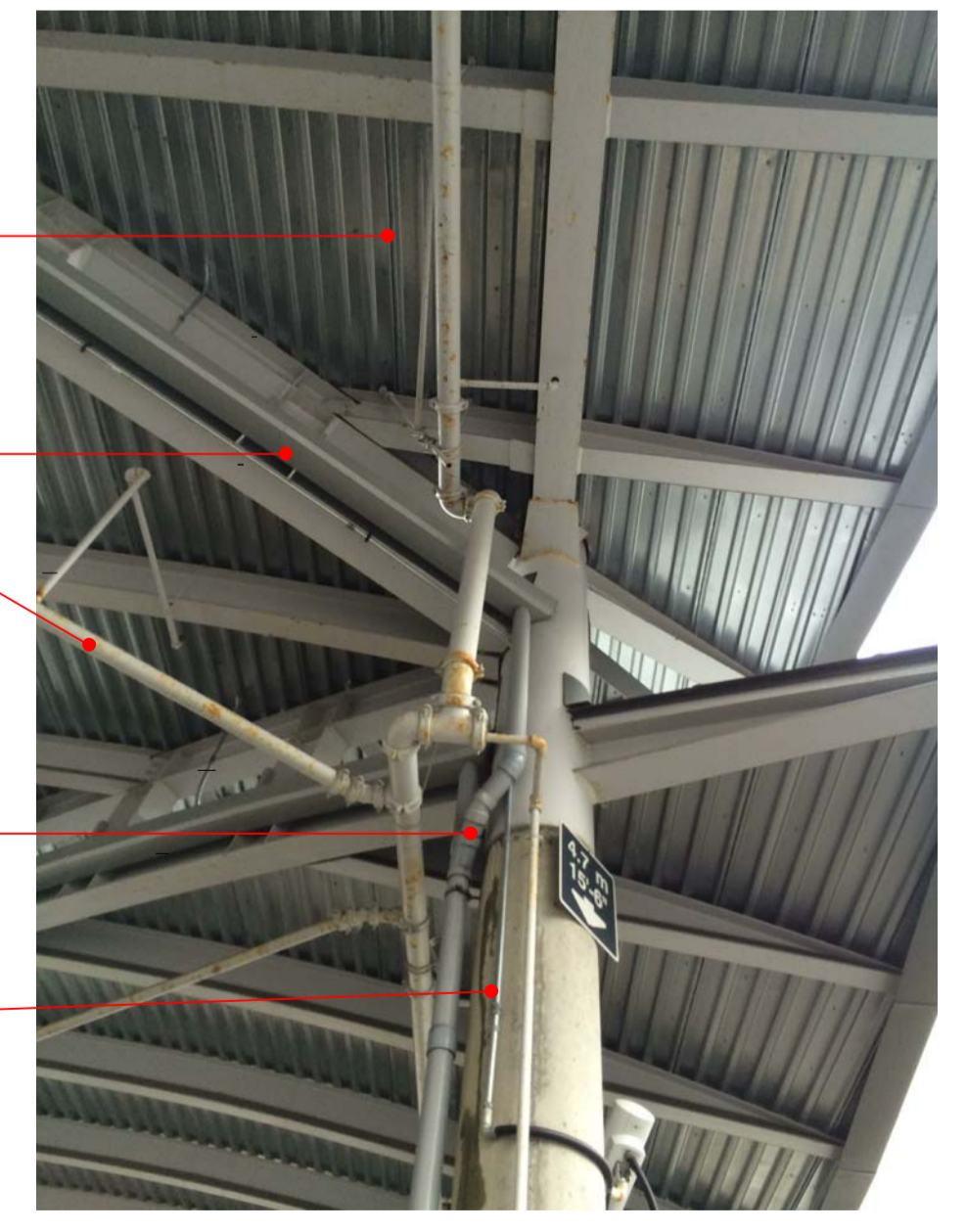
3 SIA OVERLAPPING ROOF INTERFACE A303 TYPICAL EXTG CONDITION OF STRUCTURAL STEEL, FIRE PROTECTION PIPING, RAIN WATER LEADERS AND GALVANIZED DECK
