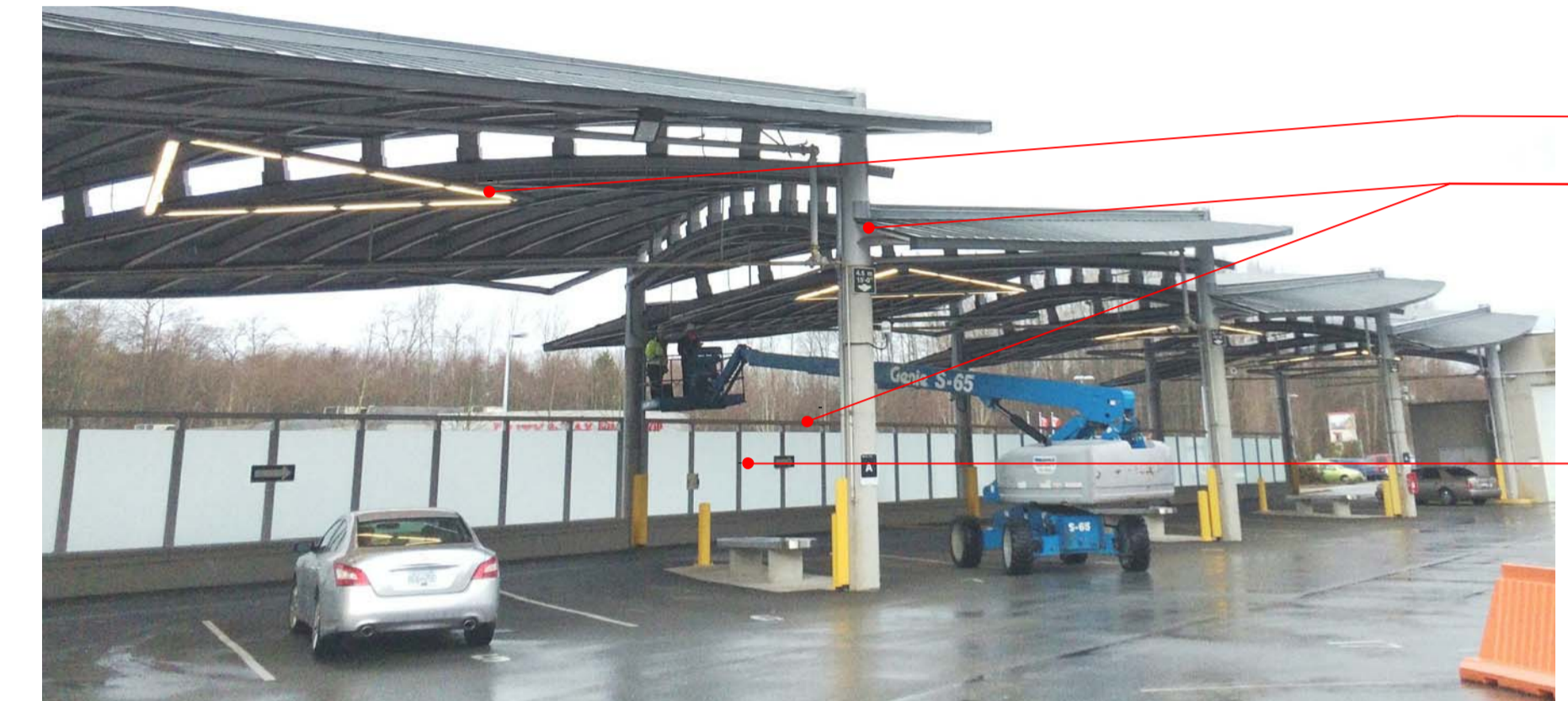
2 SIA CANOPY EAST ELEVATION A304 TYPICAL EXTG CONDITION OF STEEL CANOPY, FIRE PROTECTION PIPING AND PEDESTRIAN SCREEN
