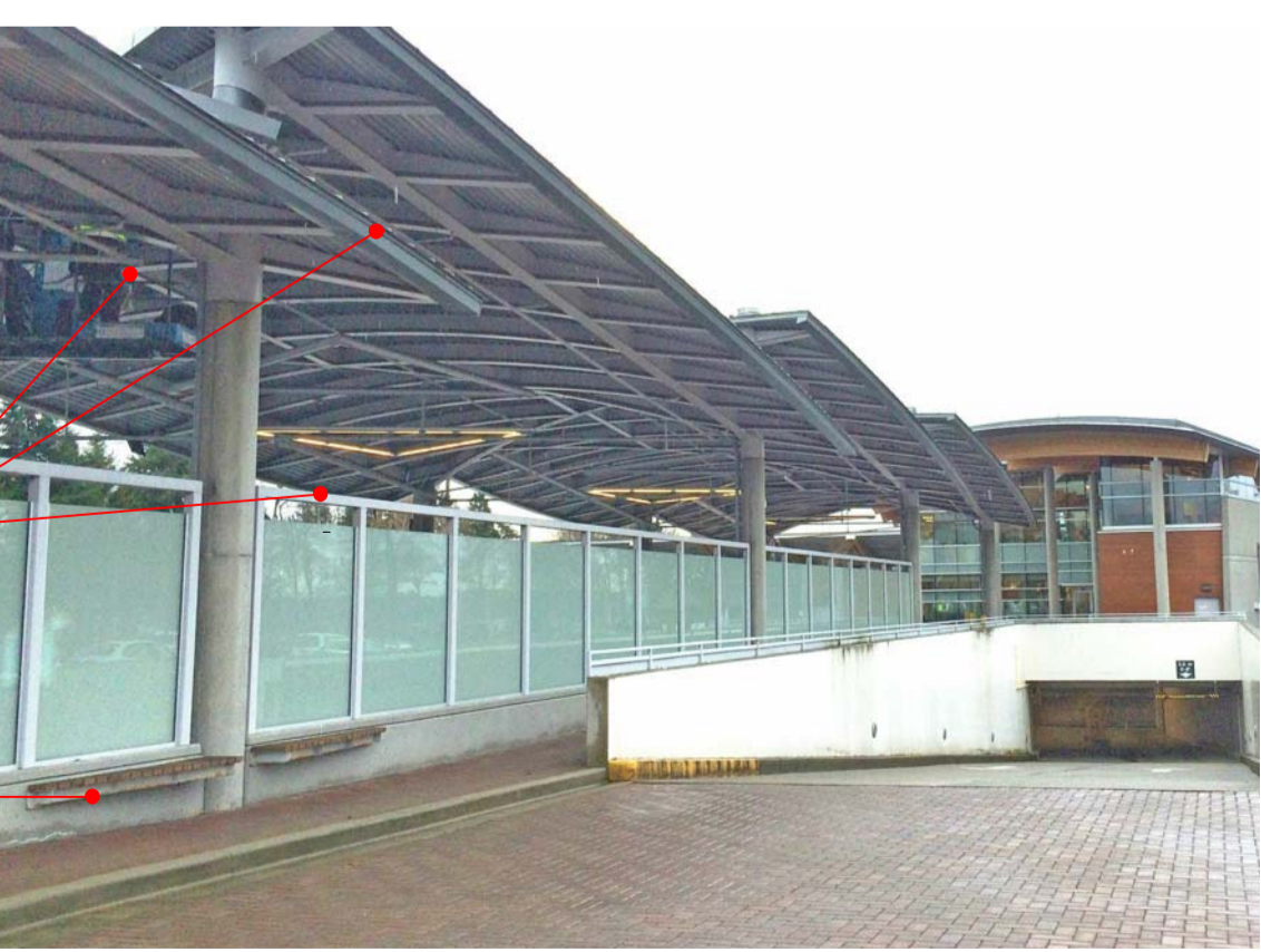
5 SIA PEDESTRIAN SCREEN A304 TYPICAL EXTG CONDITION OF PEDESTRIAN SCREEN AND BENCH
