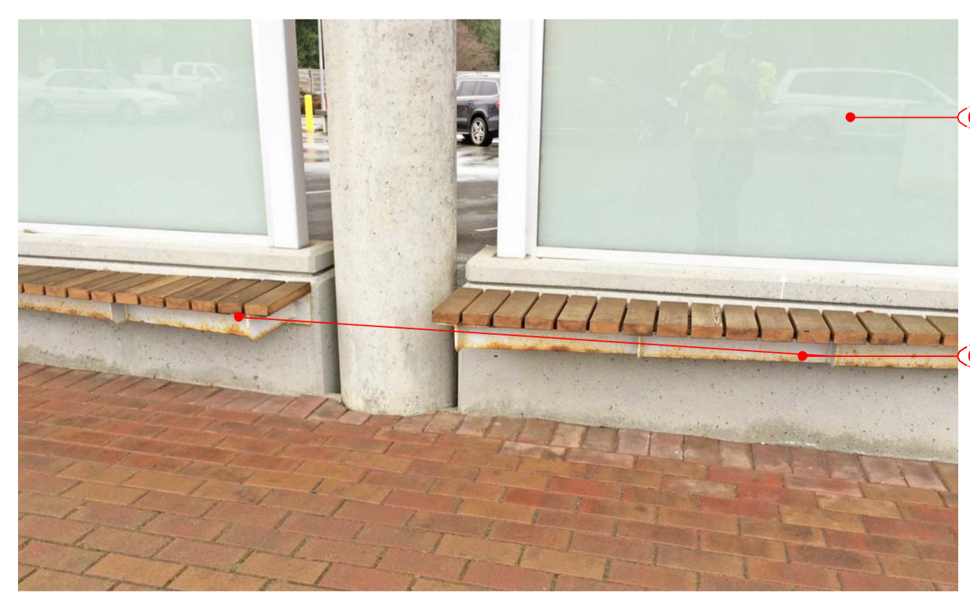
6 SIA - PEDESTRIAN SCREEN AND BENCH A304 TYPICAL EXTG CONDITION OF PEDESTRIAN SCREEN AND STEEL BENCH SUPPORTS
