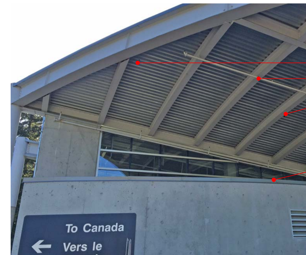
4 TIA - SOUTH ELEVATION A306 TYPICAL EXTG CONDITION OF TERTIARY INSPECTION BUILDING WITH LOWER ROOF AND CLERESTORY GLAZING
