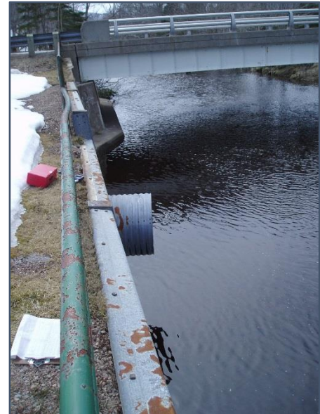
Figure 3. Showing a section of the steel retaining wall to be removed on the south bank of the river at the Big Intervale Campground/DUA.
