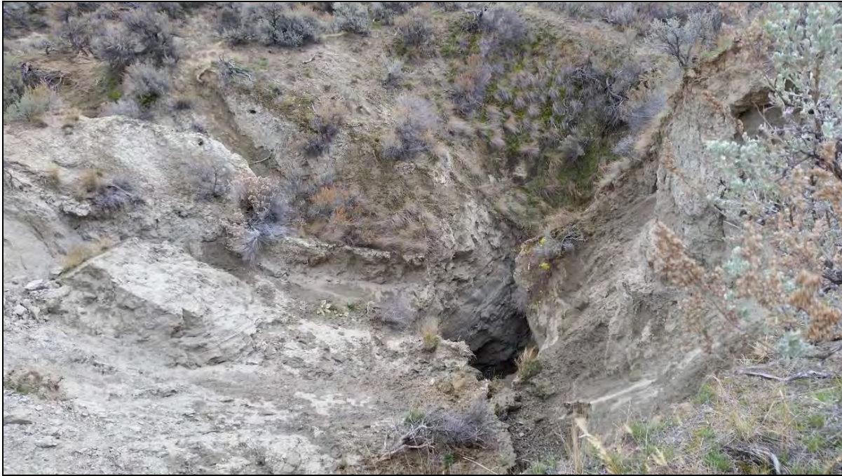
Photograph 3: South-east view looking into the downslope end of the failure where sediment flowed into a sinkhole.
