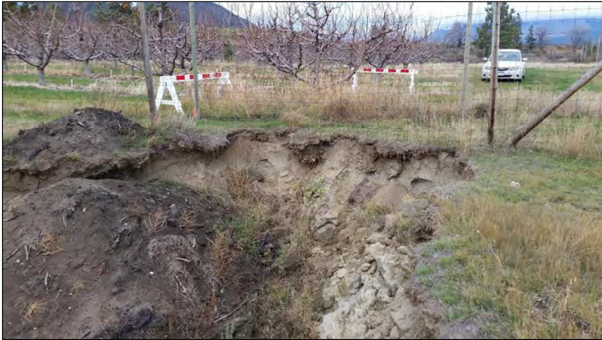
Photograph 5: North-west view of the failure showing proximity of the apple orchard behind.
