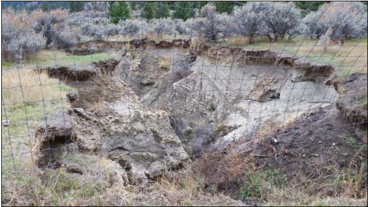
Photograph 1: South facing view of the failure taken from within the orchard.
