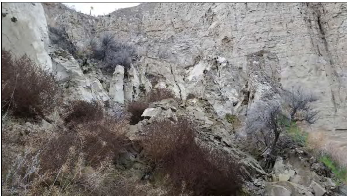
Photograph 12: View looking north-west up failing slopes of the steep bank below the gully.
