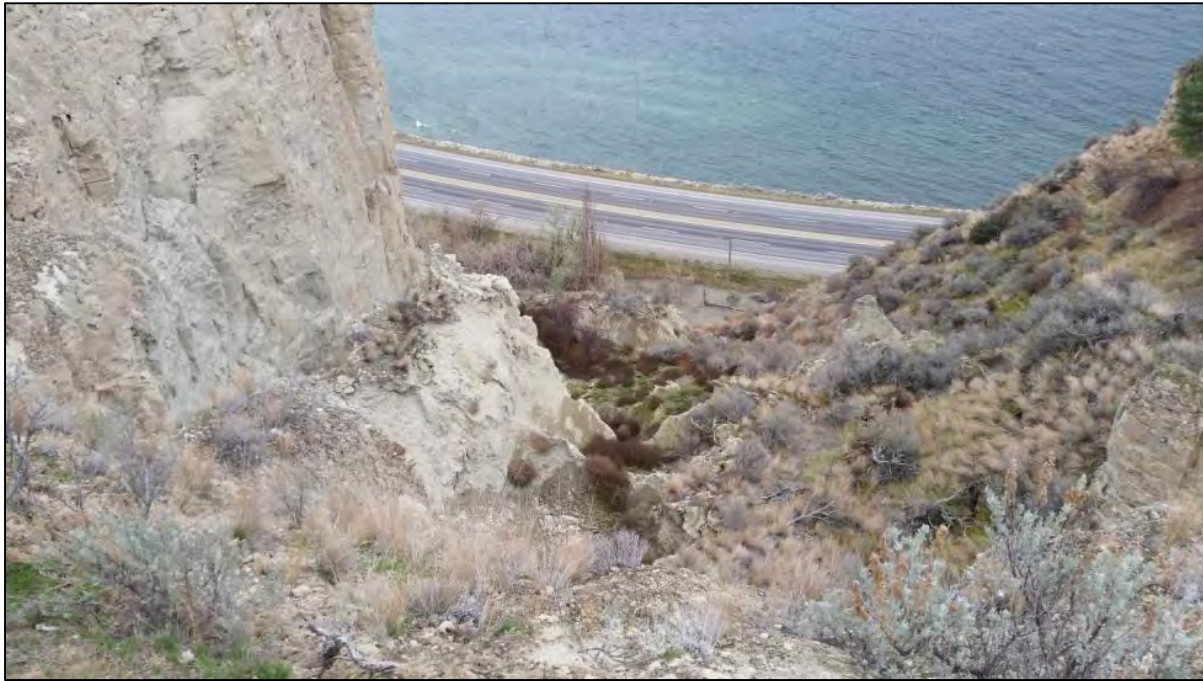
Photograph 7: East facing view down the steep bluffs where erosion has caused bank failures. Highway 97 and Okanagan Lake are in the distance.
