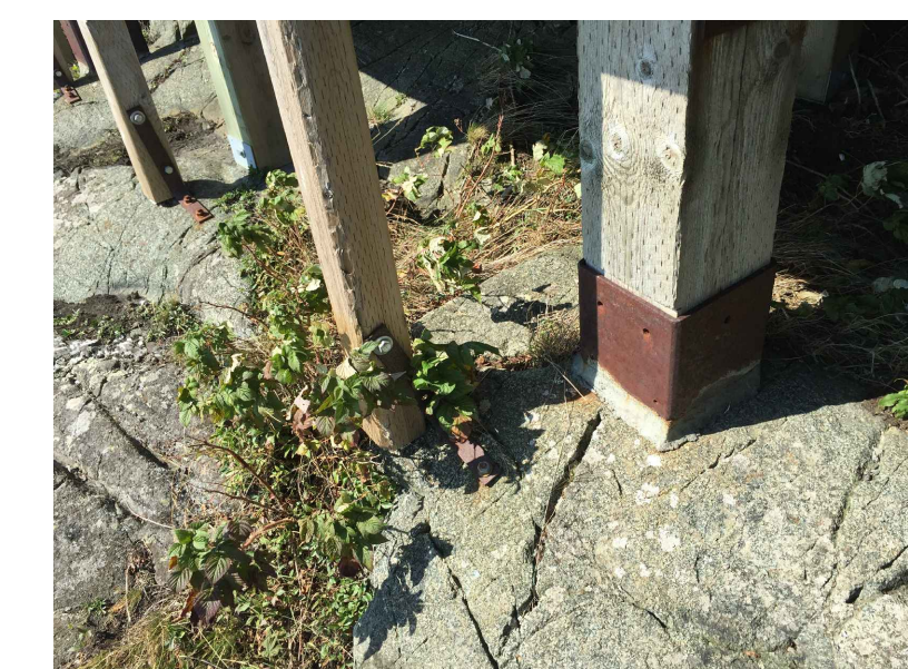
VIEW OF MISSING SUPPORT BOLTING ADD LAG SCREWS
