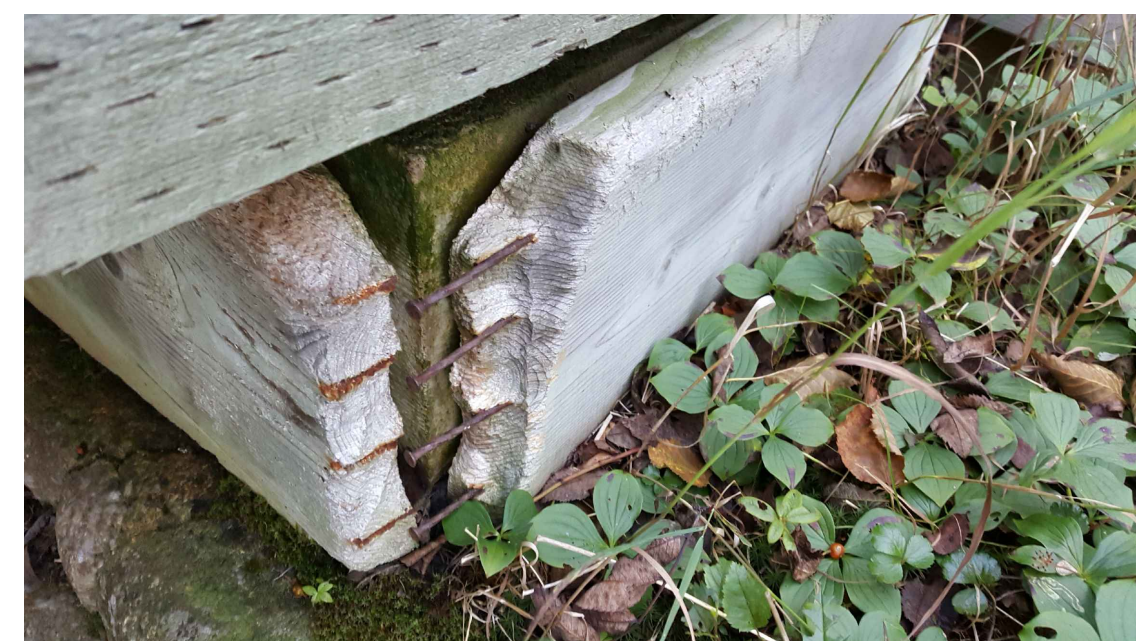
VIEW OF RUSTED NAILS TO BE REMOVED
