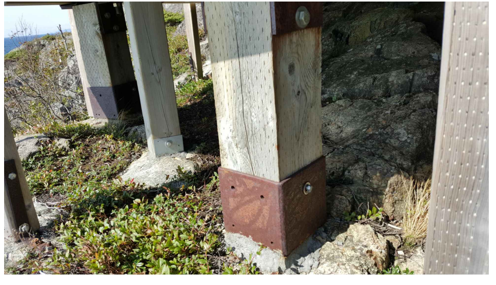
VIEW OF MISSING POST BOLTS (TYP.)
