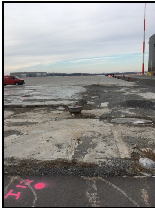
Photograph 6: View from southeast corner of concrete pad (to be removed) of former Hangar 6 looking north towards airfield (apron)
