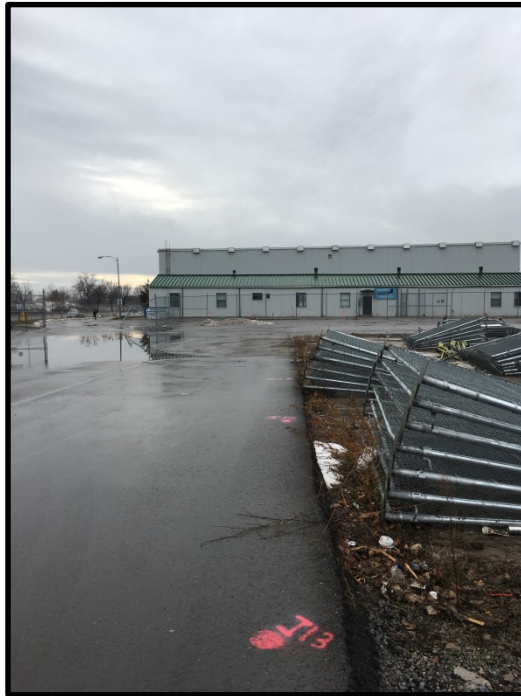
Photograph 5: View from east edge of area to be excavated looking west towards Building 65 (part of Hangar 7)
