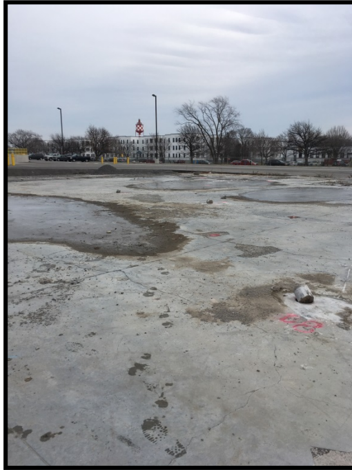
Photograph 3: View from northwest corner of concrete pad (to be removed) of former Hangar 6 looking southeast towards Highway 2
