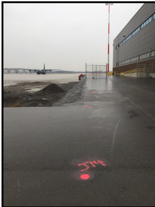
Photograph 8: View from North Star Drive: southeast corner of area to be excavated, looking north towards airfield (apron). New Hangar 6 located on the east
