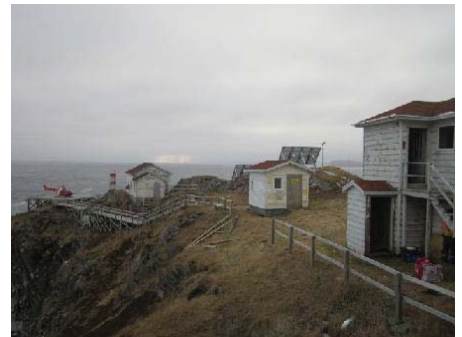
Photo 6: View of damaged fencing near new equipment building.
