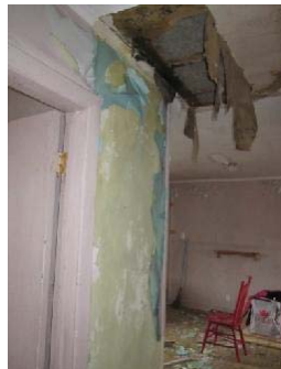
Photo 71: View of collapsed drywall and areas of flaking paint in Hallway 1.
