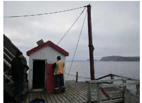
Photo 15: View of lower landing deck, winch house and spar. Note: missing boom.
