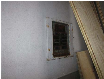
Photo 41: View of electrical panel in Room 1.
