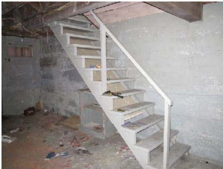
Photo 19: View of Basement 1 in double dwelling. Note: flaking paint on floor.
