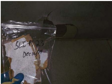
Photo 40: View of paint sample BLI-PS23 and location of mould sample BLI-MS1.
