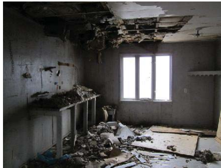
Photo 14: View of Workshop in double dwelling. Note: ceiling debris on floor.
