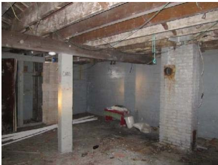
Photo 22: View of Basement 1 in double dwelling. Note: smoke detector.
