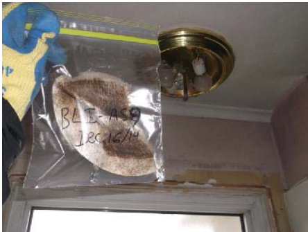
Photo 37: View of heat shield insulation sample BLI-AS9.
