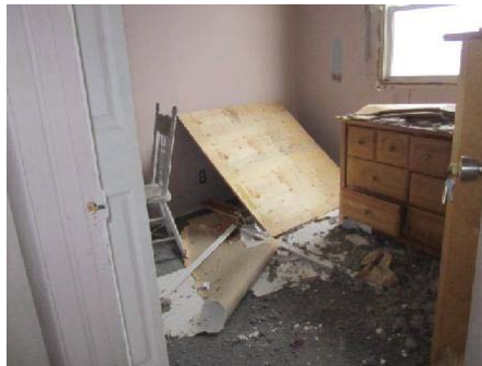
Photo 17: View of Bedroom 2-2 in double dwelling. Note: ceiling debris on floor.
