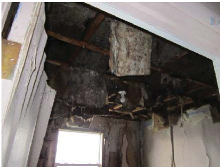
Photo 16: View of Bedroom 1-2 in double dwelling. Note: collapsed ceiling.
