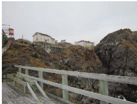
Photo 5: View of upper landing railing and collapsed walkway to double dwelling.
