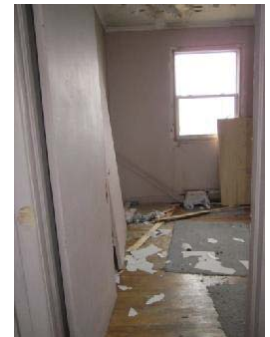
Photo 18: View of Bedroom 3-2 in double dwelling. Note: flaking paint debris on floor.
