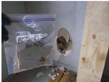
Photo 65: View of paint sample BLI-PS8 and location of mould sample BLI-MS2.
