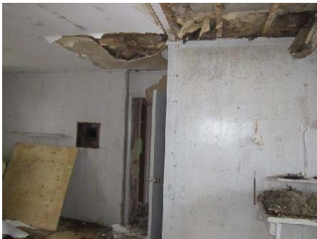
Photo 70: View of collapsed drywall and areas of SVG on drywall in Workshop.
