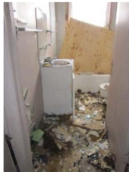
Photo 11: View of Bathroom 1 in double dwelling. Note: ceiling debris on floor.
