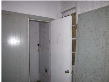
Photo 11: View of Battery Room in old equipment building.
