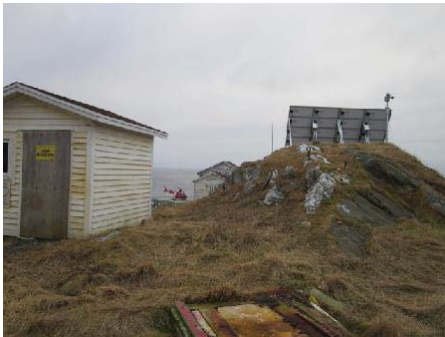
Photo 7: View of solar array panels and new equipment building.
