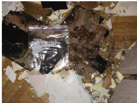
Photo 41: View of vinyl sheet floor tile and vinyl sheet flooring/mastic sample BLI-AS13.
