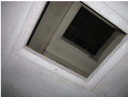
Photo 16: View of access hatches to double ceiling area/attic in old equipment building.
