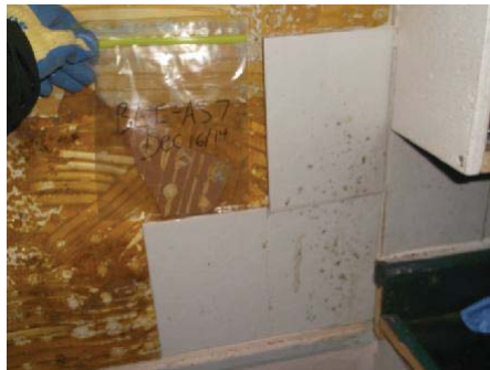
Photo 35: View of ceramic tile and mastic sample BLI-AS7.
