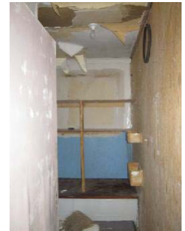
Photo 15: View of Bathroom 2 in double dwelling. Note: flaking paint.
