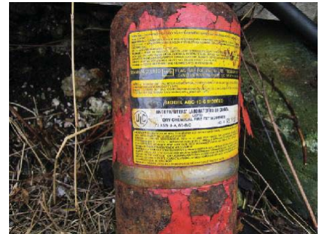
Photo 21: View of fire extinguisher label (dry chemical).
