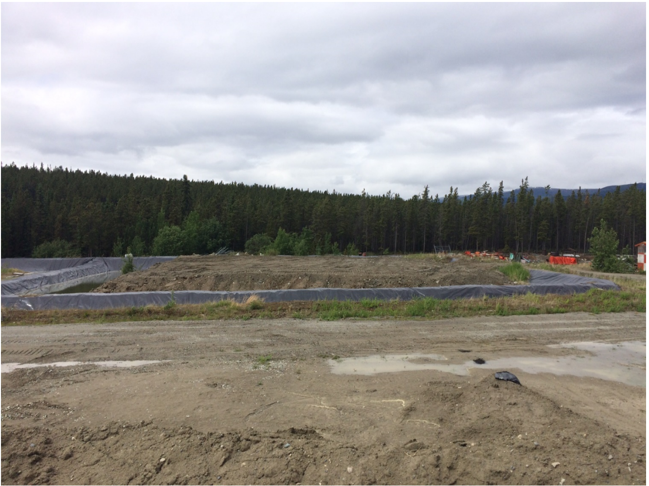
Photo 2: View from the Bioremediated Soil Storage Area showing LTF 1 located on the northwest section of the work area.
