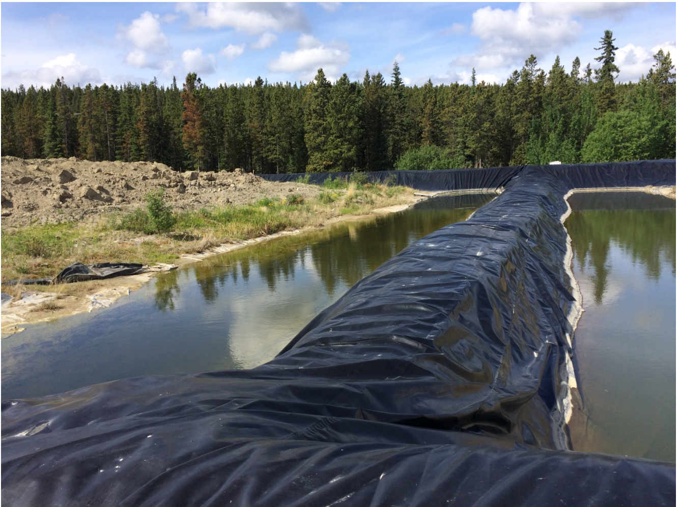
Photo 3: View of LTF 1 and 2 sumps with water for discharge.
