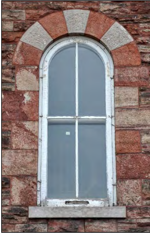
Figure 38: Exterior elevation of second floor window type (W209) at the Superintendent's House. [CLA-PWGSC/November 2012]
