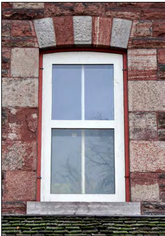
Figure 32: Exterior elevation of second floor window type (W201) at the of the Superintendent's House. [CLA-PWGSC/November 2012]
