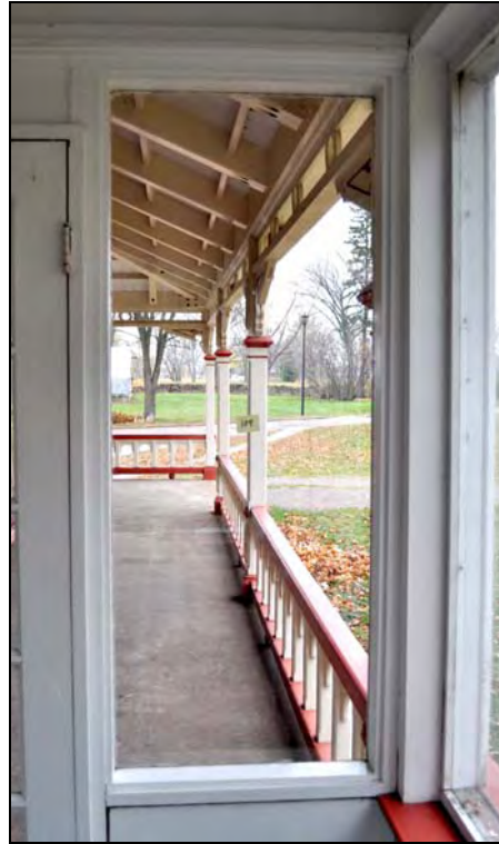
Figure 25: Interior elevation of ground floor window type (W104) at the Superintendent's House. [CLA-PWGSC/November 2012]
