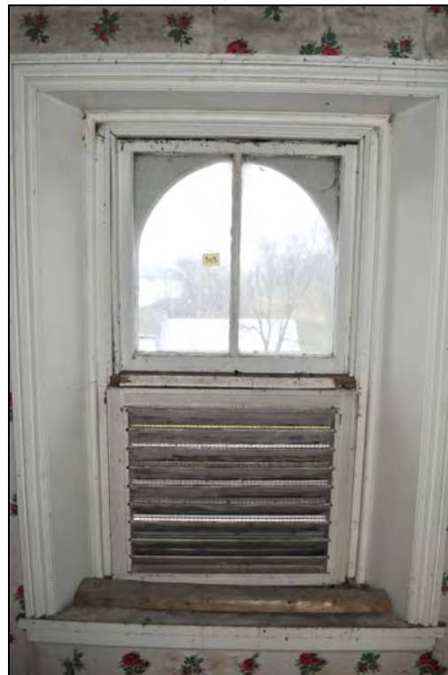
Figure 41: Interior elevation of third floor window type (W303) at the Superintendent's House. [CLA-PWGSC/November 2012]
