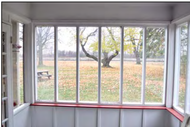
Figure 27: Interior elevation of ground floor window type (W105) at the sun room of the Superintendent's House. [CLA-PWGSC/November 2012]
