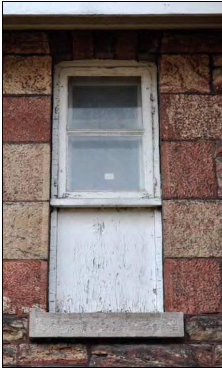
Figure 34: Exterior elevation of second floor window type (W205) at the Superintendent's House. [CLA-PWGSC/November 2012]
