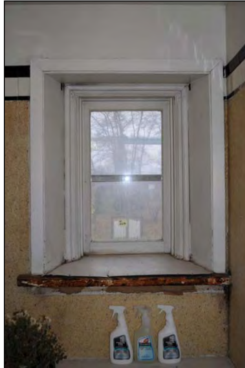
Figure 35: Interior elevation of second floor window (W205) type at the Superintendent's House. [CLA-PWGSC/November 2012]
