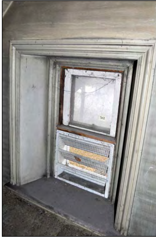
Figure 43: Interior elevation of third floor window type (W302) at the Superintendent's House. [CLA-PWGSC/November 2012]
