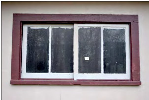
Figure 30: Exterior elevation of ground floor window type (W113) at rear addition of the Superintendent's House. [CLA-PWGSC/November 2012]
