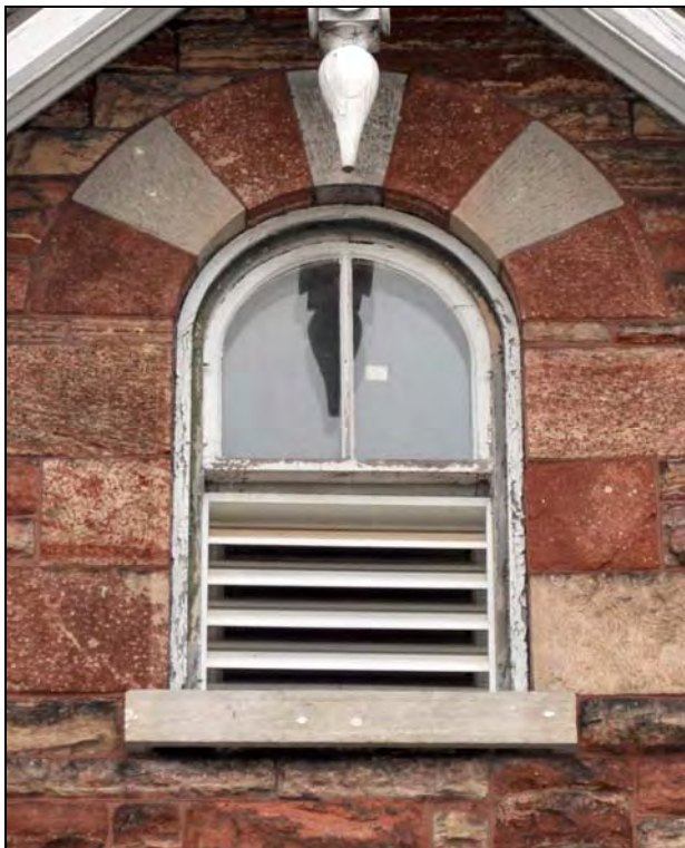
Figure 40: Exterior elevation of third floor window type (W303) at the Superintendent's House. [CLA-PWGSC/November 2012]
