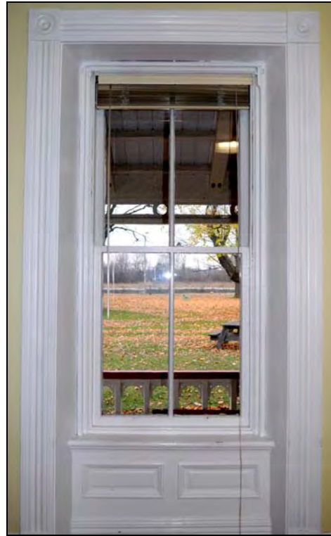
Figure 23: Interior elevation of ground floor window type (W101) at the Superintendent's House. [CLA-PWGSC/November 2012]
