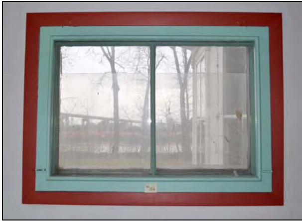
Figure 29: Interior elevation of ground floor window type (W106) at the sun room of the Superintendent's House. [CLA-PWGSC/November 2012]
