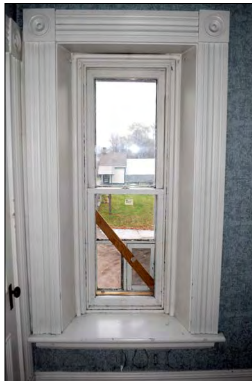
Figure 37: Interior elevation of second floor window type (W207) at the Superintendent's House. [CLA-PWGSC/November 2012]
