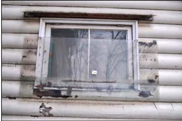
Figure 28: Exterior elevation of ground floor window type (W106) at the sun room of the Superintendent's House. [CLA-PWGSC/November 2012]
