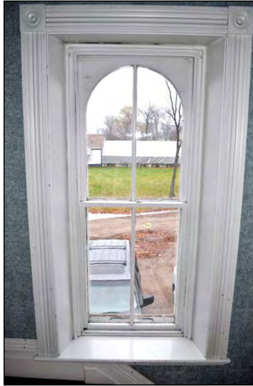
Figure 39: Interior elevation of second floor window type (W209) at the Superintendent's House. [CLA-PWGSC/November 2012]
