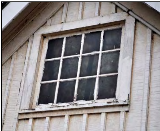
Figure 44: Exterior elevation of second floor window type (W211) at the of the Superintendent's House. [CLA-PWGSC/November 2012]
