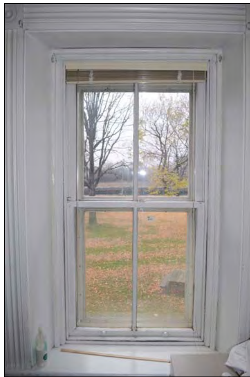
Figure 33: Interior elevation of second floor window type (W201) at the of the Superintendent's House. [CLA-PWGSC/November 2012]
