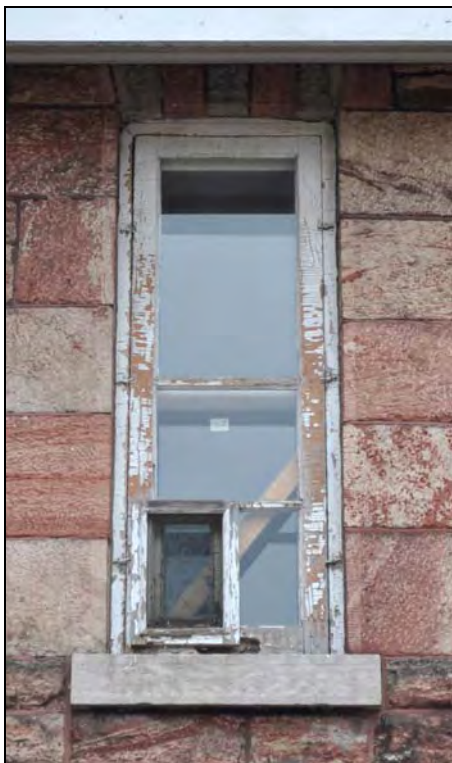
Figure 36: Exterior elevation of second floor window type (W207) at the Superintendent's House. [CLA-PWGSC/November 2012]
