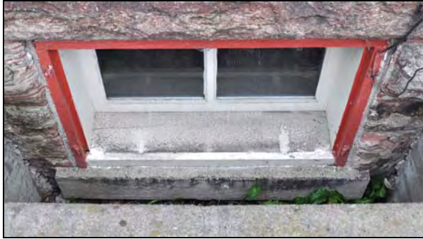
Figure 20: Exterior elevation of basement window type (W001) at the Superintendent's House. [CLA-PWGSC/November 2012]
