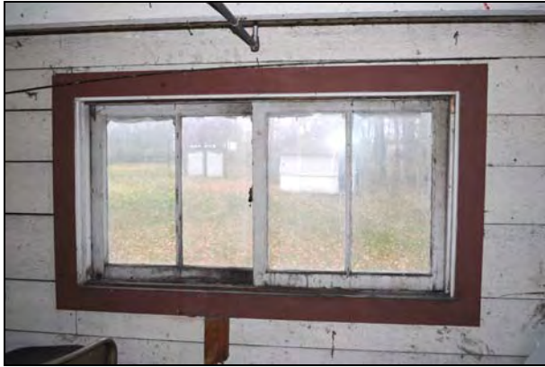
Figure 31: Interior elevation of ground floor window type (W113) at rear addition of the Superintendent's House. [CLA-PWGSC/November 2012]
