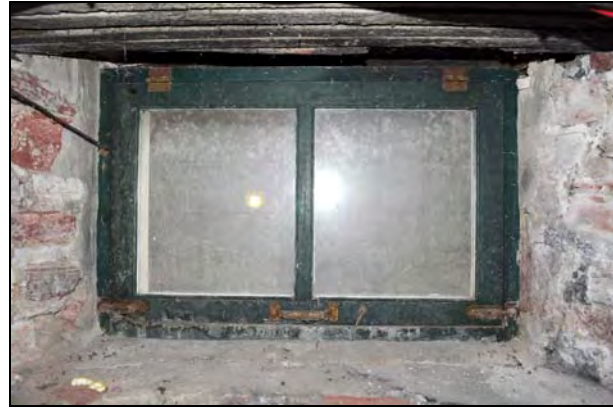
Figure 21: Interior elevation of basement window type (W001) at the Superintendent's House. [CLA-PWGSC/November 2012]
