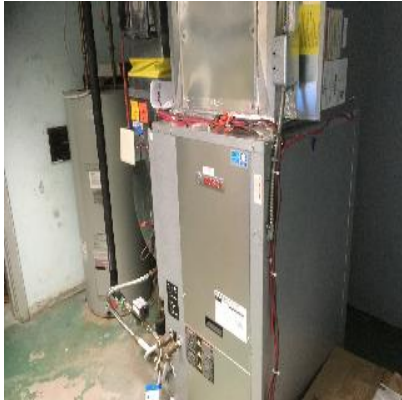
Photo 2: Mechanical equipment uninsulated in basement.
