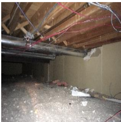
Photo 1: Ductwork in crawlspace. Uninsulated.
