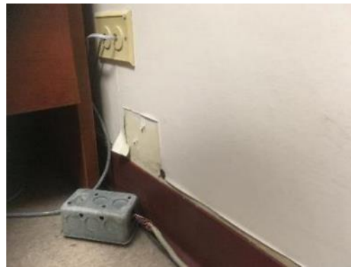
Photo 11: Water damage observed on drywall in general office area.
