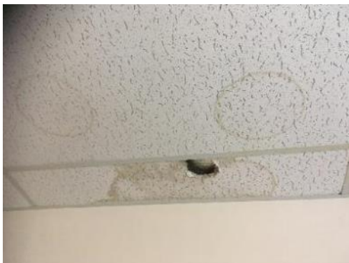
Photo 12: Water damaged acoustic ceiling tiles. General office area.
