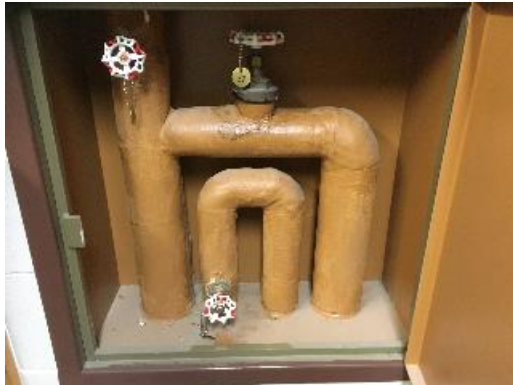
Photo 1: Parging cement on elbows of water lines.
