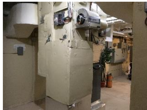
Photo 3: Fibreglass insulation covered with canvas on mechanical equipment. No parging noted.
