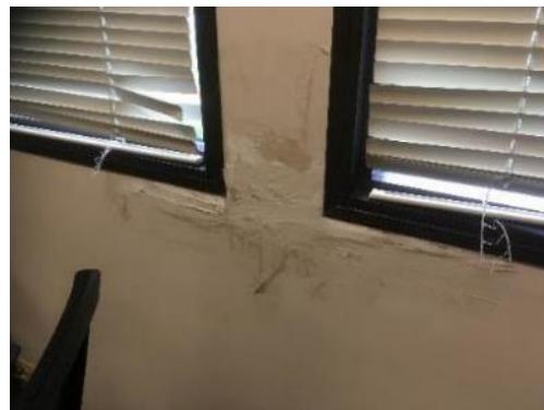
Photo 13: Water damaged drywall adjacent to windows on east exterior wall.
