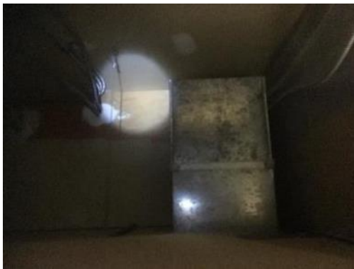
Photo 10: Water damage on drywall. East exterior wall.
