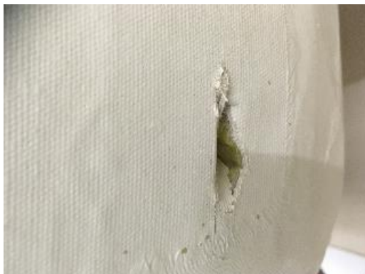
Photo 2: Basement mechanical room. Fibreglass insulation covered with canvas. No parging noted.
