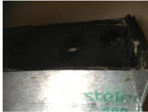
Photo 9: Asbestos-containing black mastic applied to fibreglass insulation inside duct work observed in the NCO Room (0004A-C).
