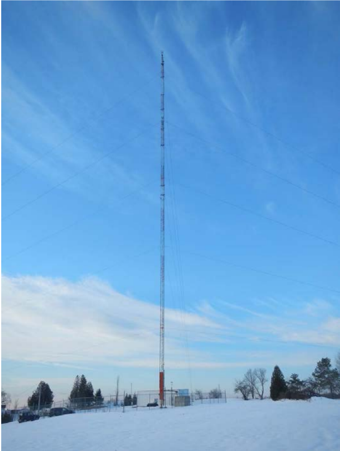
Figure 3: Cobourg MCTS Tower
