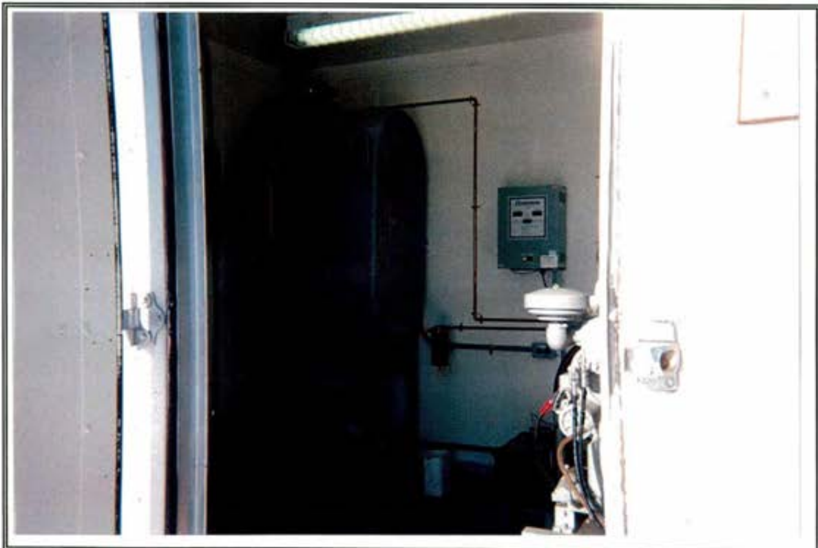
PHOTO 6: VIEW OF DIESEL FUEL AST IN GENERATOR BUILDING; NOTE VENT PIPE EXITING STRUCTURE AND FILL PIPE AT TOP OF TANK.
