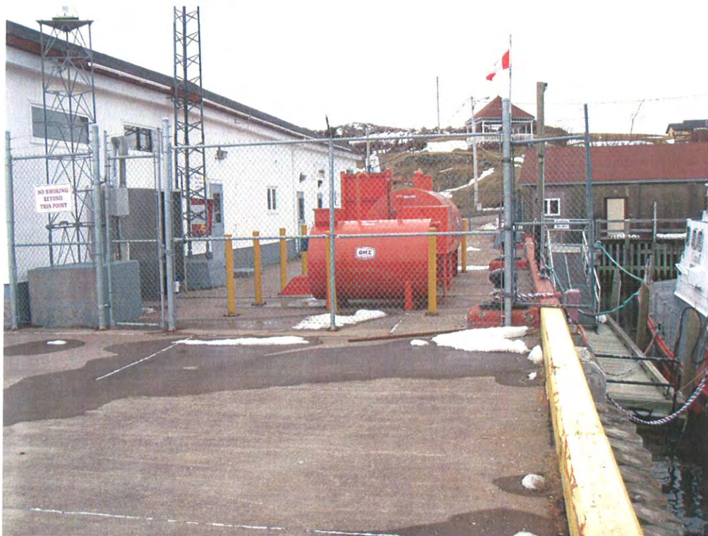
Photo 3: Waste oil AST and fuel oil AST located on the north side of the wharf, looking northwest.
