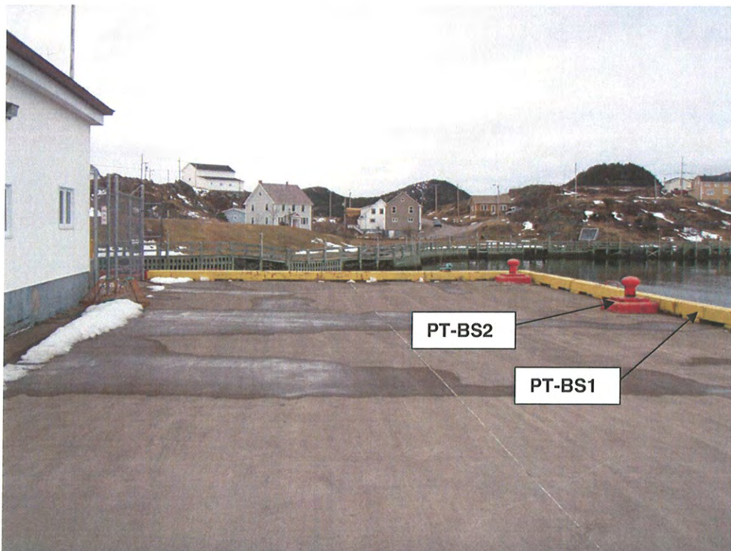
Photo 2: Concrete wharf deck showing yellow wheel guard and red bollards, facing northeast.
