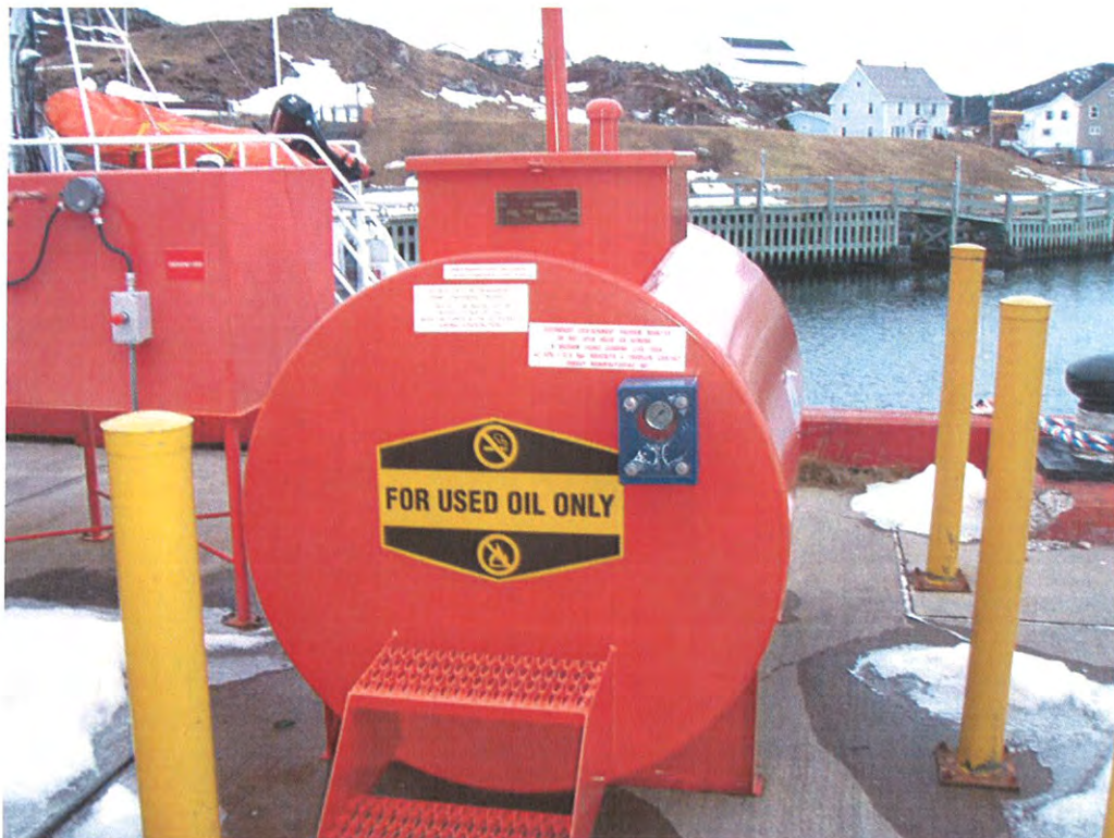
Photo 6: 2,273 L waste oil tank located on the northeastern side of the wharf. Photo taken looking northeast.
