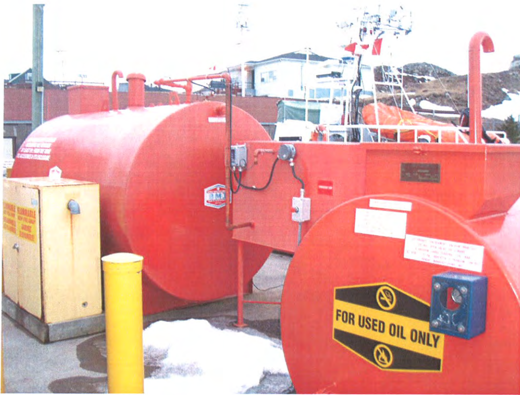
Photo 9: Location of chemical storage locker on the wharf. Photo taken looking north.
