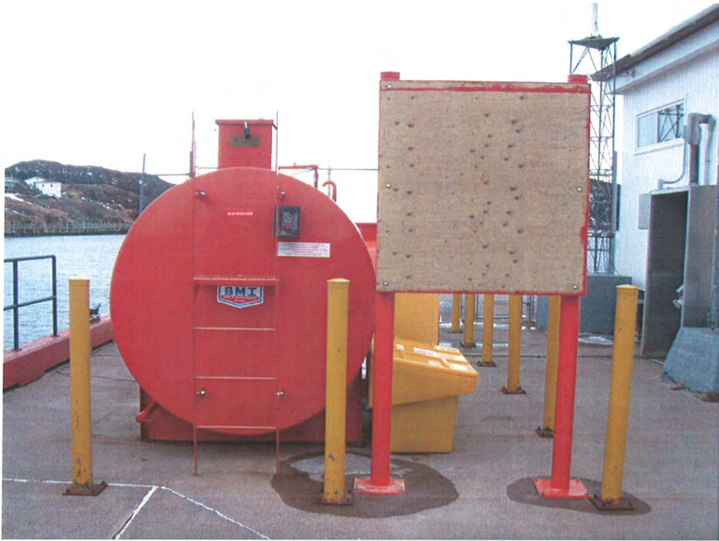
Photo 7: 6,819 L fuel oil tank located on the northeastern side of the wharf. Photo taken looking southeast.
