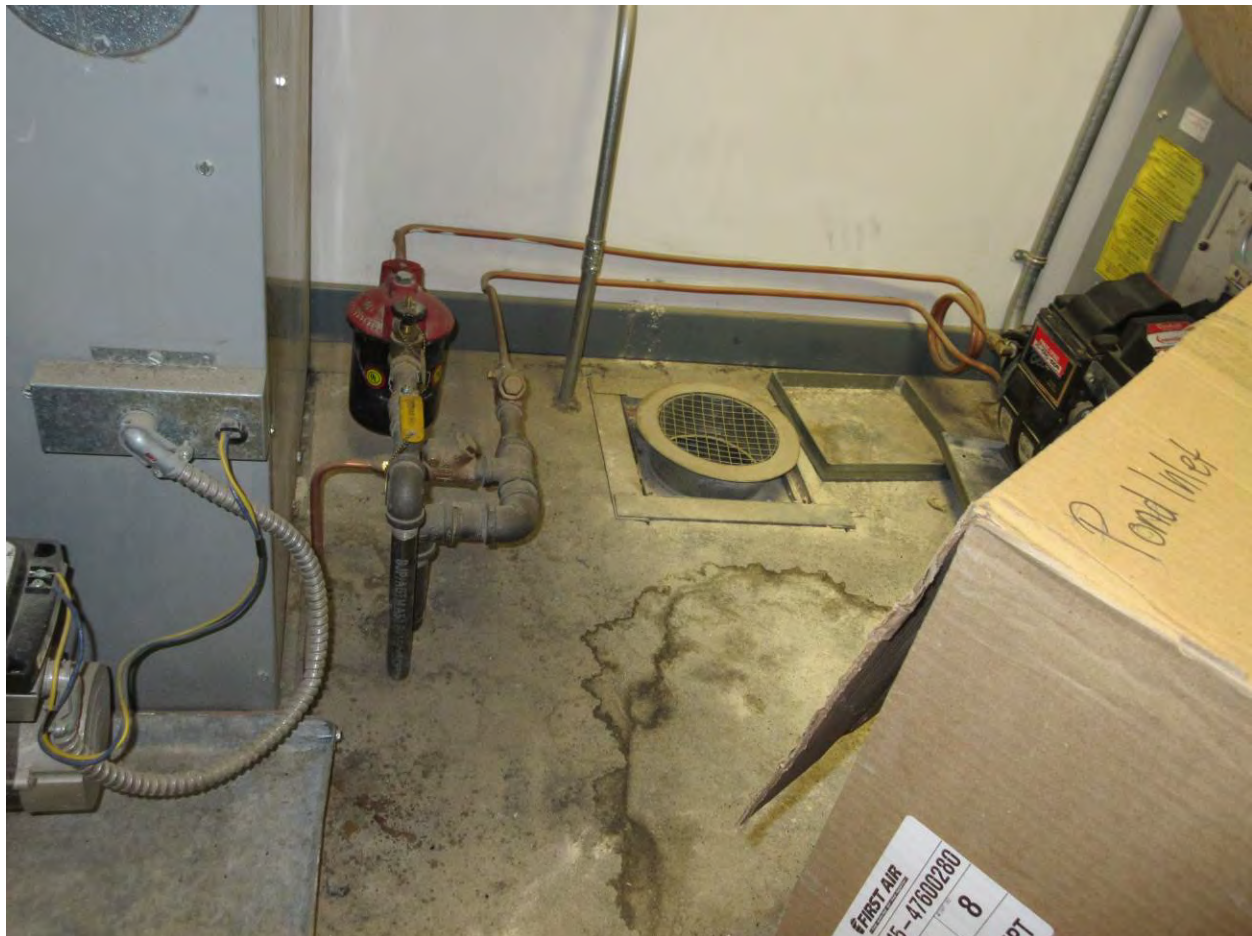
Photo 14 Furnace No. 4 Piping
