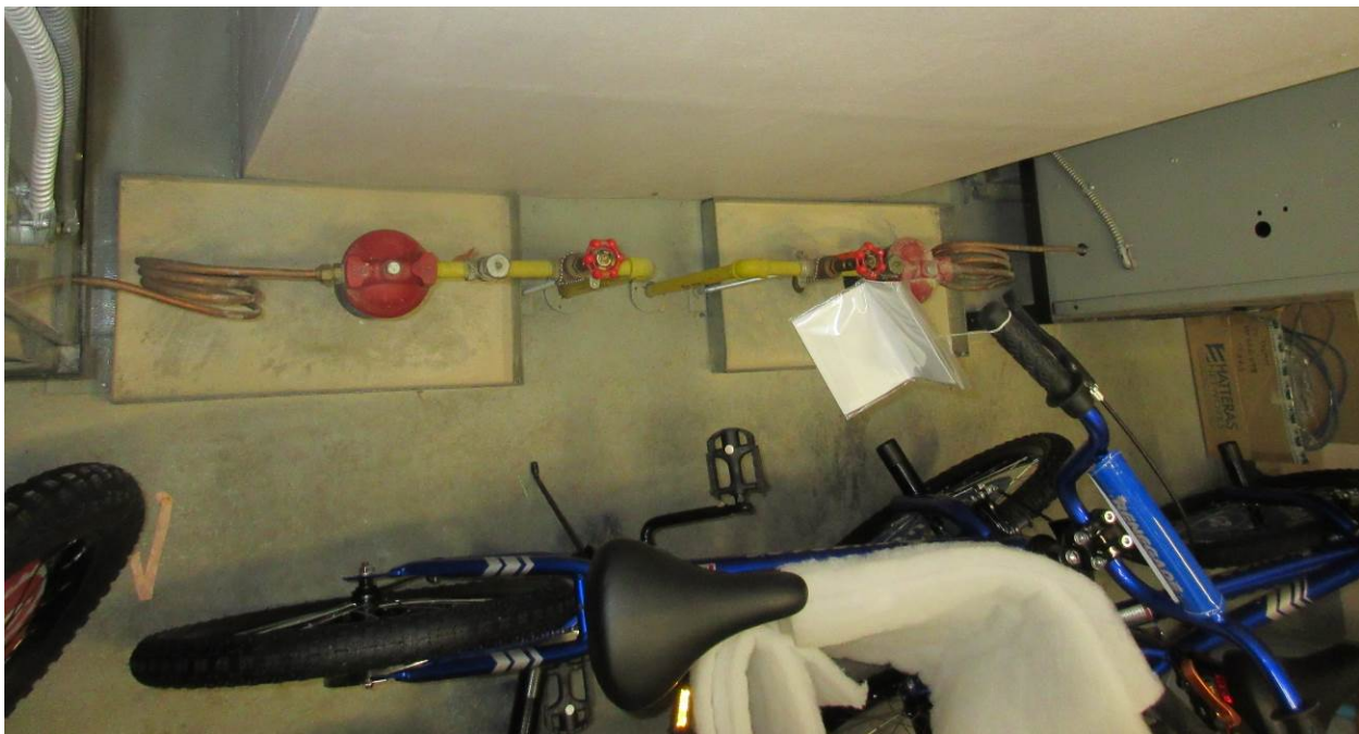
Photo 12 Interior Furnace 1 and 2 Piping
