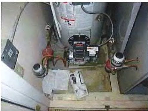
Photo 3: Interior piping and accessories
