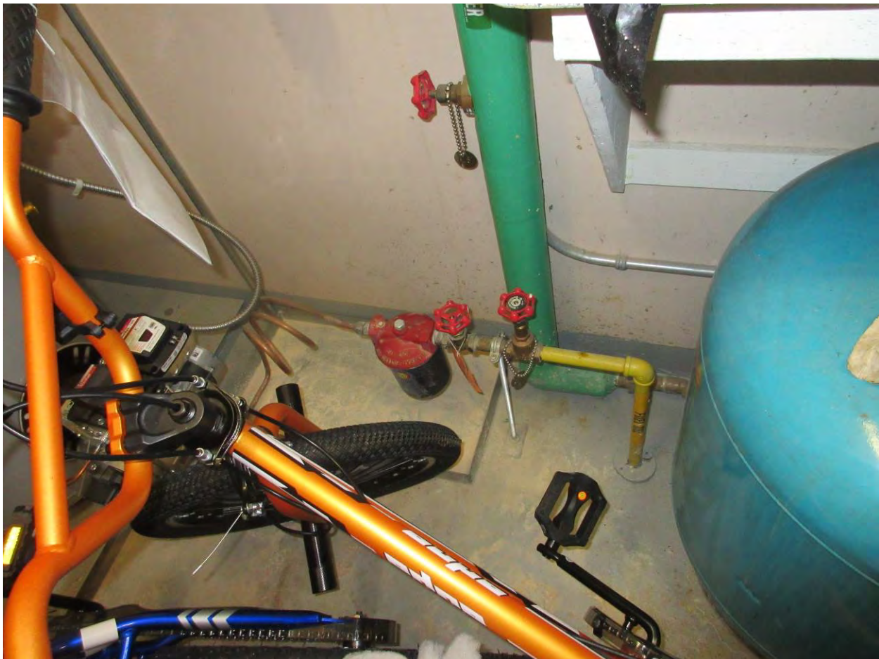
Photo 14 Hot Water Tank Fuel Piping
