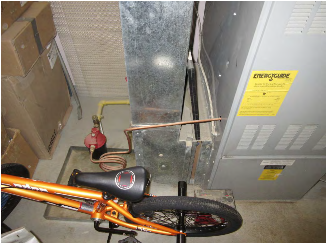
Photo 18 Furnace No.3 Fuel Piping
