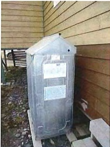
Photo 1: Outdoor above ground fuel tank
