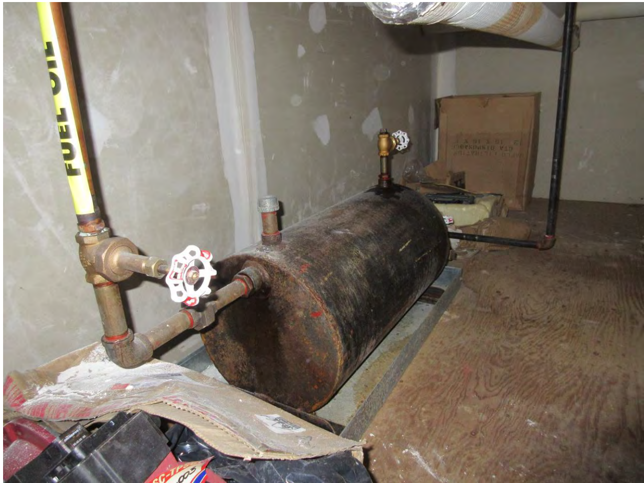
Photo 13 INTERIOR DAY TANK – BOILERS
