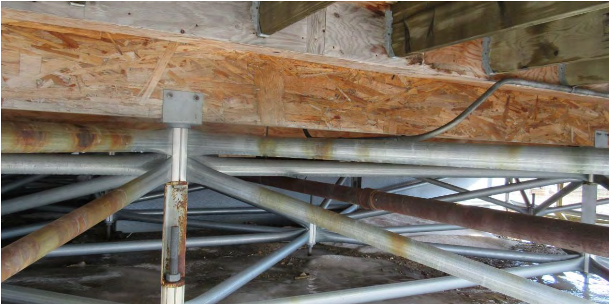
Photo 2 Exterior Piping Under Duplex
