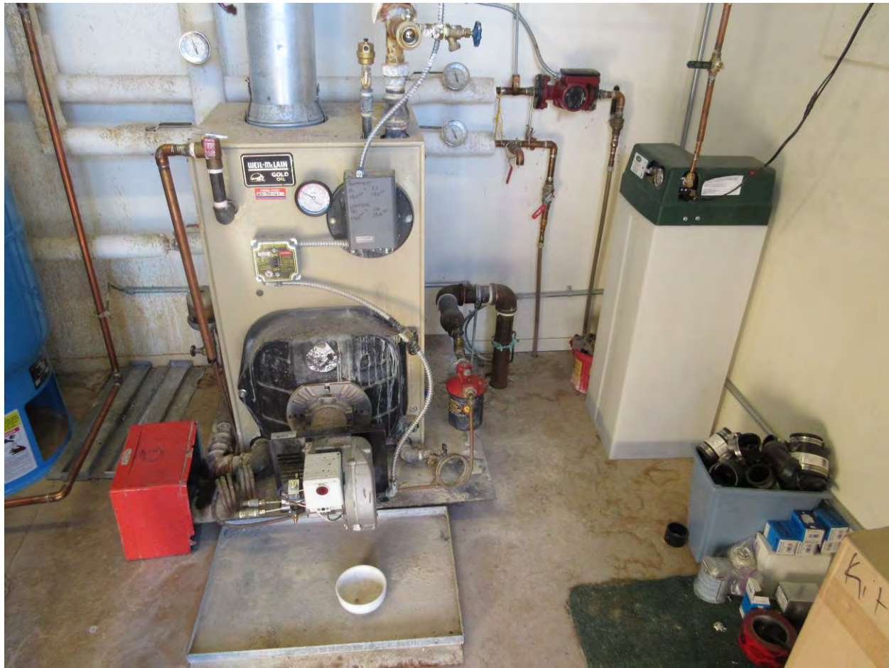
Photo 3 Mechanical Room Piping
