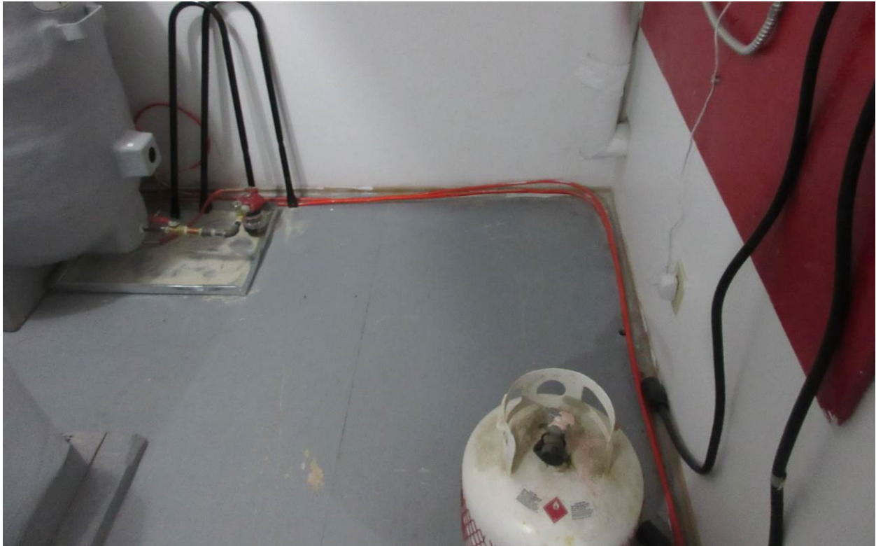
Photo 19 Fuel Lines On Floor
