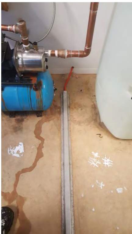
Photo 16 Interior Piping from exterior tank
