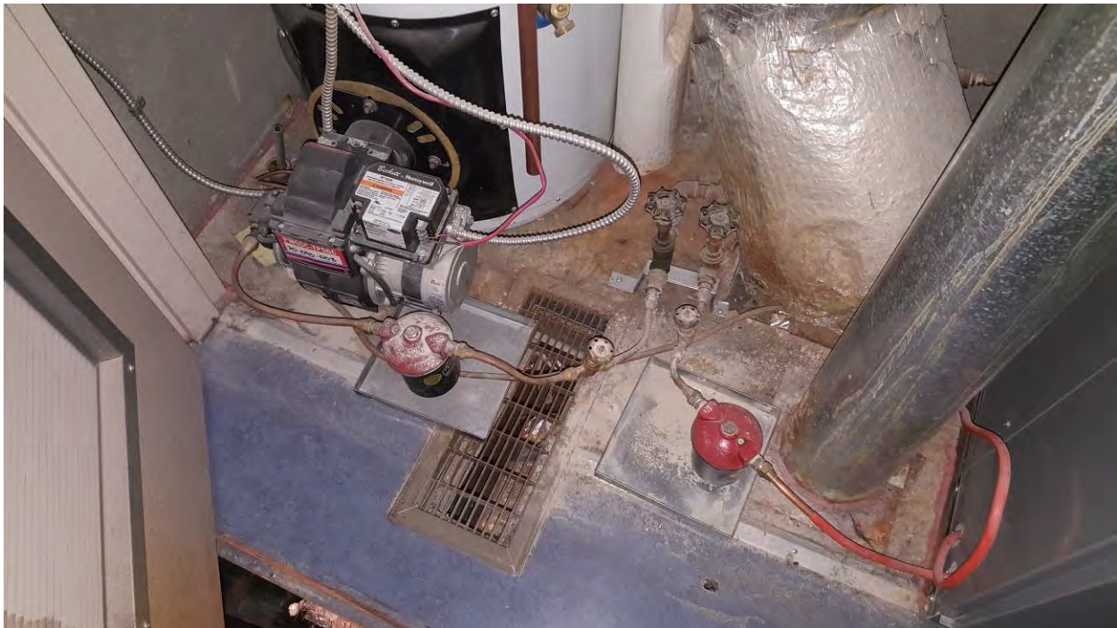
Photo 18 Hot water tank piping
