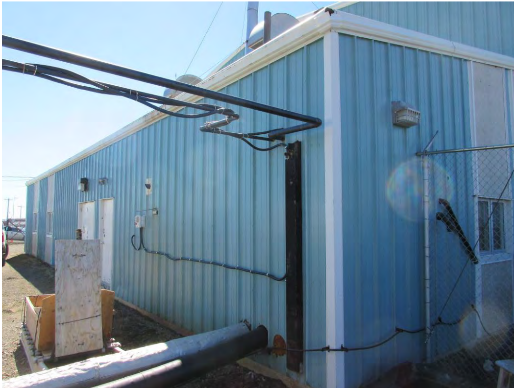
Photo 4 Piping into Building
