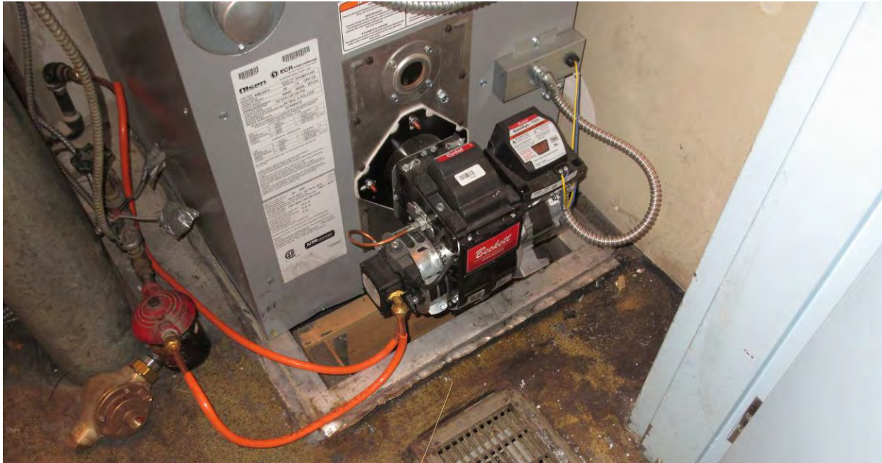
Photo 11 Furnace No. 2 Piping
