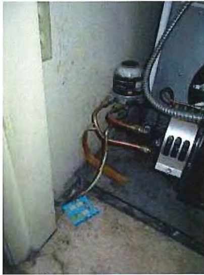
Photo 5: Indoor piping & accessories
