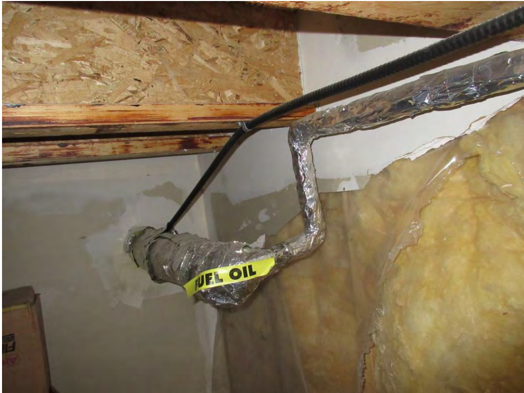
Photo 11 FUEL PIPE ENTRY INTO CRAWL SPACE
