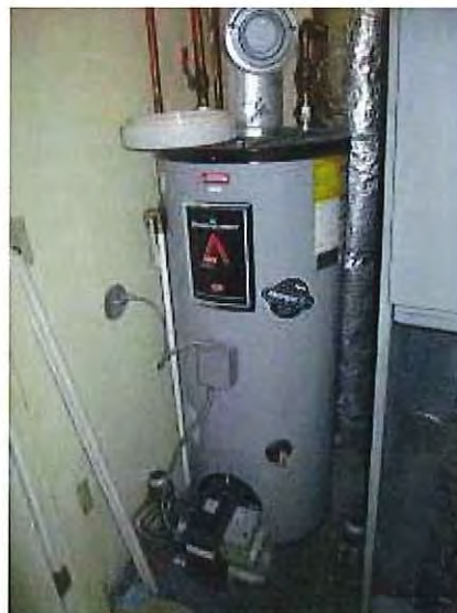
Photo 4: Indoor water heater
