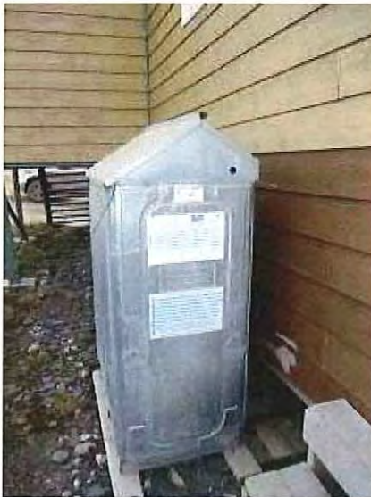
Photo 1: Outdoor above ground fuel tank
