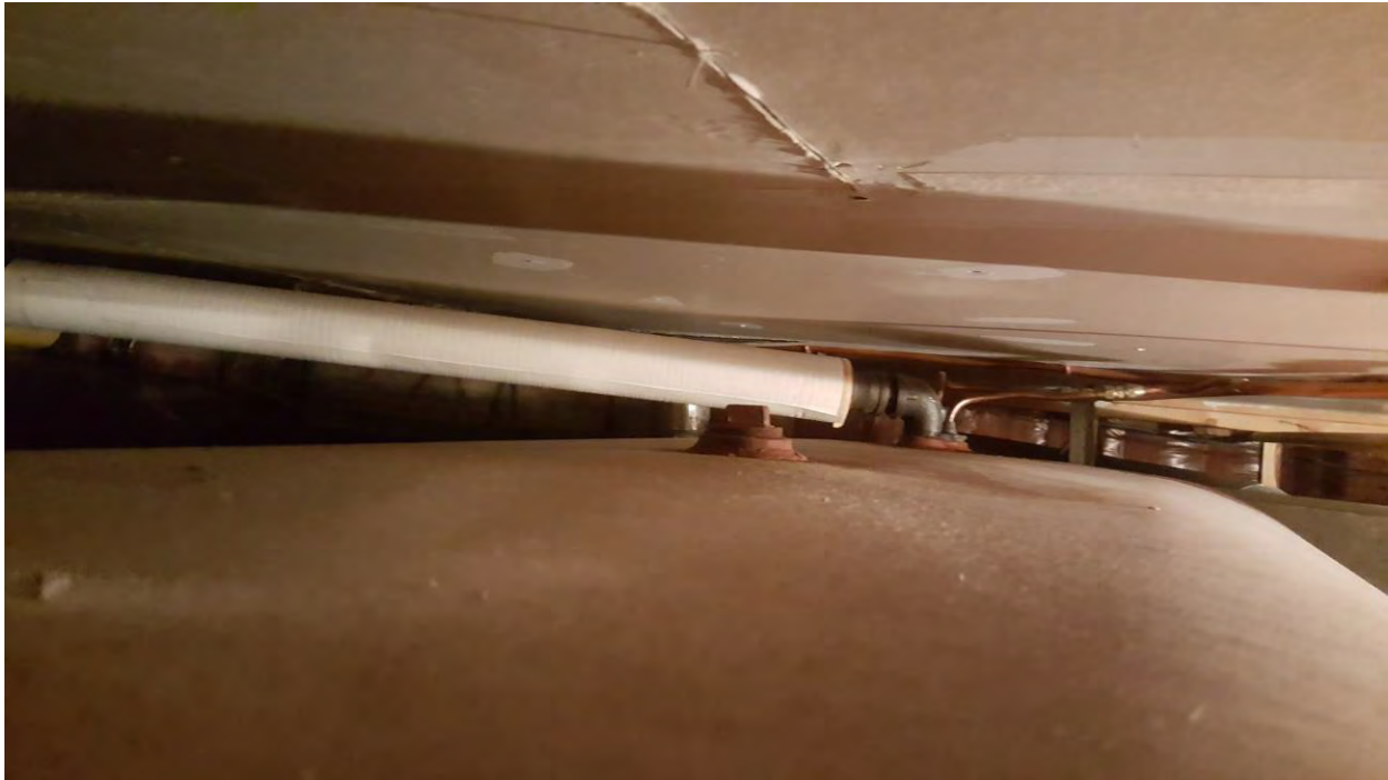
Photo 17 Interior Venting to be removed
