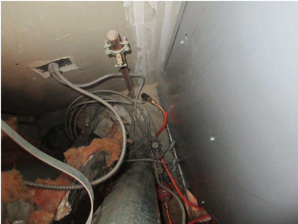
Photo 12 Furnace No.2 Piping
