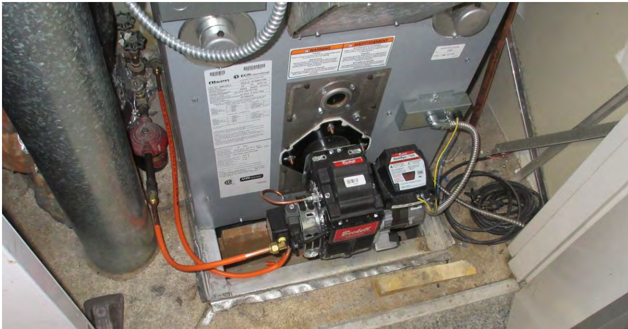
Photo 8 Furnace Room No. 1
