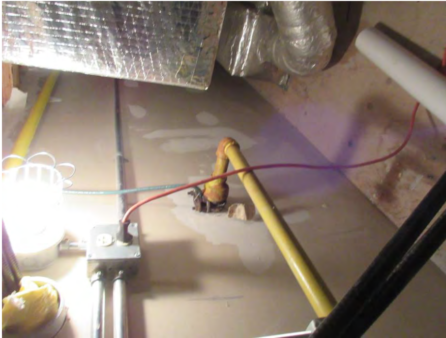
Photo 15 Crawl Space Entry Piping
