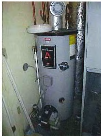
Photo 4: Indoor water heater
