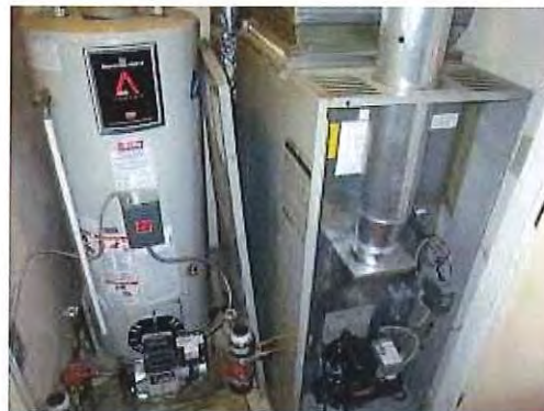
Photo 2: Interior furnace and water heater
