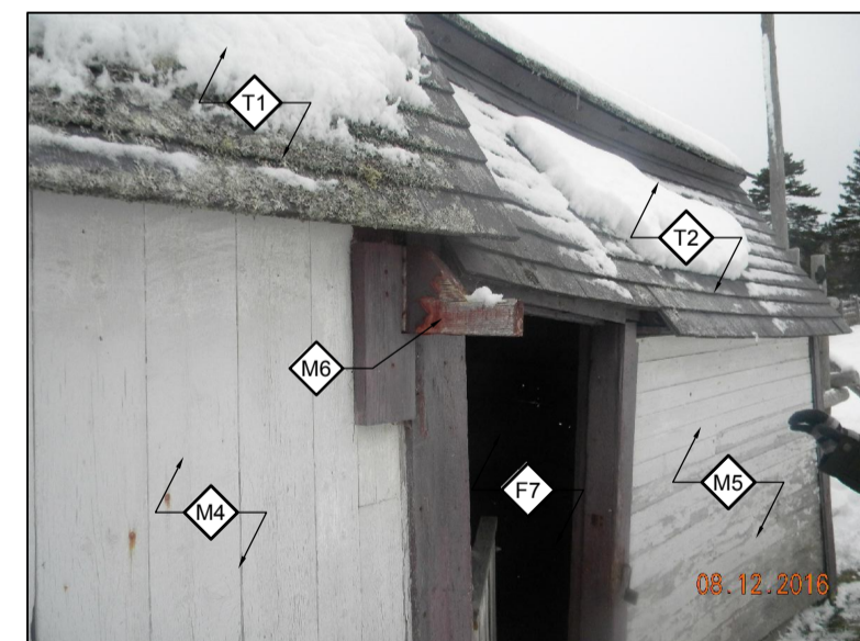
PHOTO 3 - GUTTER SUPPORT TO REPLACE
