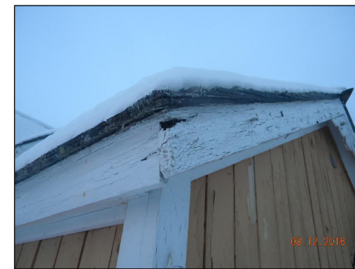
PHOTO 5 - FASCIA BOARD TO REPLACE
