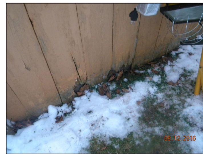
PHOTO 3 - WOOD SIDING DAMAGED WHERE IN TOUCH WITH GROUND
