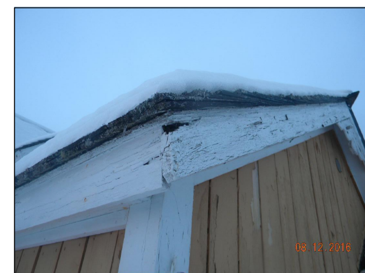
PHOTO 5 - FASCIA BOARD TO REPLACE
