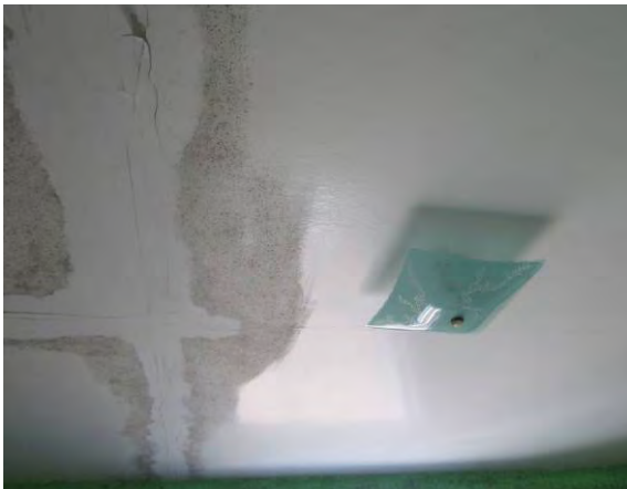
Photo 124: View of mould growth on ceiling in single dwelling bedroom #1.
