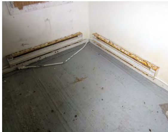
Photo 125: View of mould growth on walls in equipment building.
