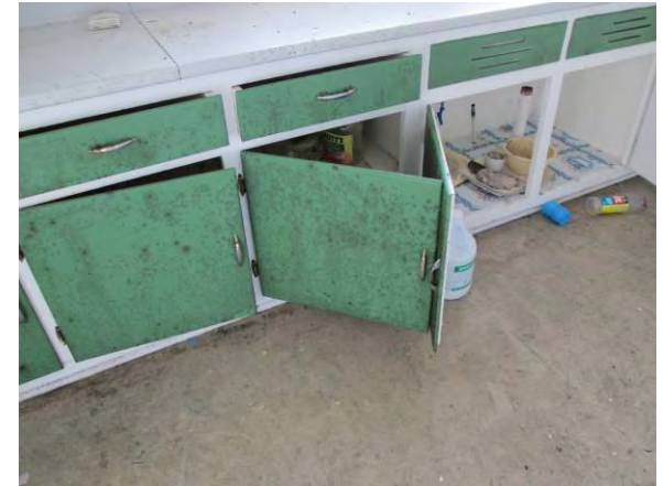
Photo 123: View of mould growth on cabinets in duplex kitchen.
