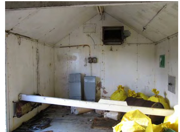
Photo 126: View of mould growth on walls, ceiling and floor in generator building.
