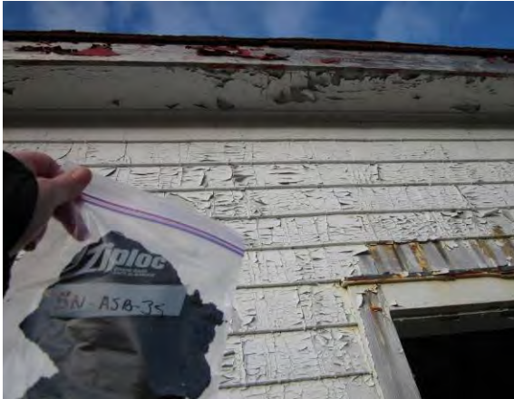
Photo 37: View of red asphalt shingle with felt/paper backing sample BN-ASB-35.
