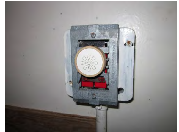
Photo 135: View of thermostat in equipment building.
