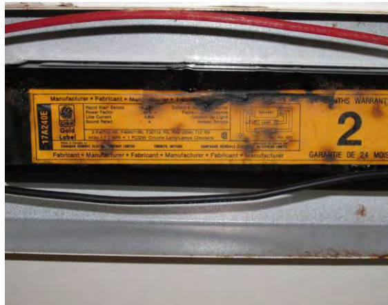
Photo 137: View of CGE Gold Label light ballast in equipment building.
