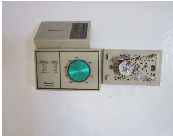
Photo 134: View of mercury tube in beige Honeywell rectangular thermostat.
