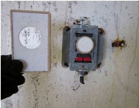
Photo 136: View of thermostat in generator building.
