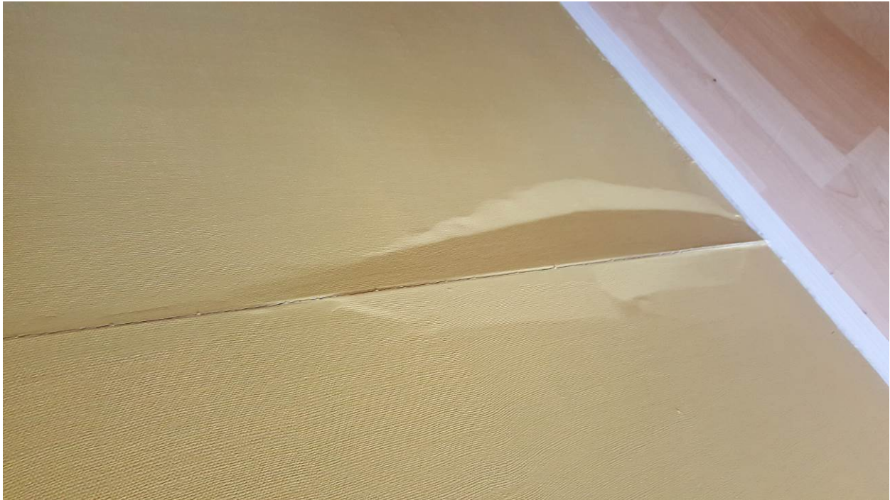
Photo 3 Damaged Vinyl Covered Drywall
