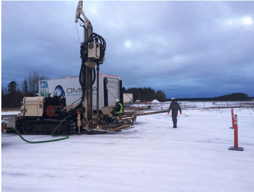
Photograph 1: Drilling performed by Omega using a Geoprobe 8140LS Sonic Track Drill Rig.
