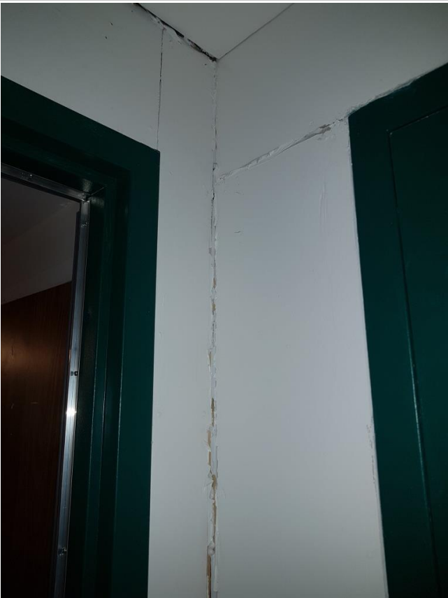
Photo 25 – Trailer, Separation at Porch/Trailer Walls and Ceiling
