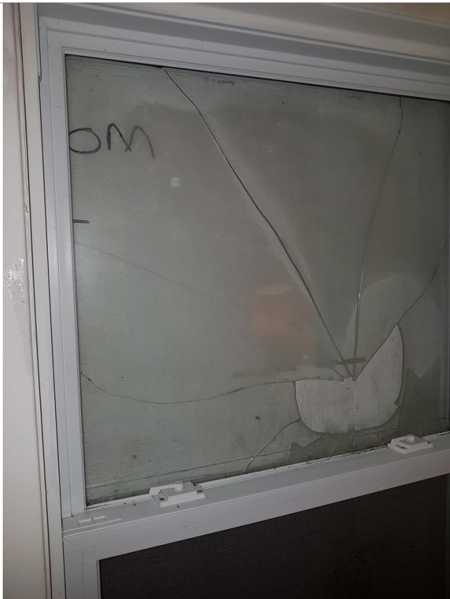
Photo 29 – Trailer, Broken Sealed Unit in Window (Window is Covered with Plywood on Exterior)
