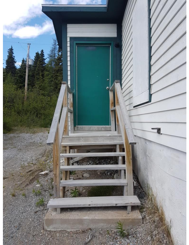
Photo 8 – Trailer, Step at Main Entrance to Porch
