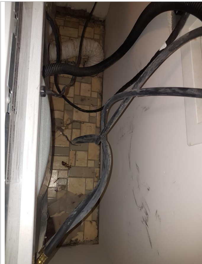
Photo 43 – Trailer, M&E Behind Laundry
