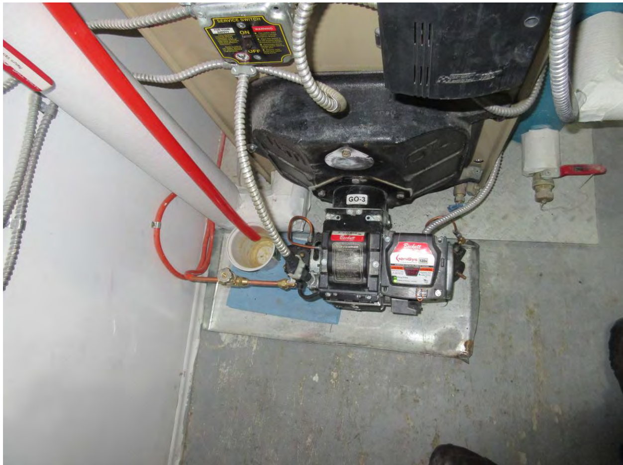
Photo 22 Fuel Line at Boiler
