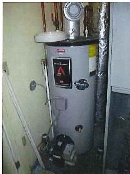
Photo 4: Indoor water heater
