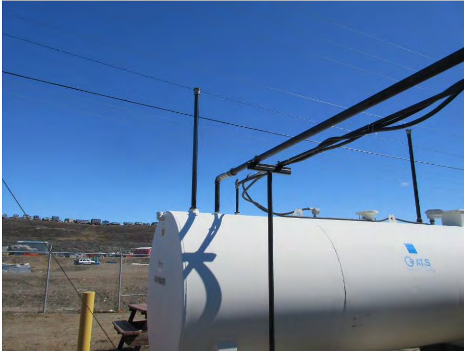
Photo 3 PIPING TO TANK
