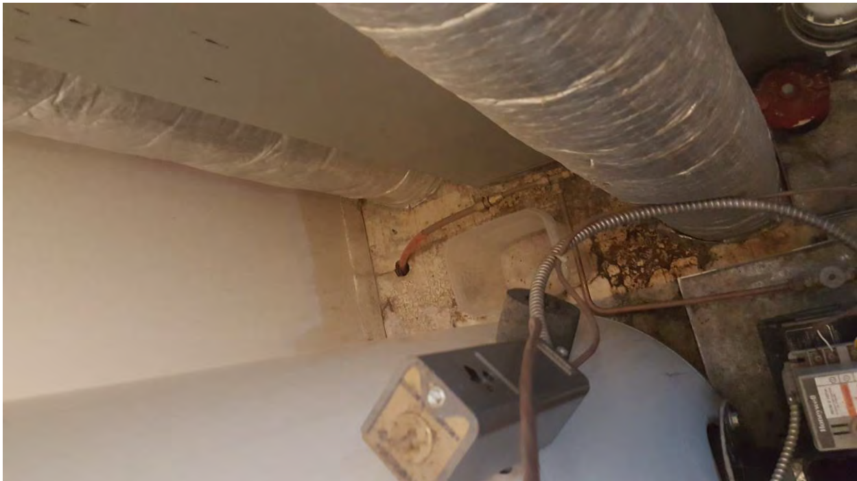
Photo 14 Piping from Crawl Space
