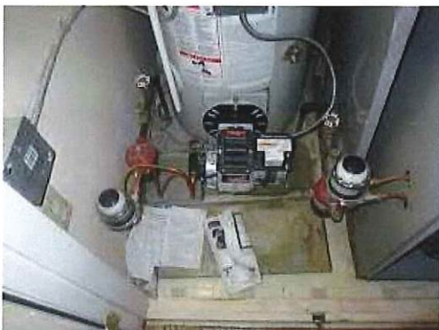
Photo 3: Interior piping and accessories
