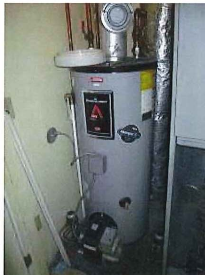
Photo 4: Indoor water heater
