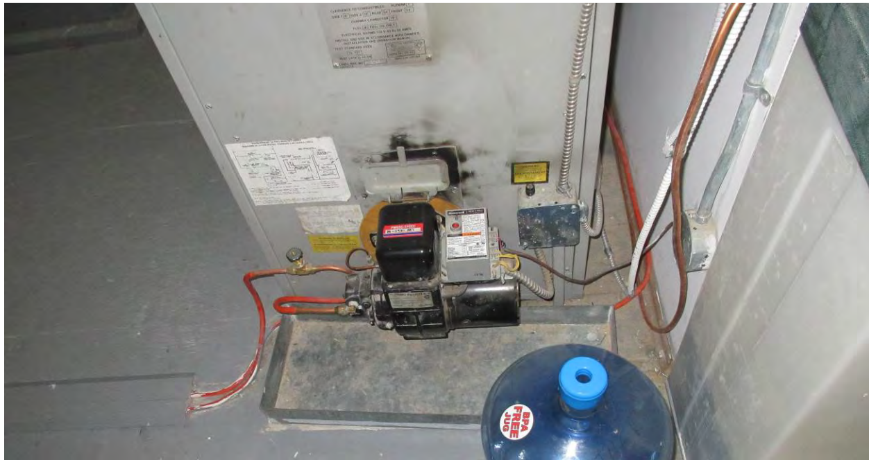
Photo 21 Fuel Lines at Furnace
