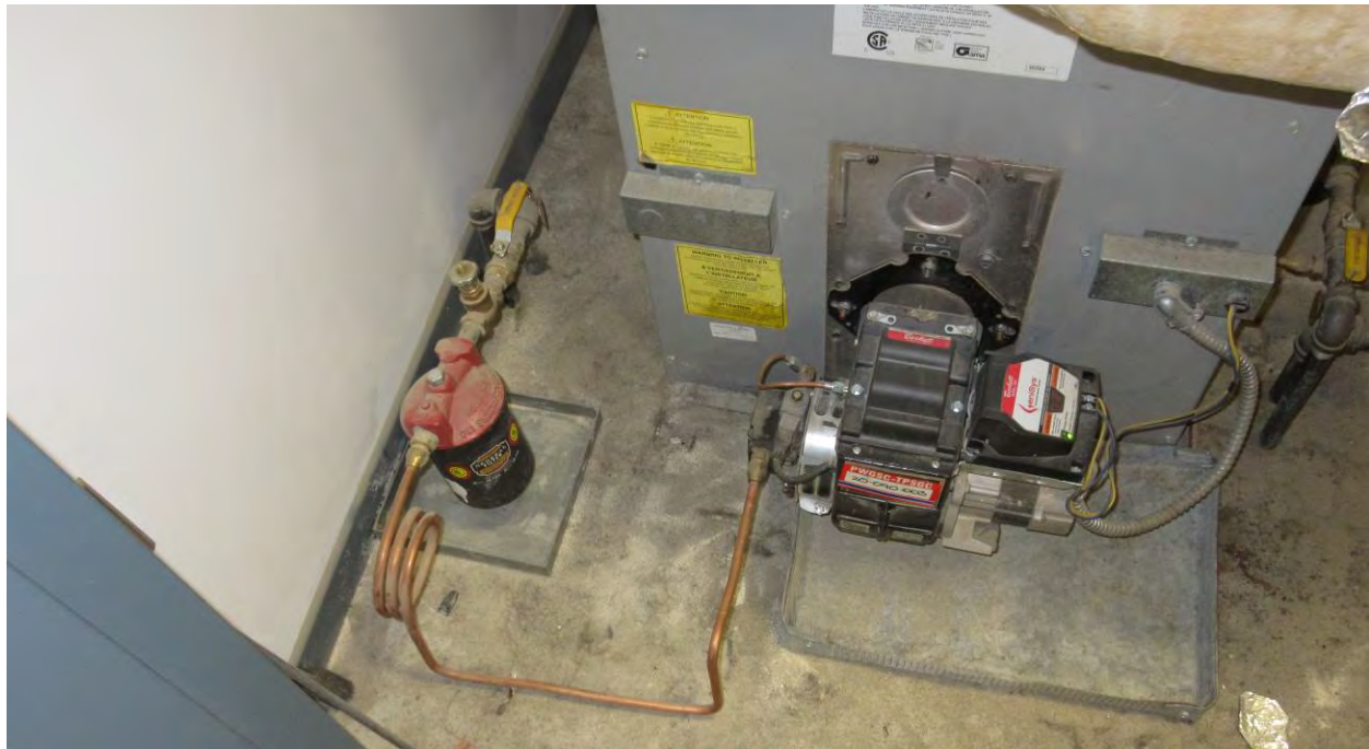
Photo 13 Furnace No. 3 Piping
