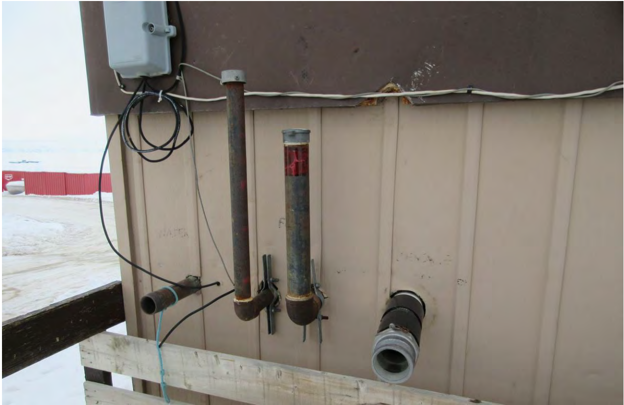
Photo 23 Exterior Fill Lines
