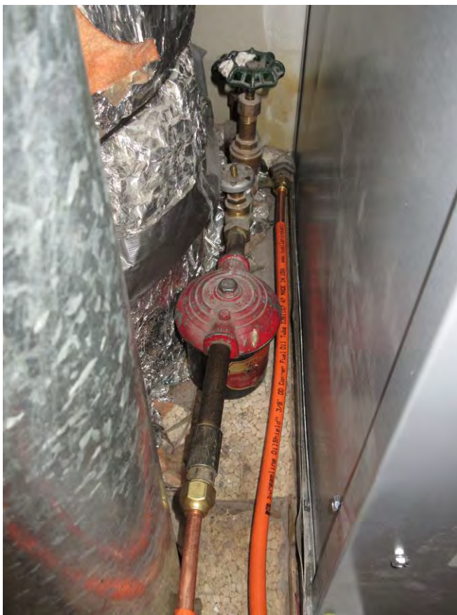
Photo 10 Furnace No. 1 Piping
