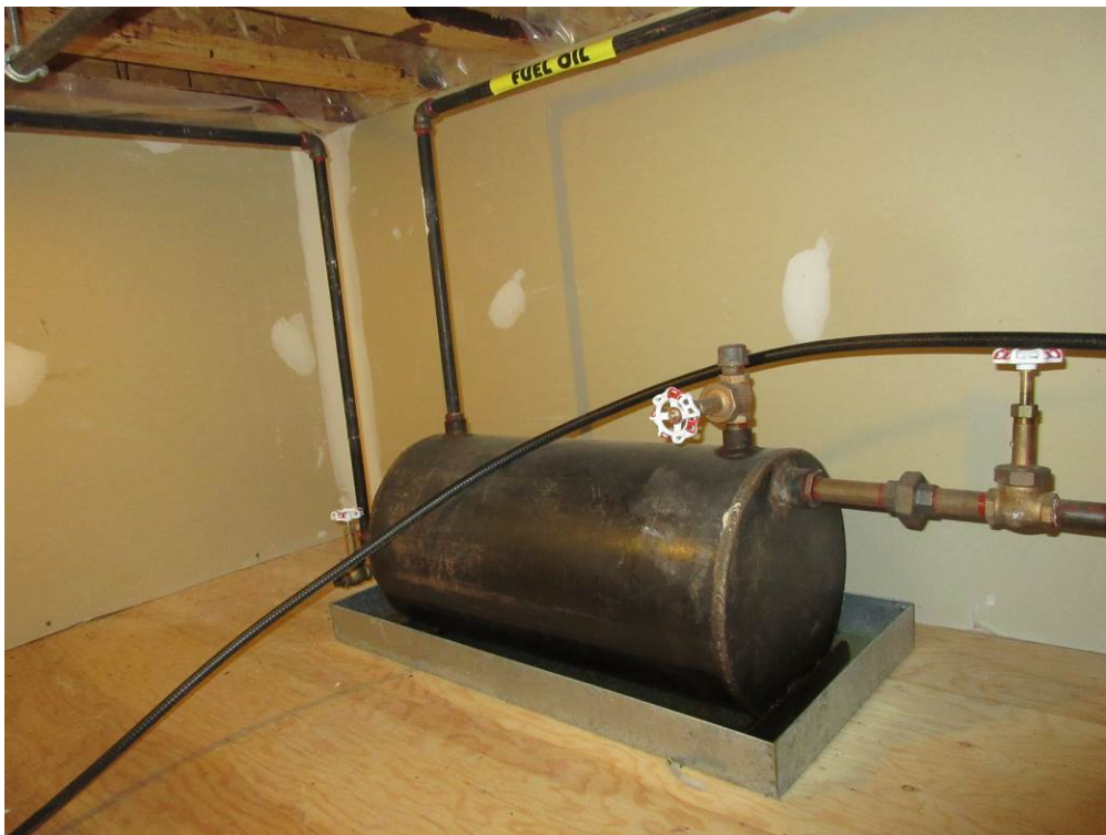
Photo 12 EXISTING GENERATOR DAY TANK
