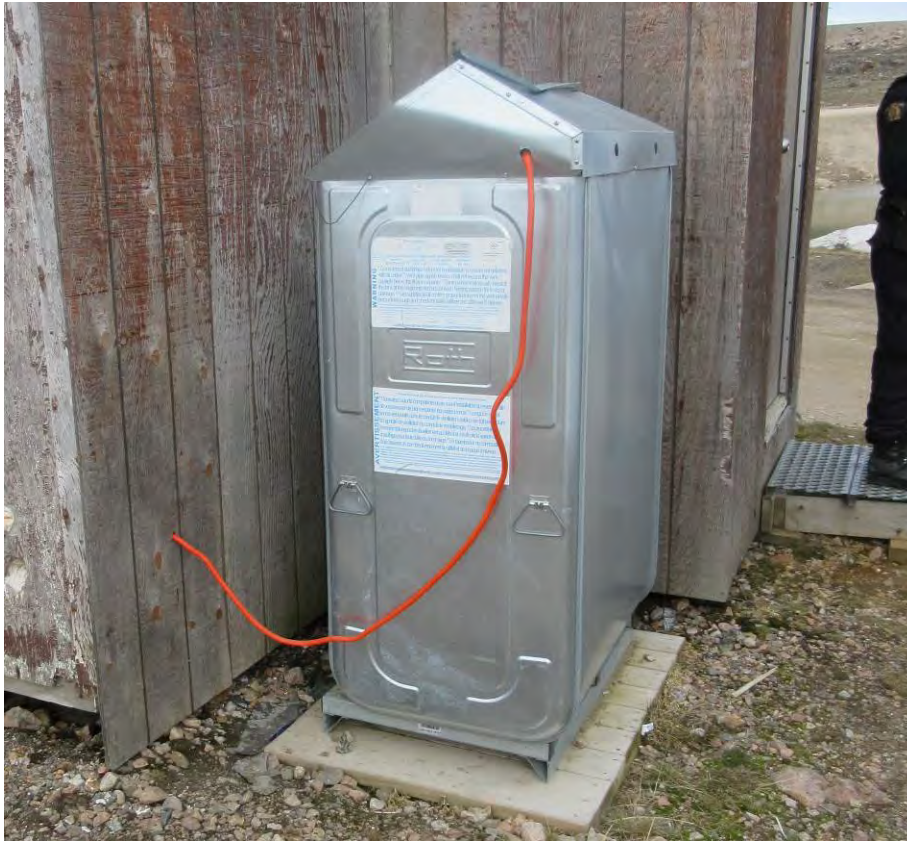
Photo 5 Existing Fuel Tank
