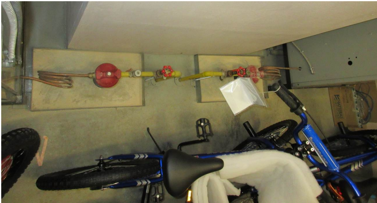
Photo 12 Interior Furnace 1 and 2 Piping
