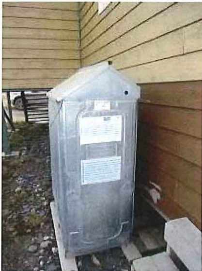
Photo 1: Outdoor above ground fuel tank
