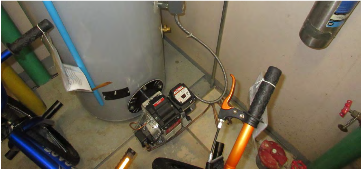
Photo 13 Hot Water Tank Fuel Piping
