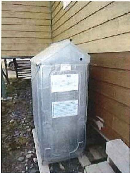
Photo 1: Outdoor above ground fuel tank
