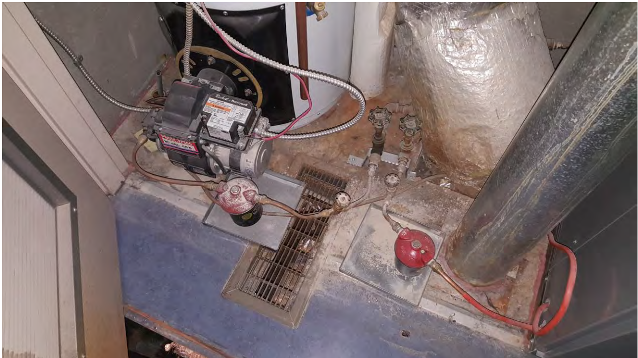
Photo 18 Hot water tank piping
