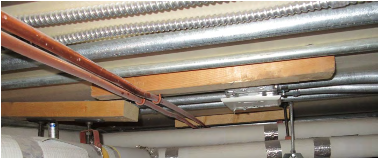
Photo 16 Crawl Space Piping to Furnaces 1 and 2
