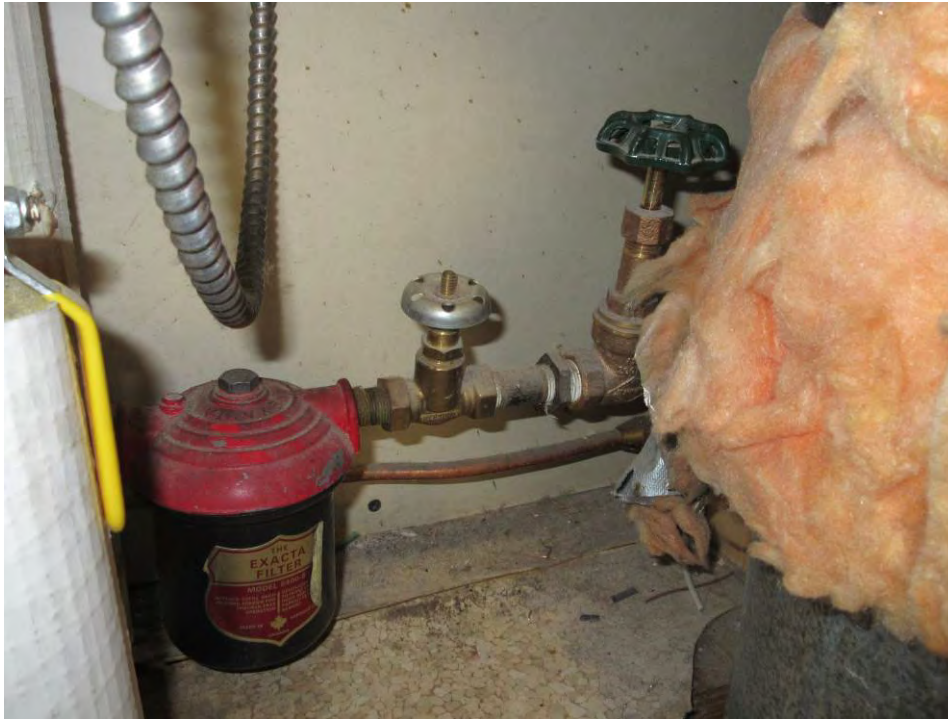
Photo 9 Furnace Room No. 1
