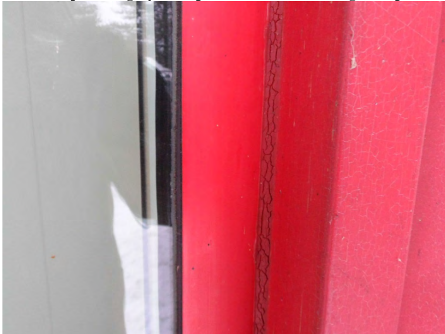
Photo 6: Main Building exterior red siding – Lead-containing (Sample Admin-P-29).
