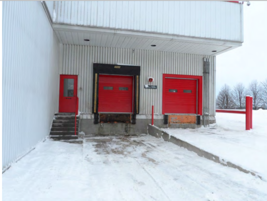
Photo 3: Main Building exterior red trim paint–Lead-containing (Sample Admin-P-29).
