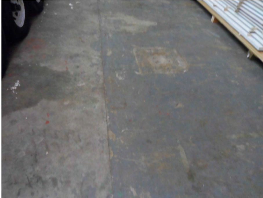
Photo 5: Ship stores grey floor paint – Lead-containing (Sample SHP-P-27).
