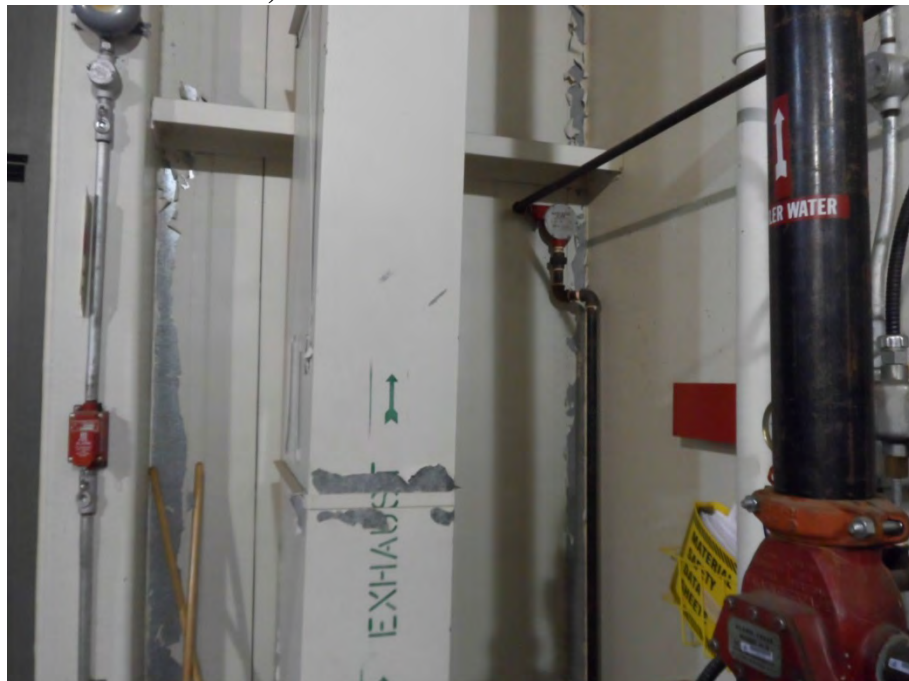
Photo 4: Hazard Storage Building cream interior wall paint – Lead-containing (Sample Haz-P-25).
