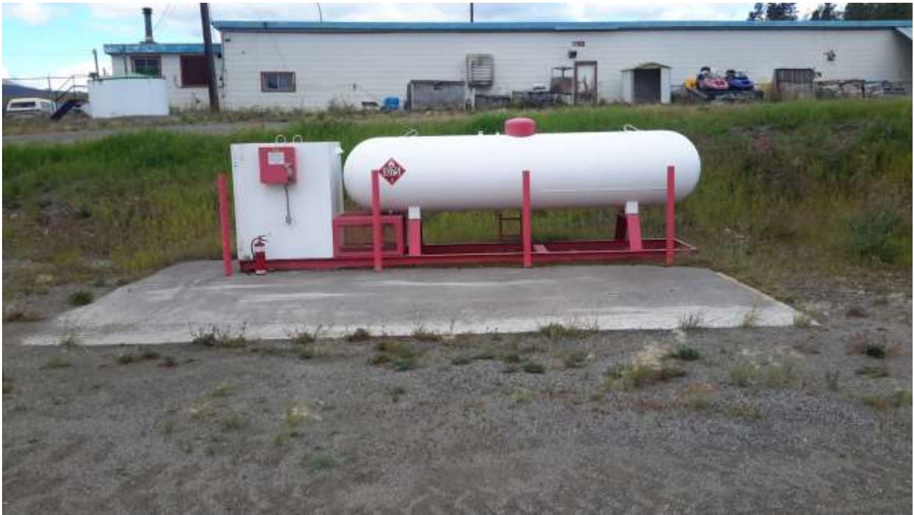
Photo 2: View of the propane tank in the 'Base Work' area. Concrete pad has dimension of 2.4 x 1.8m (8 x 6 feet).
