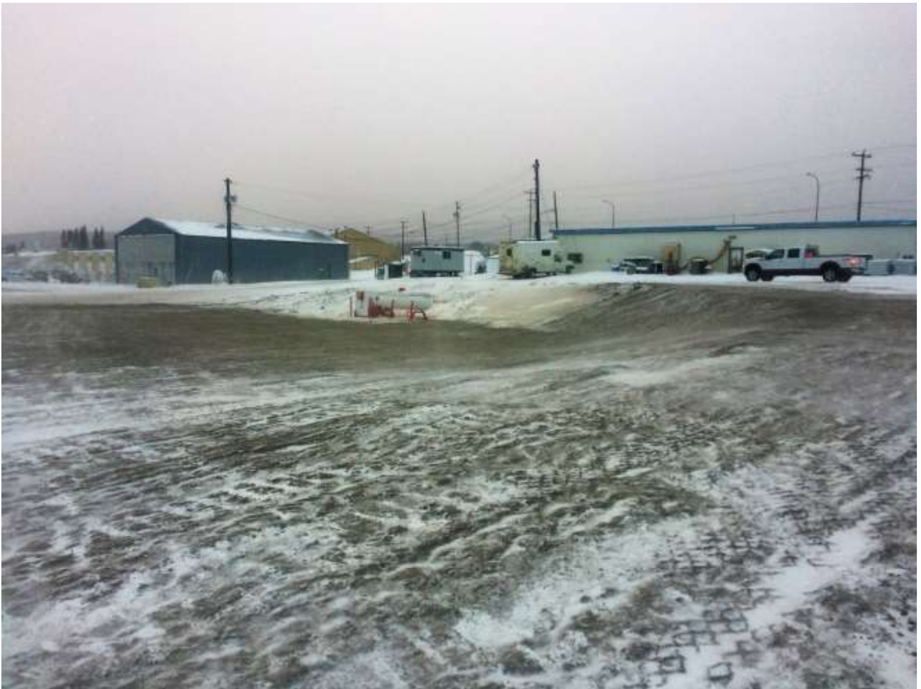
Photo 1: Propane tank and view of the base work area. Camera facing southwest.
