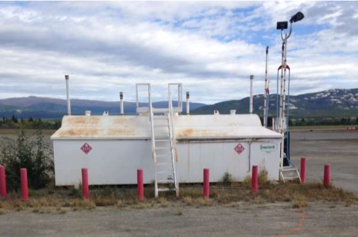
Photo 3: Fuel AST in the 'Optional Work' area. No concrete pad.
