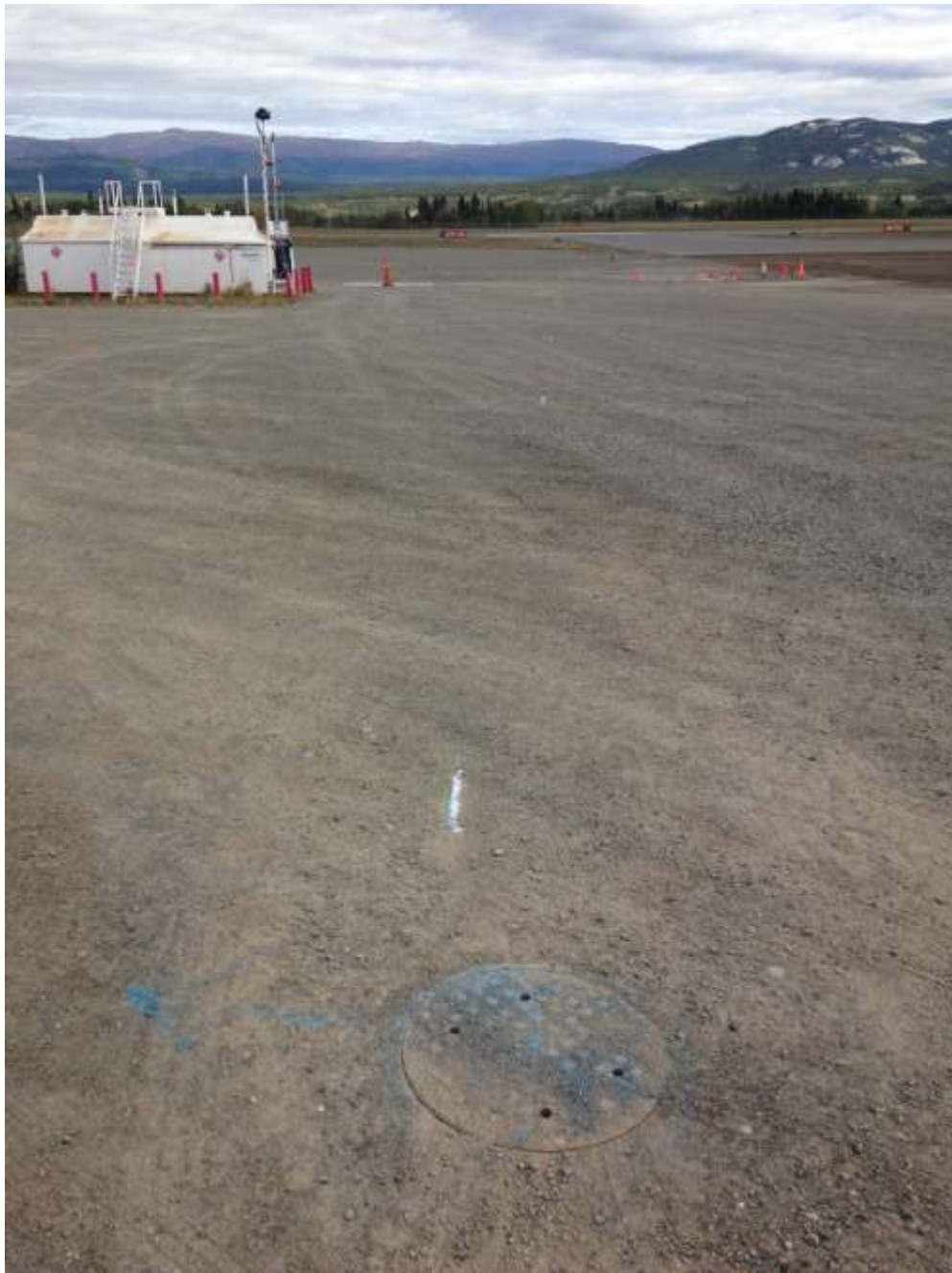
Photo 5: Man hole and sani dump in the background showing general alignment of sanitary sewer.
