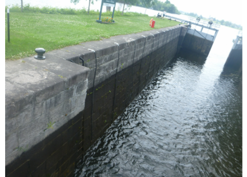
PHOTO O7 SCALE: NTS S03 LOCK WALL SHOWING HORIZONTAL JOINTS, AT TOP OF WALL
