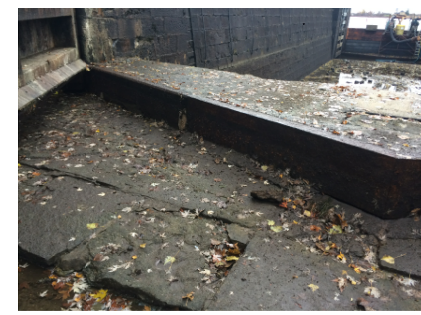
PHOTO O4 SCALE: NTS S03 DAMAGED FLAGSTONES
