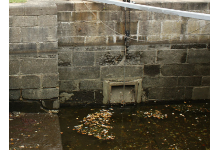
PHOTO O6 SCALE: NTS S03 BADLY DAMAGED WEST WALL AT SLUICE TUNNEL
