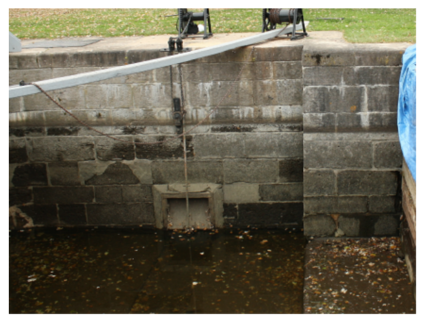
PHOTO O5 SCALE: NTS S03 BADLY DAMAGED EAST WALL AT SLUICE TUNNEL
