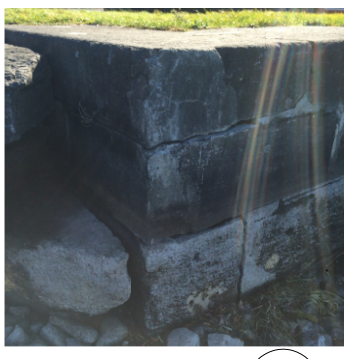
PHOTO 11 SCALE: NTS CONCRETE RETAINING WALL AND DRYSTACK STONE CAP TO BE REPAIRED.
