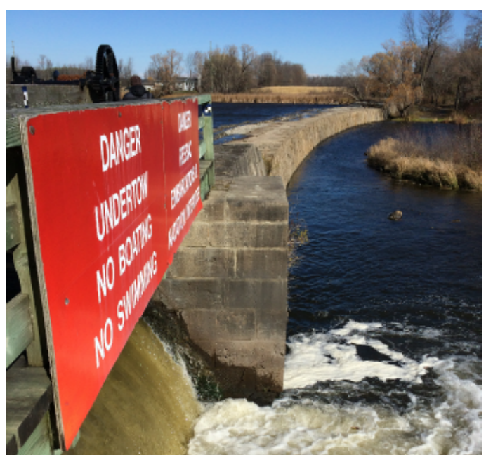
PHOTO 08 SCALE: NTS DOWNSTREAM WEIR WALLS TYPICAL DAMAGE AND WINTER WATER FLOW
