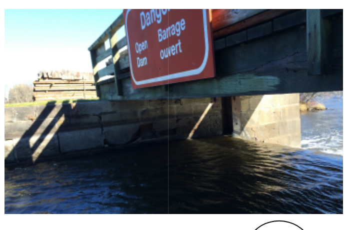
PHOTO 07 SCALE: NTS DAMAGE AT WEIR
