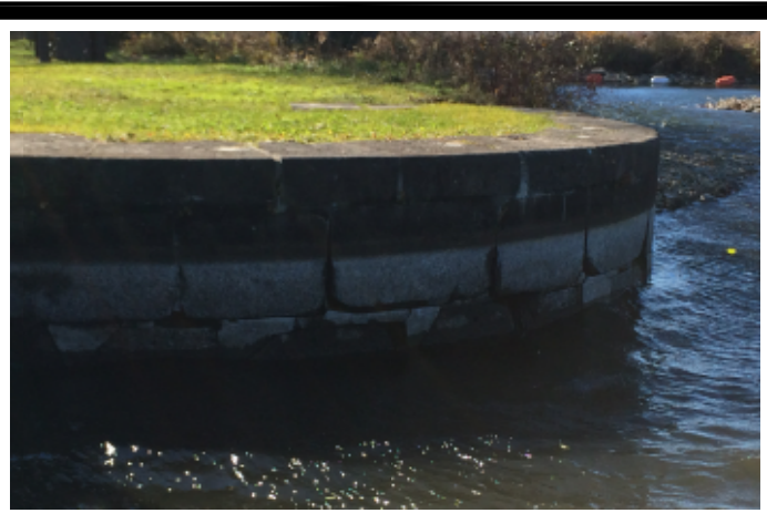
PHOTO 06 SCALE: NTS WEIR NW WALL TYPICAL STONE CONDITION
