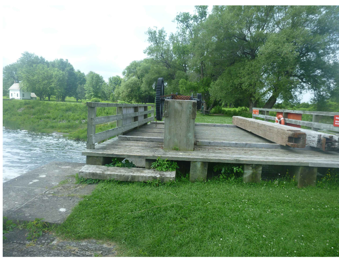
PHOTO 06 SCALE: NTS EXISTING WEIR TIMBER STRUCTURE. TIMBER FRAMED LOG HOIST TO REMAIN. TIMBER LOG SLIDES TO BE REPLACED, AS SHOWN ON DETAILS 01 THROUGH 05/S06.
