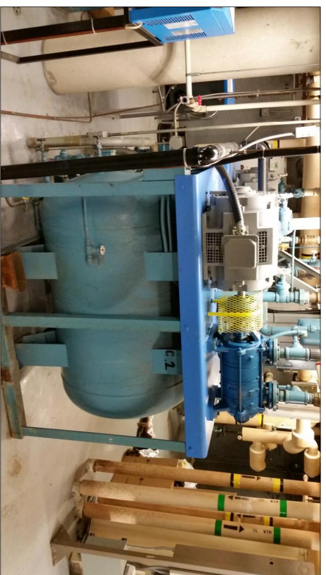
EXISTING DUPLEX AIR COMPRESSOR TO BE REMOVED
