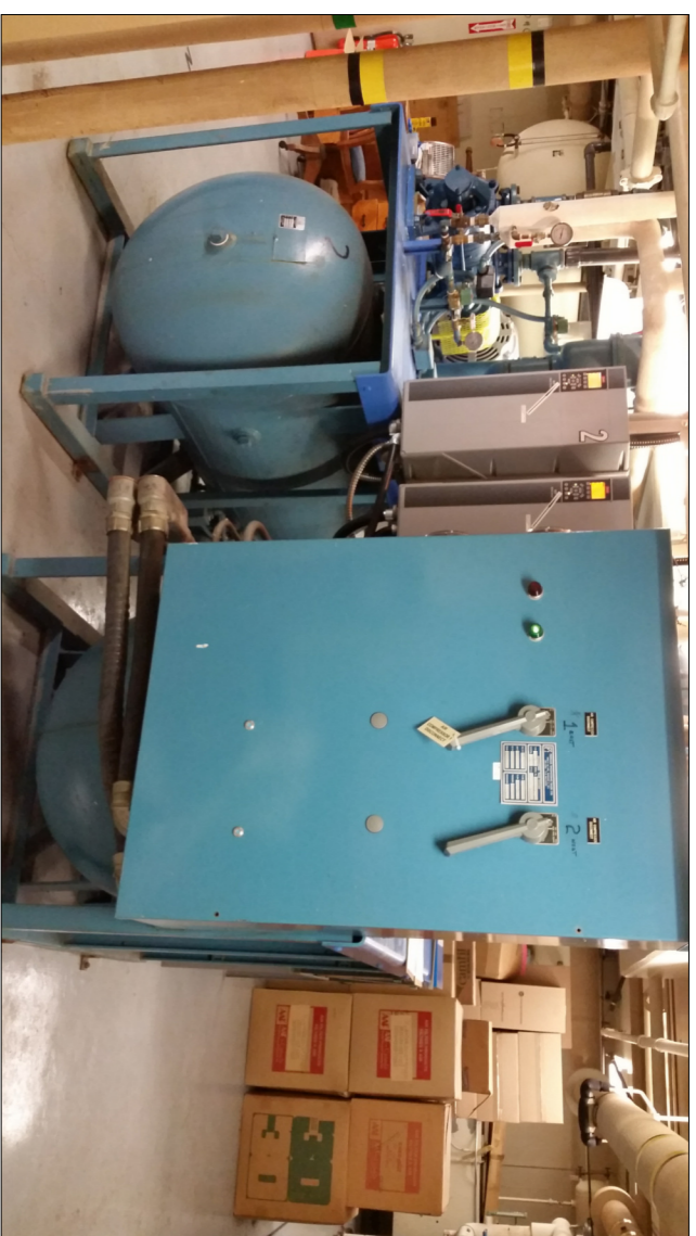
EXISTING DUPLEX AIR COMPRESSOR TO BE REMOVED
