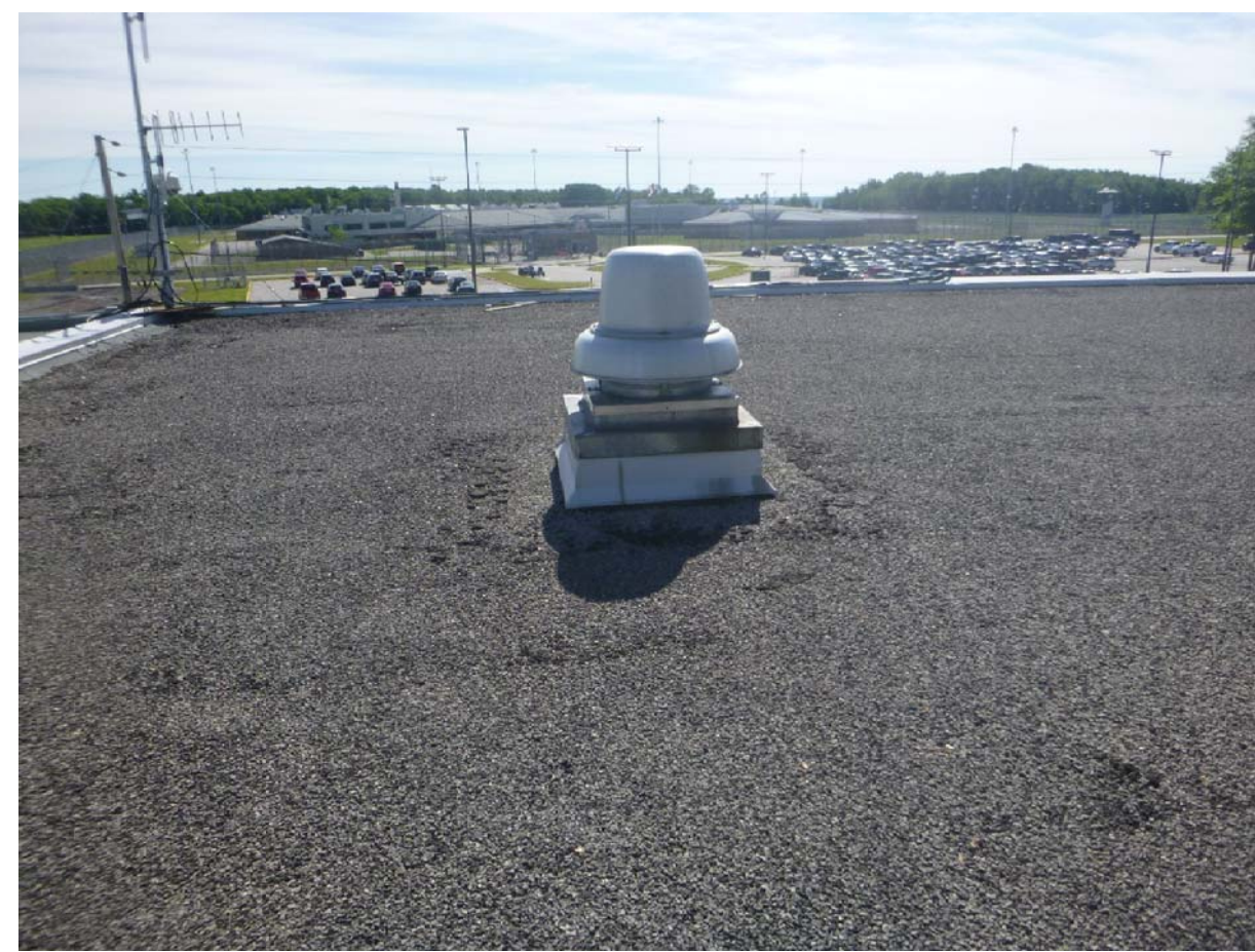
06 PICTURE - EXISTING MECHANICAL BASE SCALE: NONE
