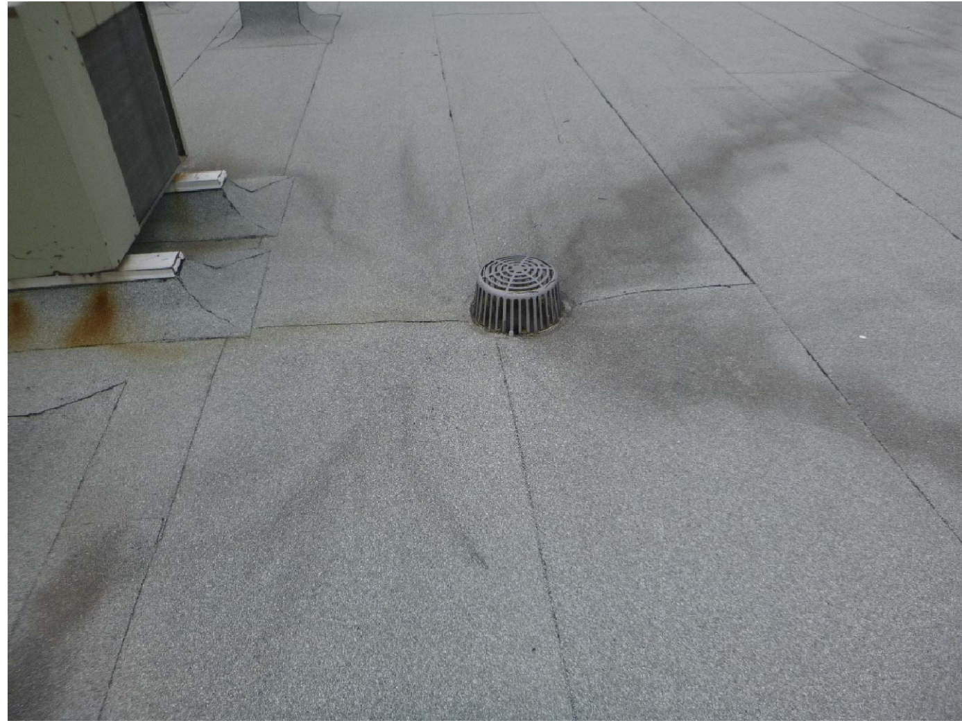
02 PICTURE - ROOF DRAIN SCALE: NONE
