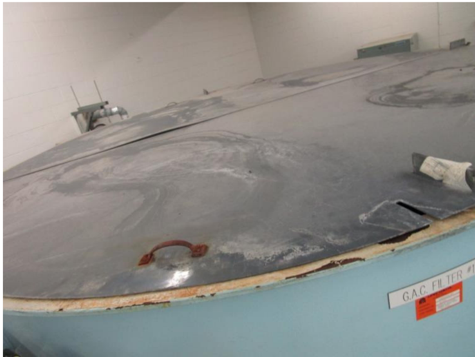
Photo 3: GAC tank cover
