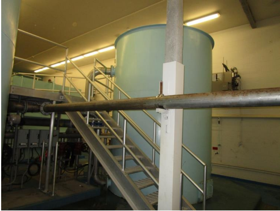
Photo 1: GAC tank #1 and platform
