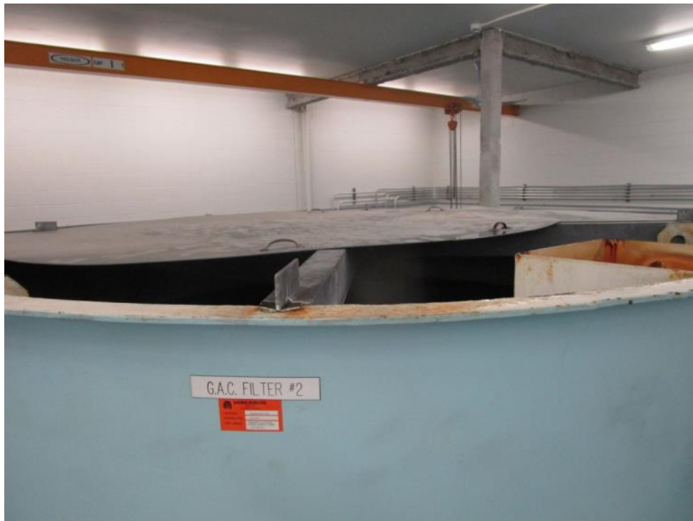
Photo 4: Cover partially opened showing cover frame and adjustable influent weir
