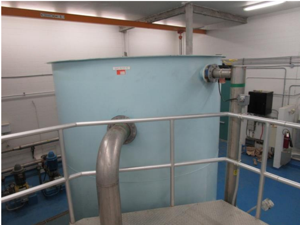
Photo 2: Top Section of GAC Tank #2
