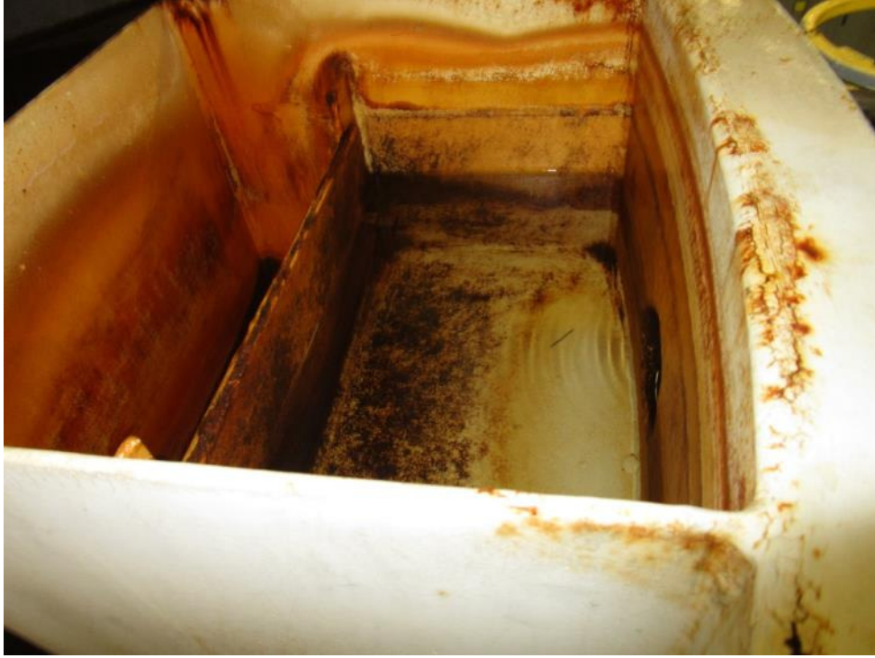
Photo 5 – Adjustable influent weir
