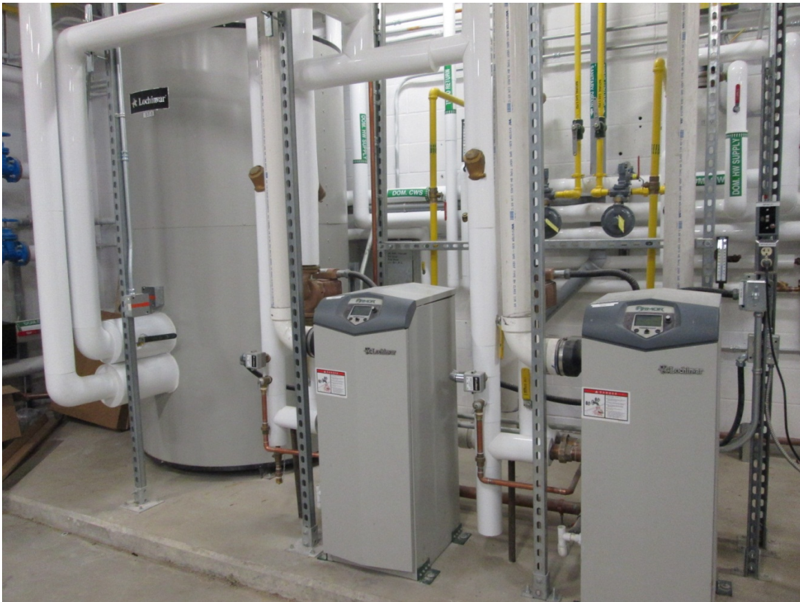
Fig. 9: Domestic Water Heaters and Storage Tank
