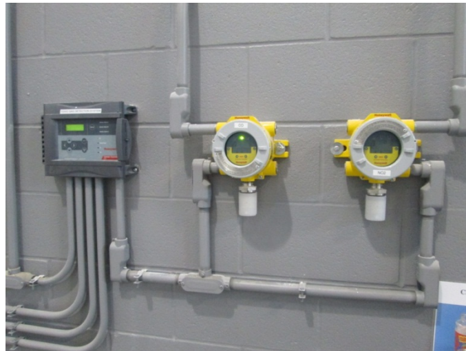
Fig. 58: Gas Detection Alarm Controller, CO & NOx Detectors
