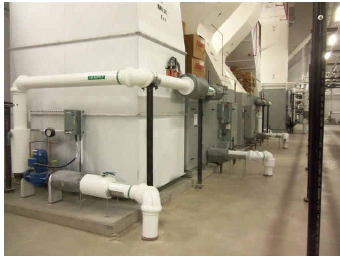
Fig. 28: Energy Recovery Units 2A & 2B (AHU5 in background)
