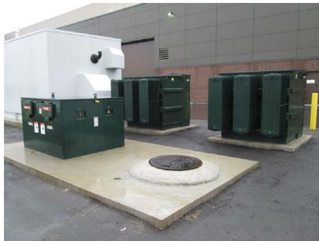
Fig. 39: Switchgear and Transformers
