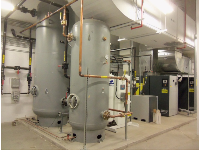
Fig. 12: Compressed and Breathing Air Plant
