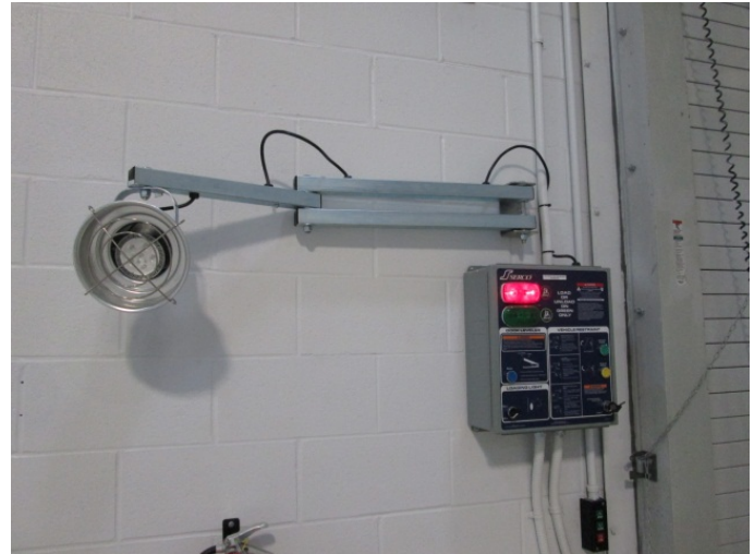
Fig. 4: Loading Dock Controller
