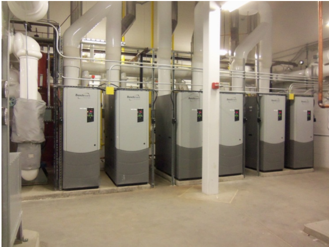
Fig. 23: High Temp Boiler Plant
