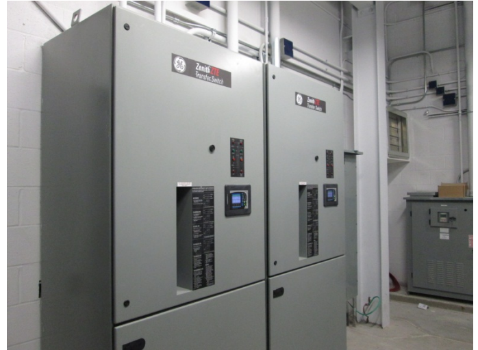
Fig. 50: Automatic Transfer Switches
