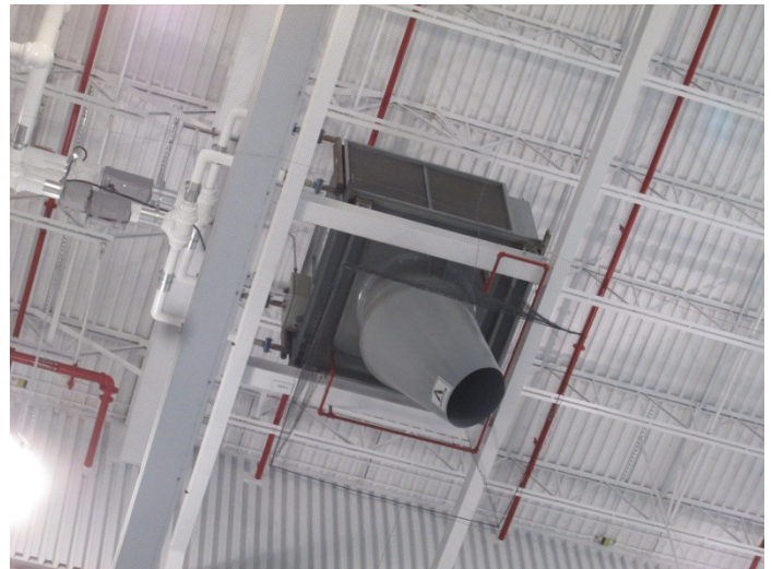
Fig. 32: Vertical Unit Heater
