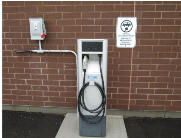
Fig. 53: Electric Vehicle Charging Station
