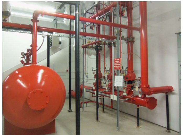
Fig. 8: HEF Tank, Foam Header and Proportioning Valves
