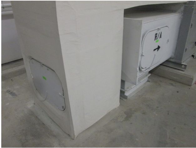
Fig. 16: AHU3 Fire Dampers with Verification Stickers Applied
