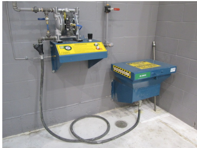
Fig. 14: Waste Oil Collector
