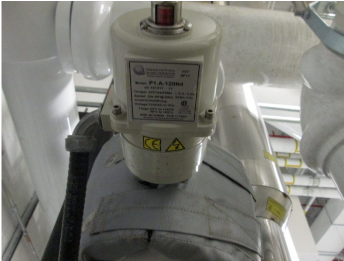
Fig. 64: Boiler Isolation Valve
