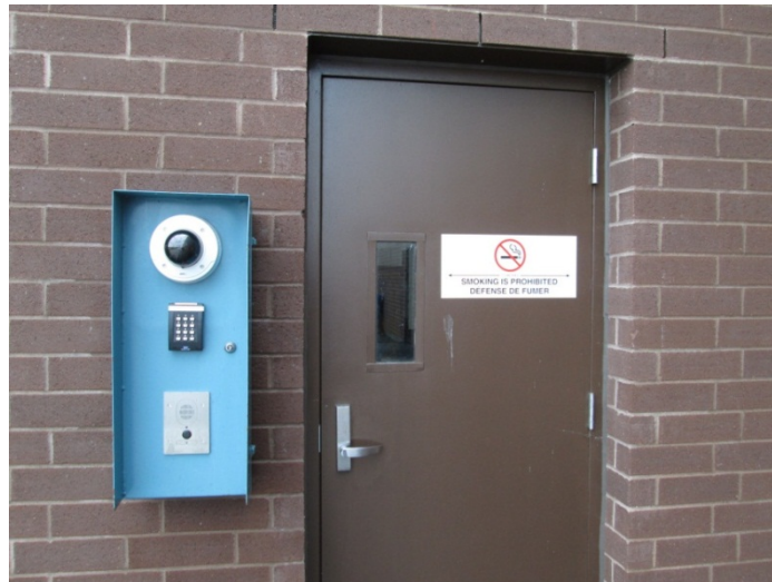
Fig. 60: Access Control Point
