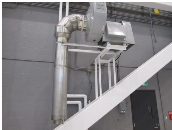
Fig. 21: Fuel Cell Exhaust Fan
