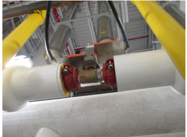
Fig. 65: Boiler Bypass Valve
