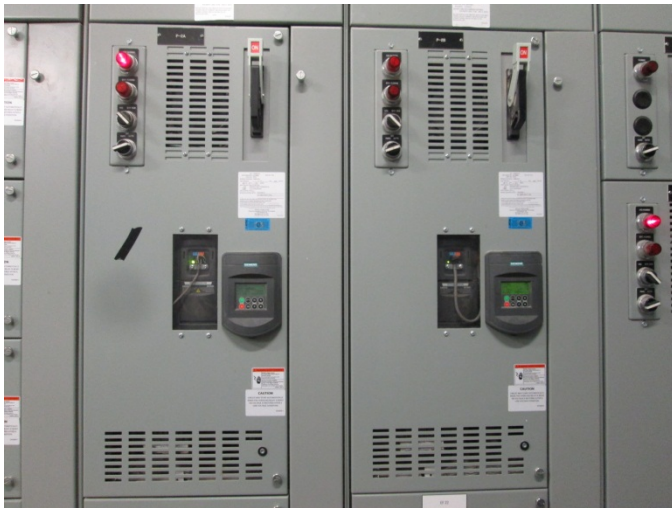
Fig. 45: Variable Frequency Drives for Pumps
