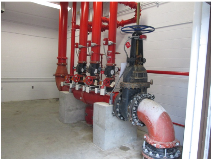
Fig. 7: Fire Water Entrance
