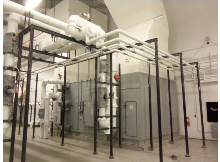
Fig. 27: Air Handling Unit 5
