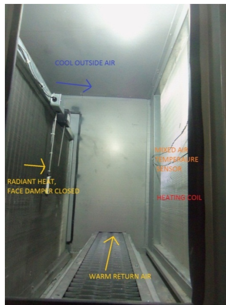
Fig. 67: AHU6 Mixing Section
