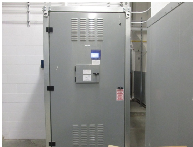
Fig. 42: Active Harmonic Filter
