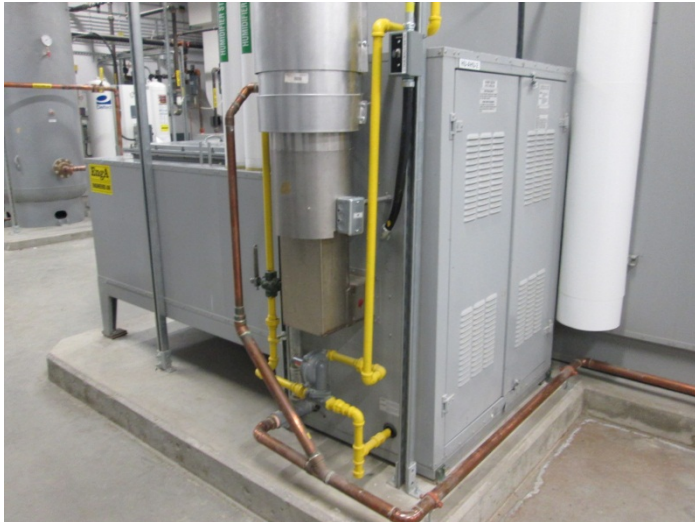
Fig. 33: Gas Fired Humidifier, HUH2
