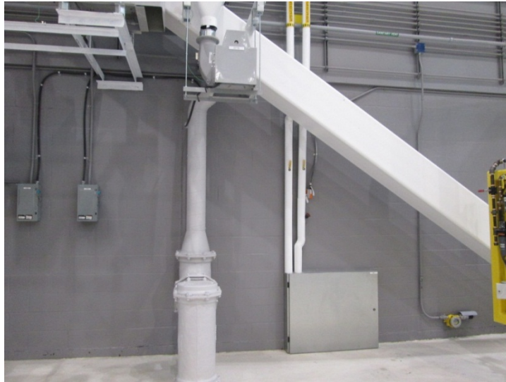
Fig. 20: Trench Drain Ventilation Unit
