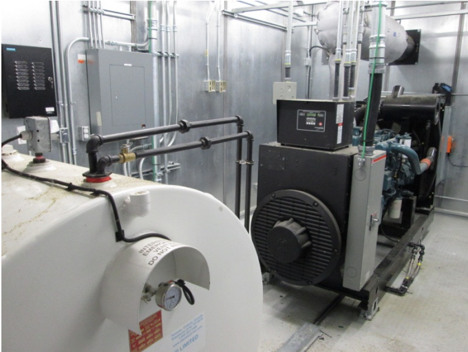
Fig. 49: Generator and Fuel Tank
