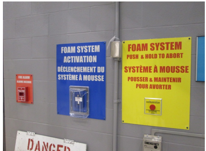
Fig. 55: Fire and Foam Pull Stations, Foam Abort Station
