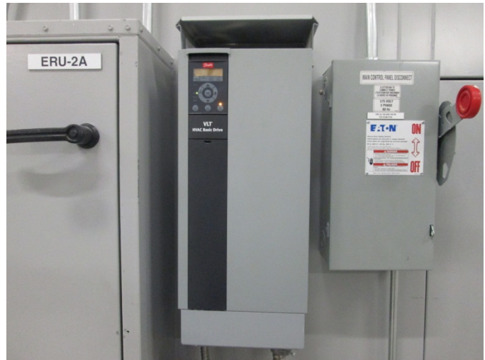
Fig. 46: Variable Frequency Drive for AHU Fan
