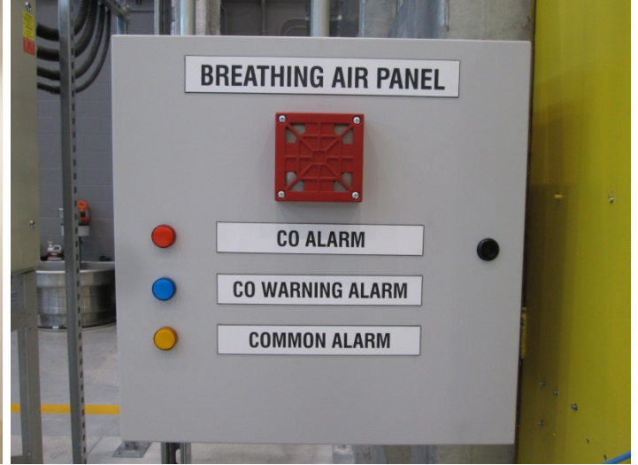
Fig. 13: Remote Breathing Air Alarm Station
