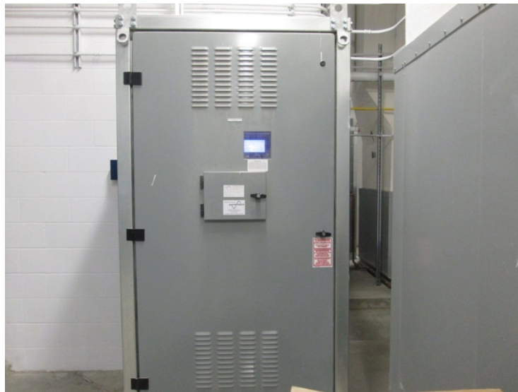
Fig. 42: Active Harmonic Filter
