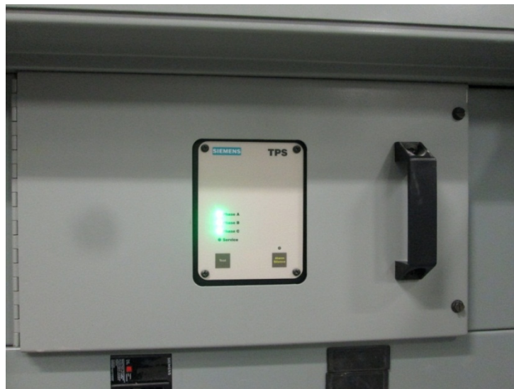
Fig. 44: Surge Protection Device
