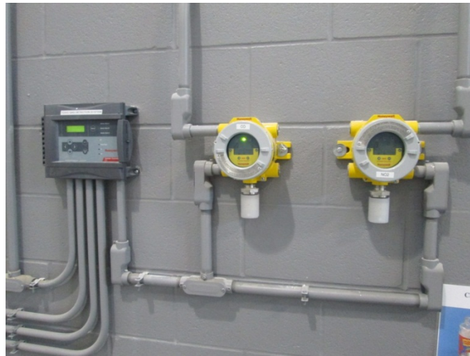
Fig. 58: Gas Detection Alarm Controller, CO & NOx Detectors
