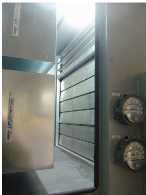
Fig. 66: Heat Pipe Face Damper Closed, Bypass Open
