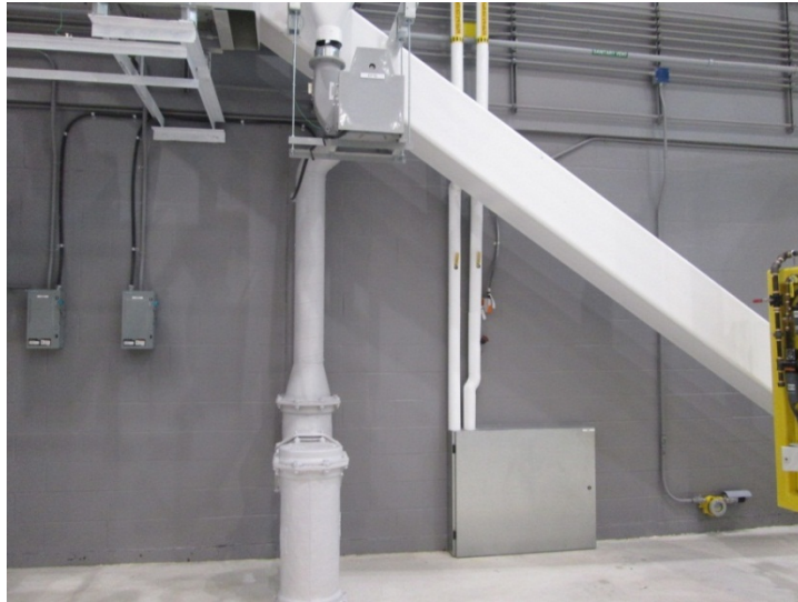
Fig. 20: Trench Drain Ventilation Unit
