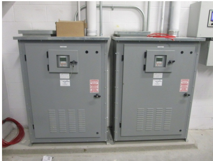
Fig. 43: Power Factor Correction Units
