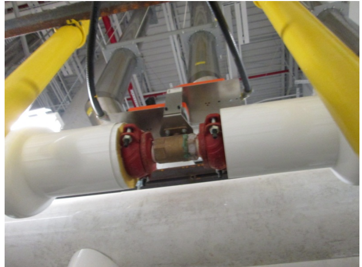
Fig. 65: Boiler Bypass Valve
