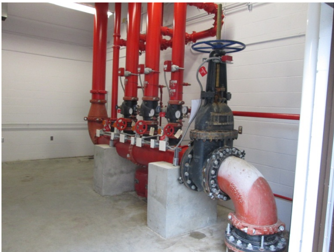
Fig. 7: Fire Water Entrance
