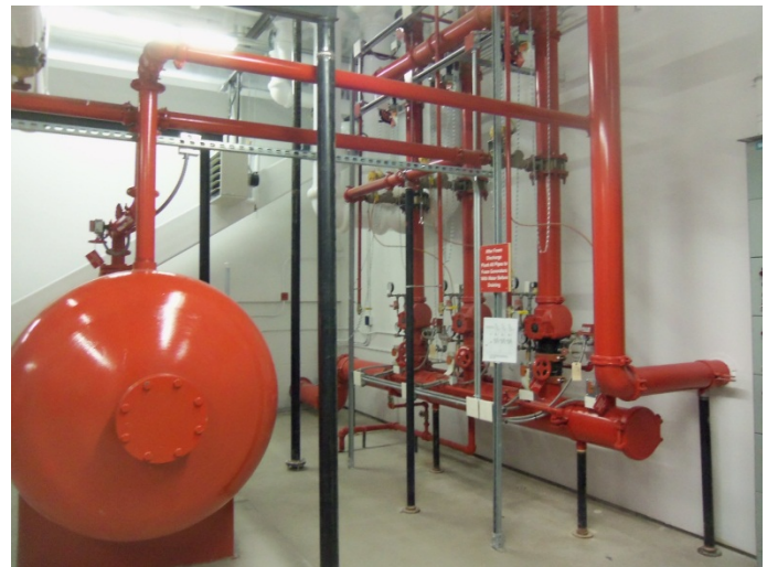
Fig. 8: HEF Tank, Foam Header and Proportioning Valves
