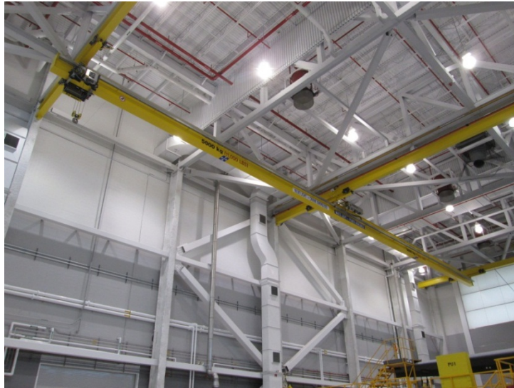
Fig. 62: Hangar Bay Bridge Crane
