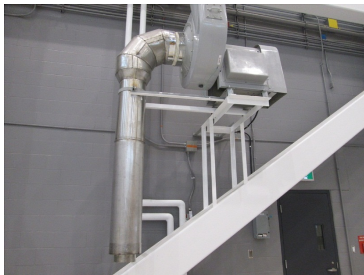
Fig. 21: Fuel Cell Exhaust Fan
