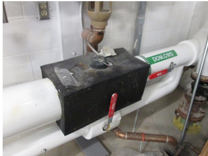
Fig. 15: Domestic Water Meter
