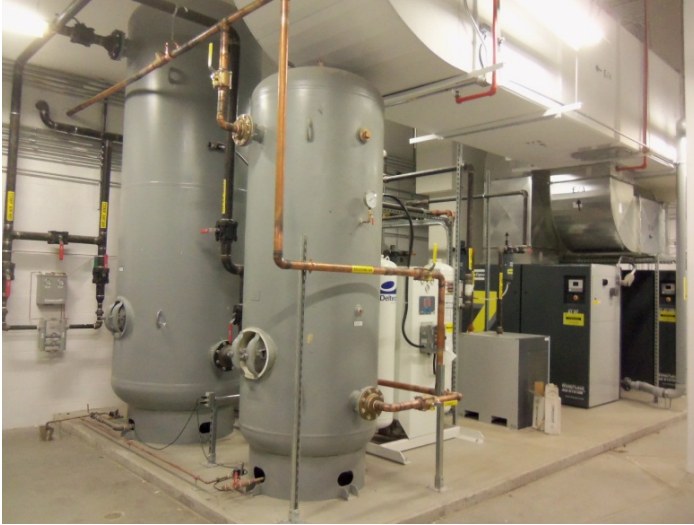
Fig. 12: Compressed and Breathing Air Plant
