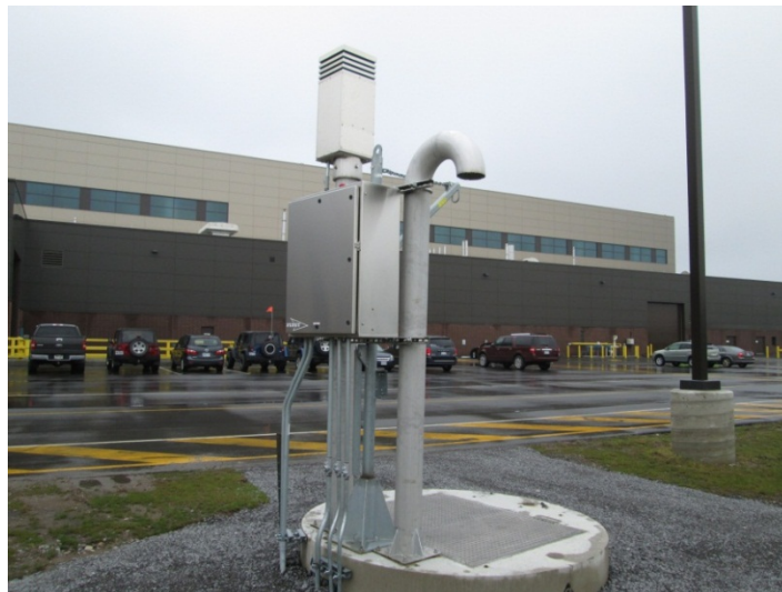
Fig. 61: Sewage Lift Station
