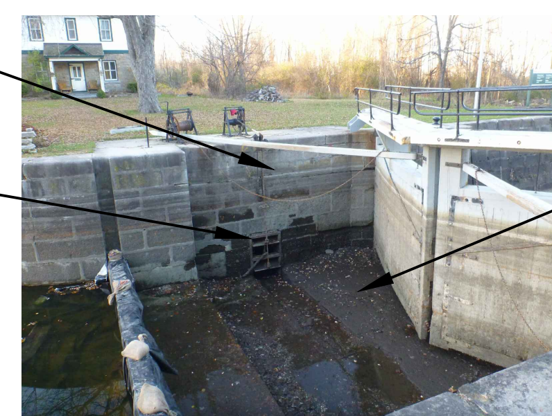
PHOTO 29 SCALE:NTS CONCRETE PAD TO BE REPAIRED
