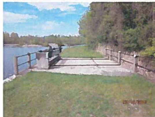
Figure 6 - Minnow Creek Waste Weir before the earth dam and weir were rebuilt in 2015.
