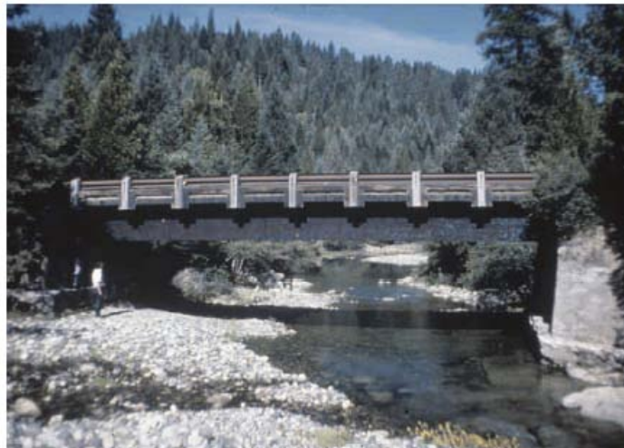
Figure 4.2 Oilborne preservatives are often used for treatment of glulam beams, such as in this bridge (Lebow and Tippie, 2001).
