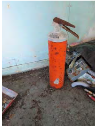
Photo 182: View of fire extinguisher in standby diesel building.
