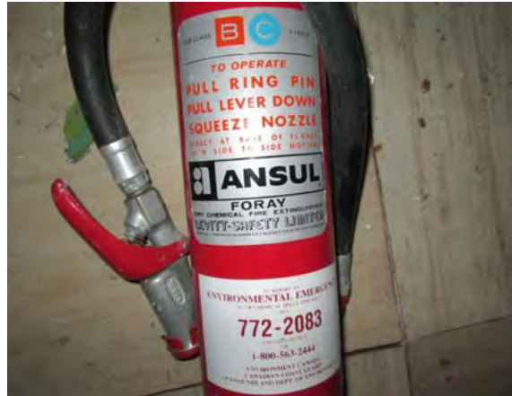
Photo 176: View of fire extinguisher in duplex dwelling kitchen.
