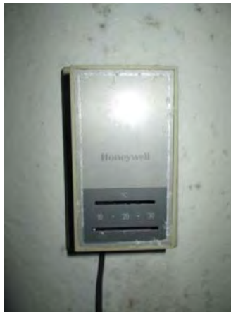
Photo 167: View of rectangular Honeywell thermostat (mercury-containing).
