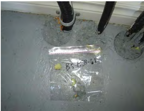
Photo 64: View of yellow/orange insulation sample BS-ASB-61.
