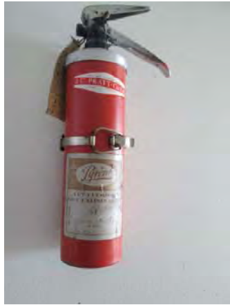
Photo 181: View of fire extinguisher in single dwelling hallway.
