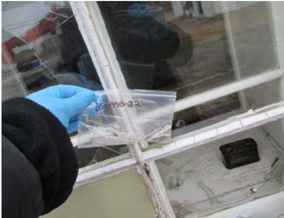
Photo 25: View of window caulking sample BS-AS-22.
