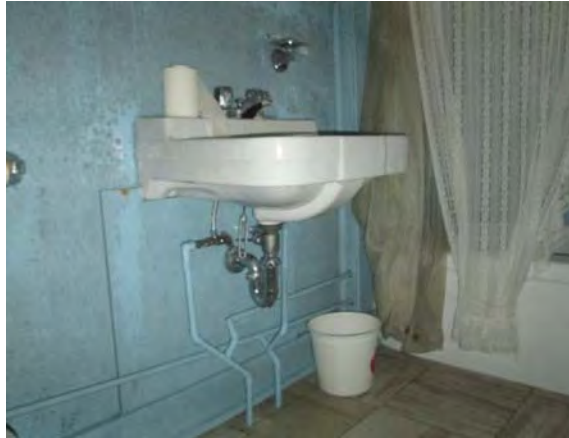
Photo 164: View of suspected visible mould growth in duplex dwelling washroom.
