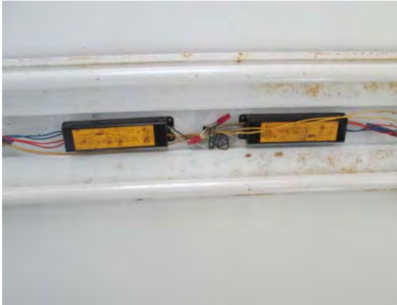
Photo 169: View of fluorescent light Ballasts (Cat./Serial No. 17A240N).
