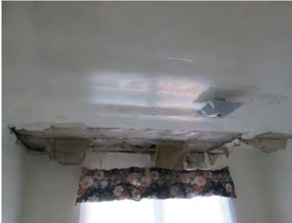
Photo 163: View of water damaged ceiling in single dwelling.
