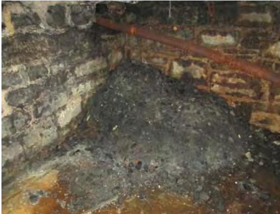
Photo 184: View of coal pile in duplex dwelling basement.
