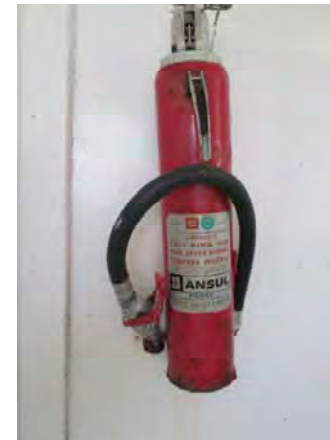
Photo 180: View of fire extinguisher in single dwelling pantry.
