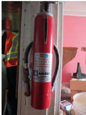
Photo 178: View of fire extinguisher in duplex dwelling hallway.
