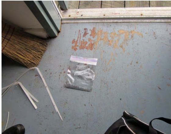
Photo 92: View of paint sample GULL-PS-48.
