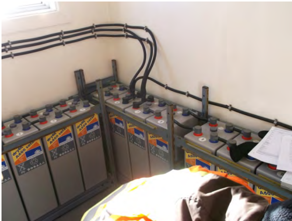
Photo 106: View of solar batteries.
