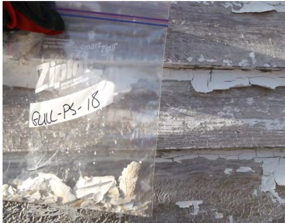
Photo 62: View of paint sample GULL-PS-18.
