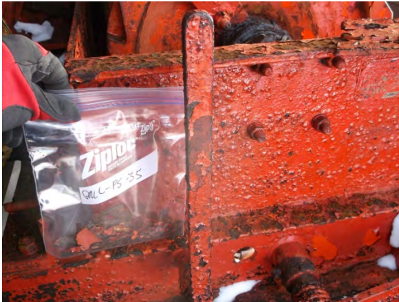
Photo 79: View of paint sample GULL-PS-35.
