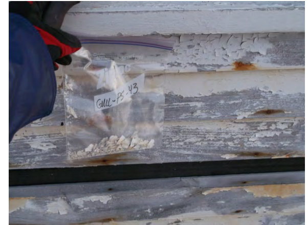
Photo 87: View of paint sample GULL-PS-43.
