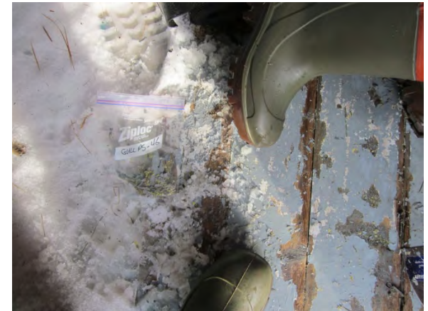
Photo 90: View of paint sample GULL-PS-46.
