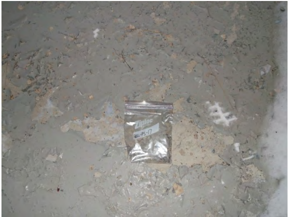
Photo 61: View of paint sample GULL-PS-17.
