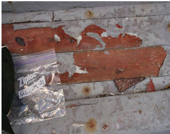
Photo 65: View of paint sample GULL-PS-21.
