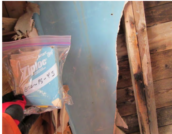
Photo 89: View of paint sample GULL-PS-45.
