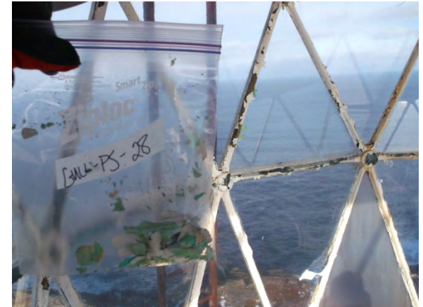
Photo 72: View of paint sample GULL-PS-28.
