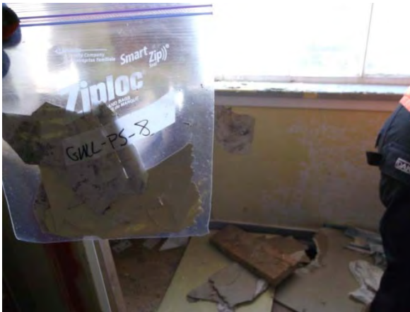
Photo 52: View of paint sample GULL-PS-8.
