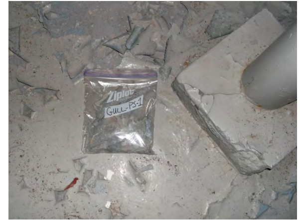
Photo 45: View of paint sample GULL-PS-1.
