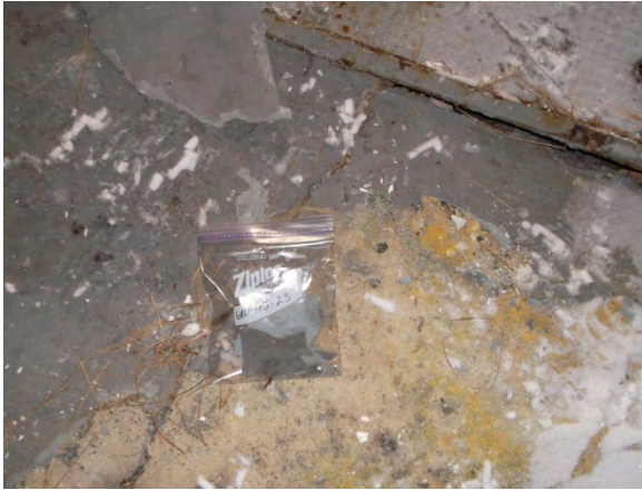
Photo 67: View of paint sample GULL-PS-23.
