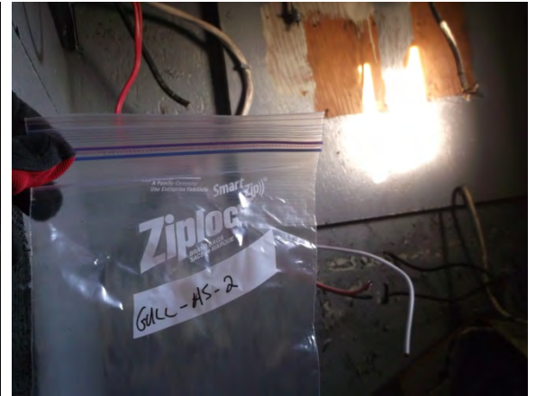
Photo 6: View of wiring insulation sample GULL-AS-2.
