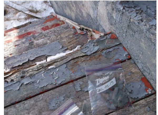
Photo 63: View of paint sample GULL-PS-19.
