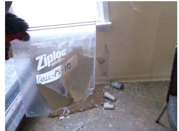
Photo 54: View of paint sample GULL-PS-10.
