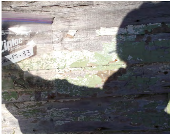
Photo 77: View of paint sample GULL-PS-33.
