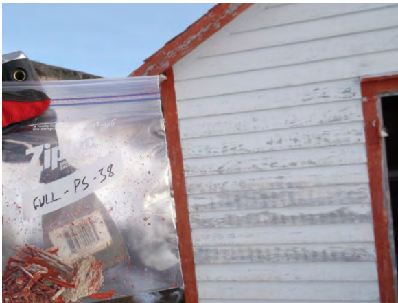
Photo 82: View of paint sample GULL-PS-38.
