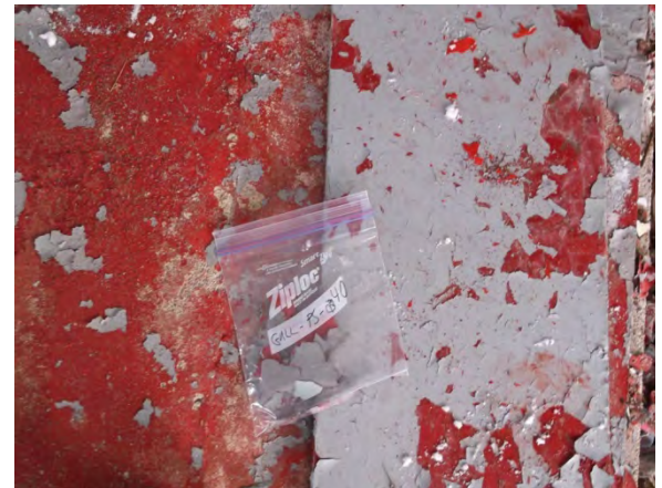
Photo 84: View of paint sample GULL-PS-40.
