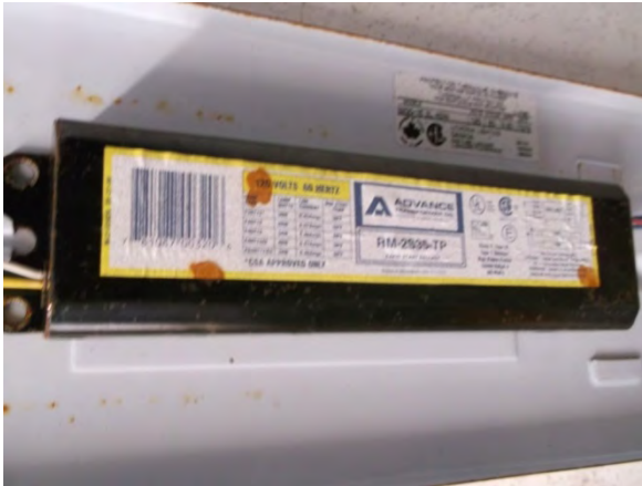
Photo 103: View of light ballast (Advance).
