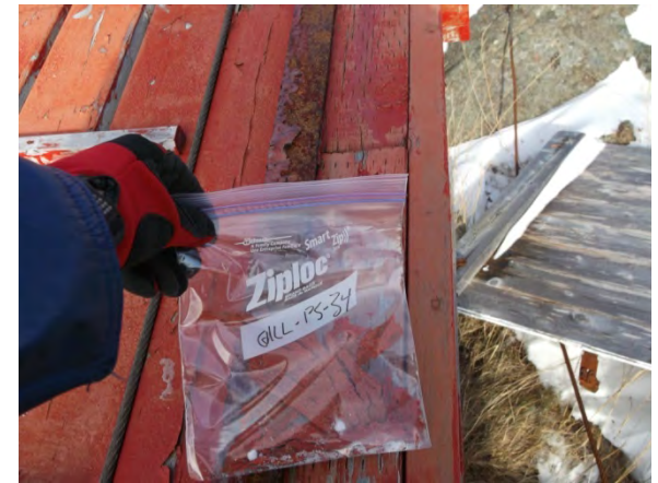
Photo 78: View of paint sample GULL-PS-34.
