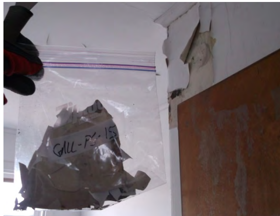
Photo 59: View of paint sample GULL-PS-15.
