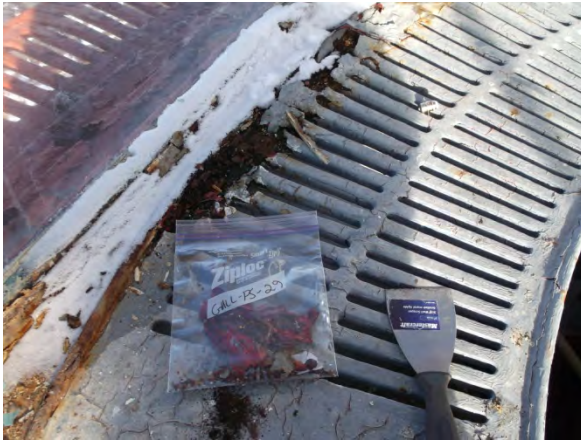
Photo 73: View of paint sample GULL-PS-29.
