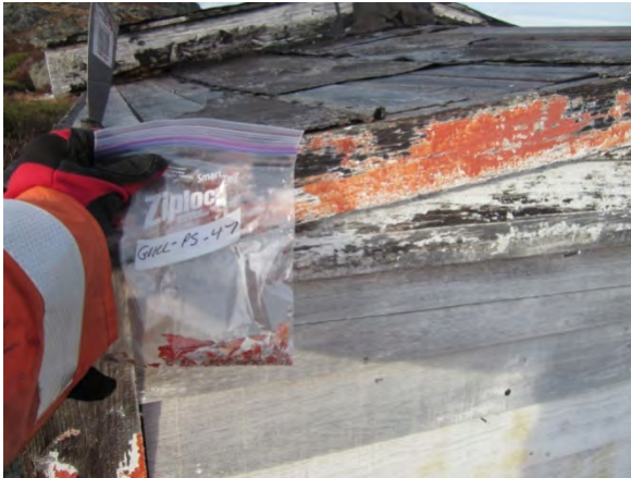
Photo 91: View of paint sample GULL-PS-47.
