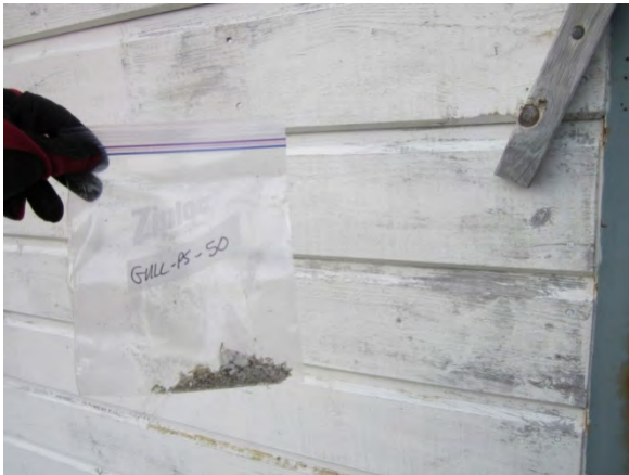
Photo 94: View of paint sample GULL-PS-50.
