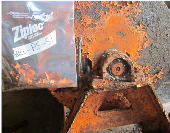
Photo 95: View of paint sample GULL-PS-51.
