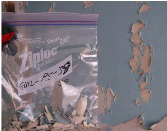
Photo 83: View of paint sample GULL-PS-39.
