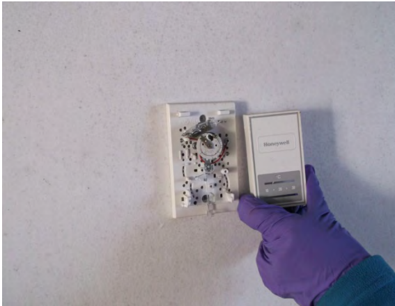
Photo 100: View of Honeywell thermostat.
