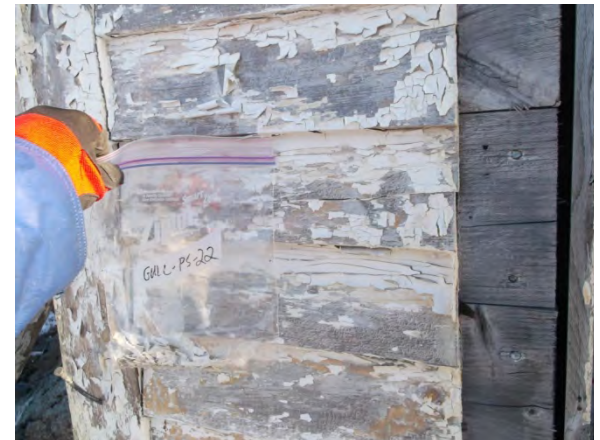
Photo 66: View of paint sample GULL-PS-22.
