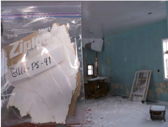
Photo 85: View of paint sample GULL-PS-41.
