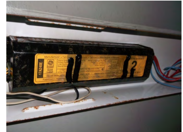
Photo 102: View of light ballast (CGE Gold Label).
