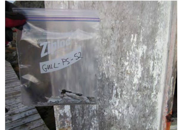
Photo 96: View of paint sample GULL-PS-52.
