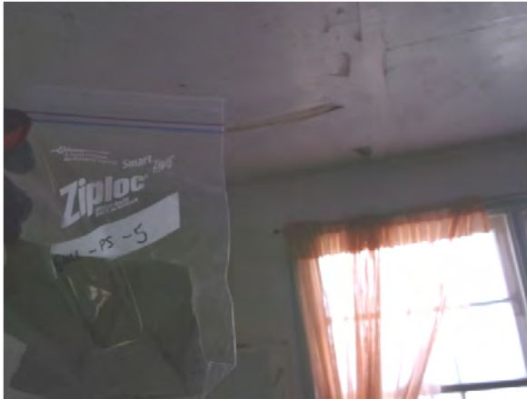
Photo 49: View of paint sample GULL-PS-5.
