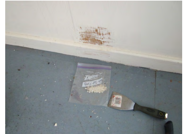
Photo 93: View of paint sample GULL-PS-49.
