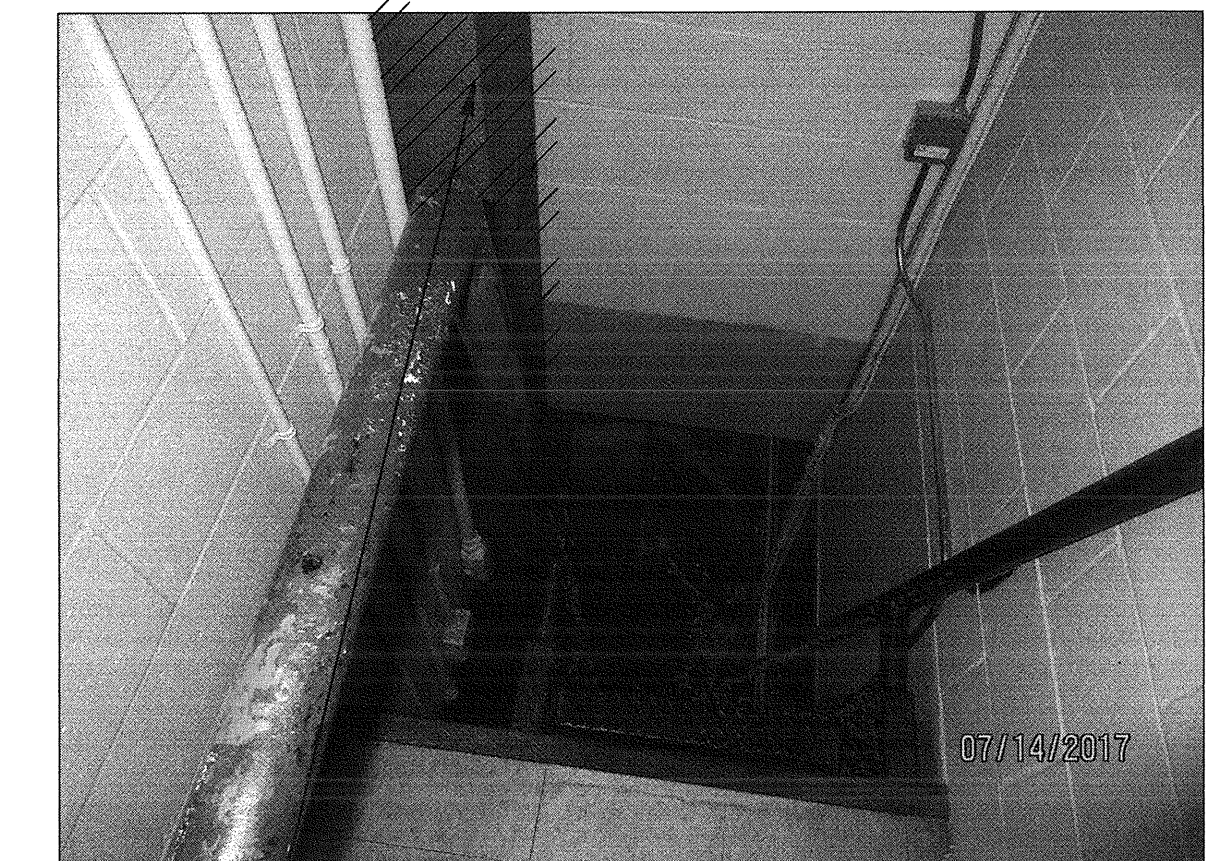
PHOTO-2 DEMOLISH DUCT RISER (FROM EQUIPMENT ROOM LEVEL TO CONTROL POST IN GROUND LEVEL.)
