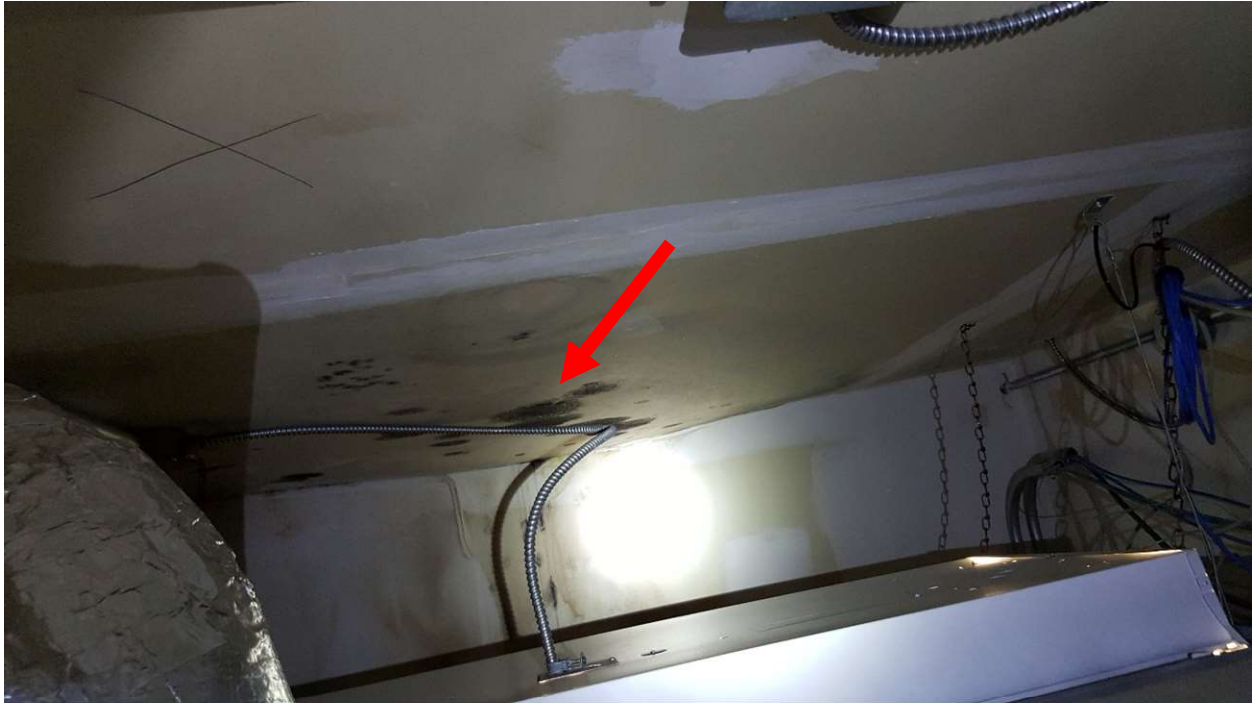
Photograph 8: Suspect mould growth above ceiling tiles of Office 108.
