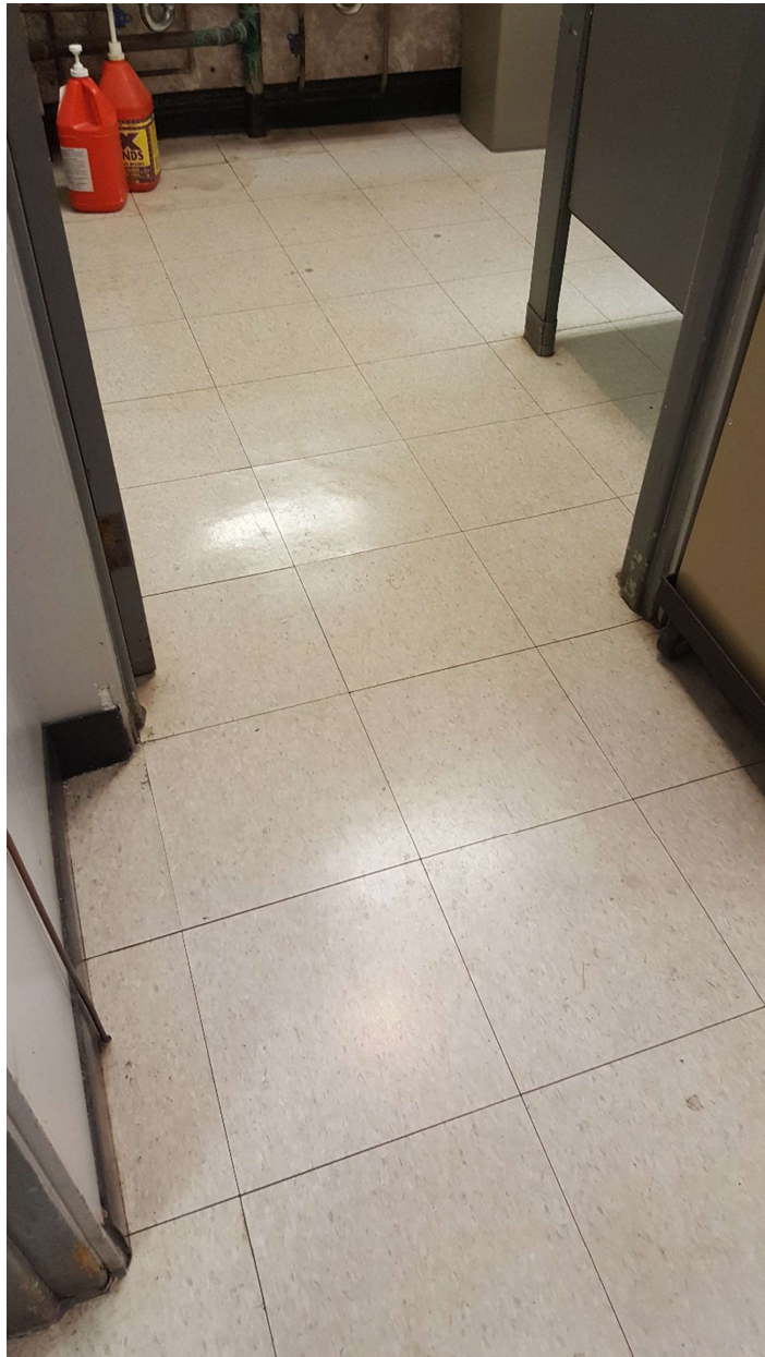
Photograph 1: Asbestos-containing black mastic associated with 12"x12" beige vinyl floor tiles, located in the men's washroom. Since the asbestos-containing mastic cannot be effectively separated from the vinyl tiles, the tiles are also considered asbestos-containing.
