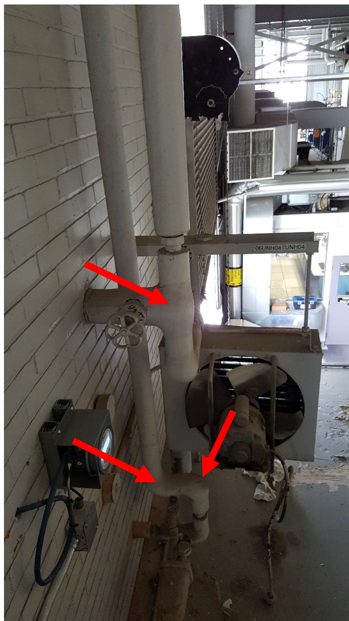
Photograph 6: Asbestos-containing grey cement compound pipe fitting insulation associated with UNH04/06UNH04 located on the roof above Office 108
