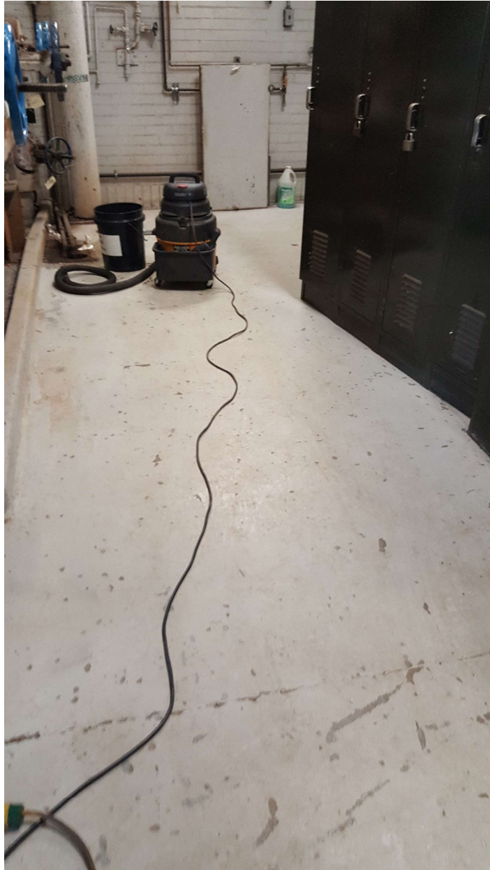
Photograph 8: Lead containing grey paint located on concrete floors throughout the project areas.
