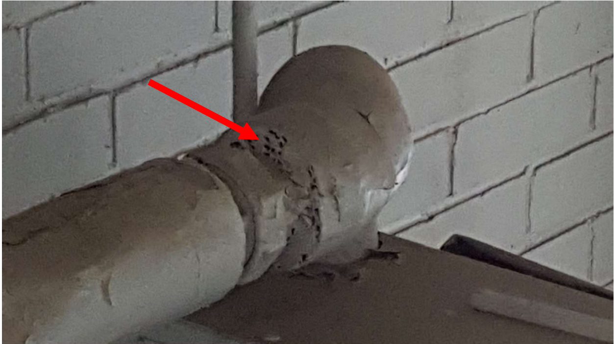
Photograph 5: Asbestos-containing cardboard pipe wrap insulation associated with UNH04/06UNH04 located on the roof above Office 108
